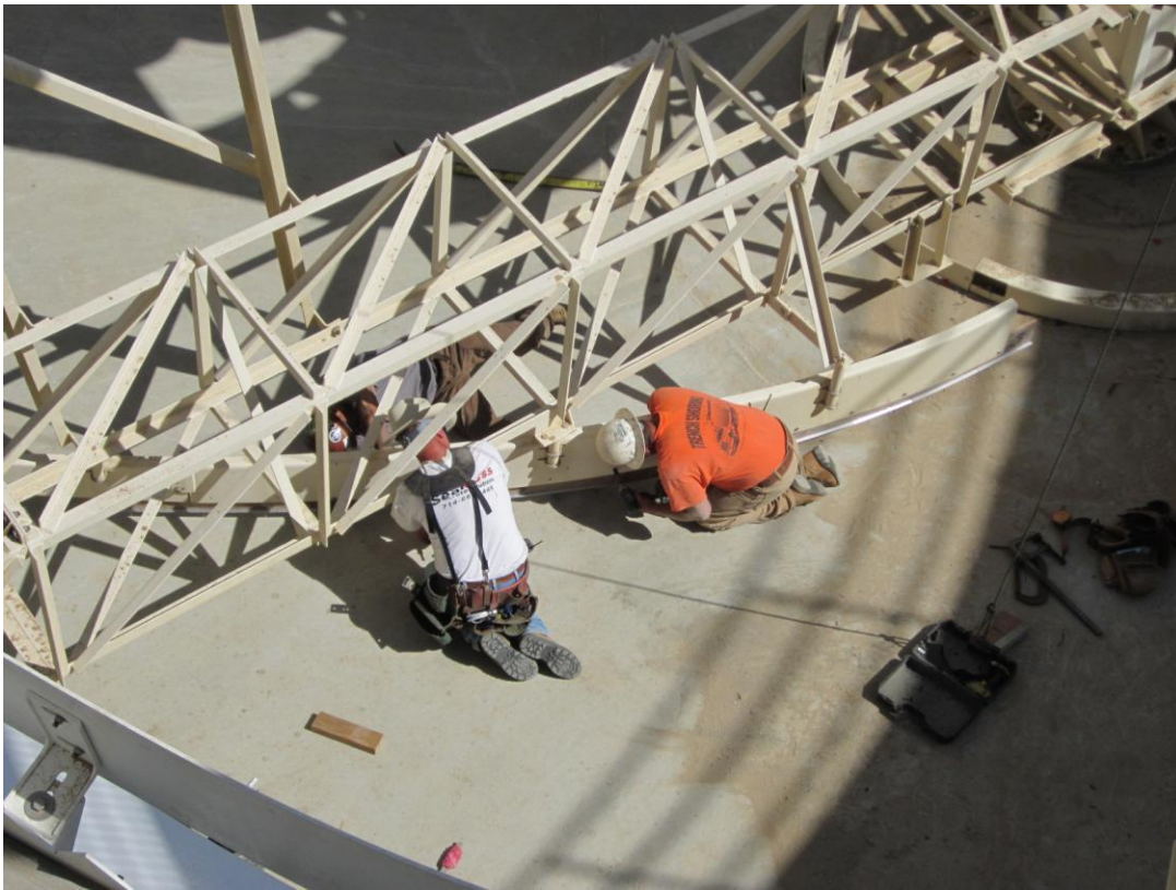
Cushman installing temporary screed to the clarifier mechanism arm for use in spreading grout.
