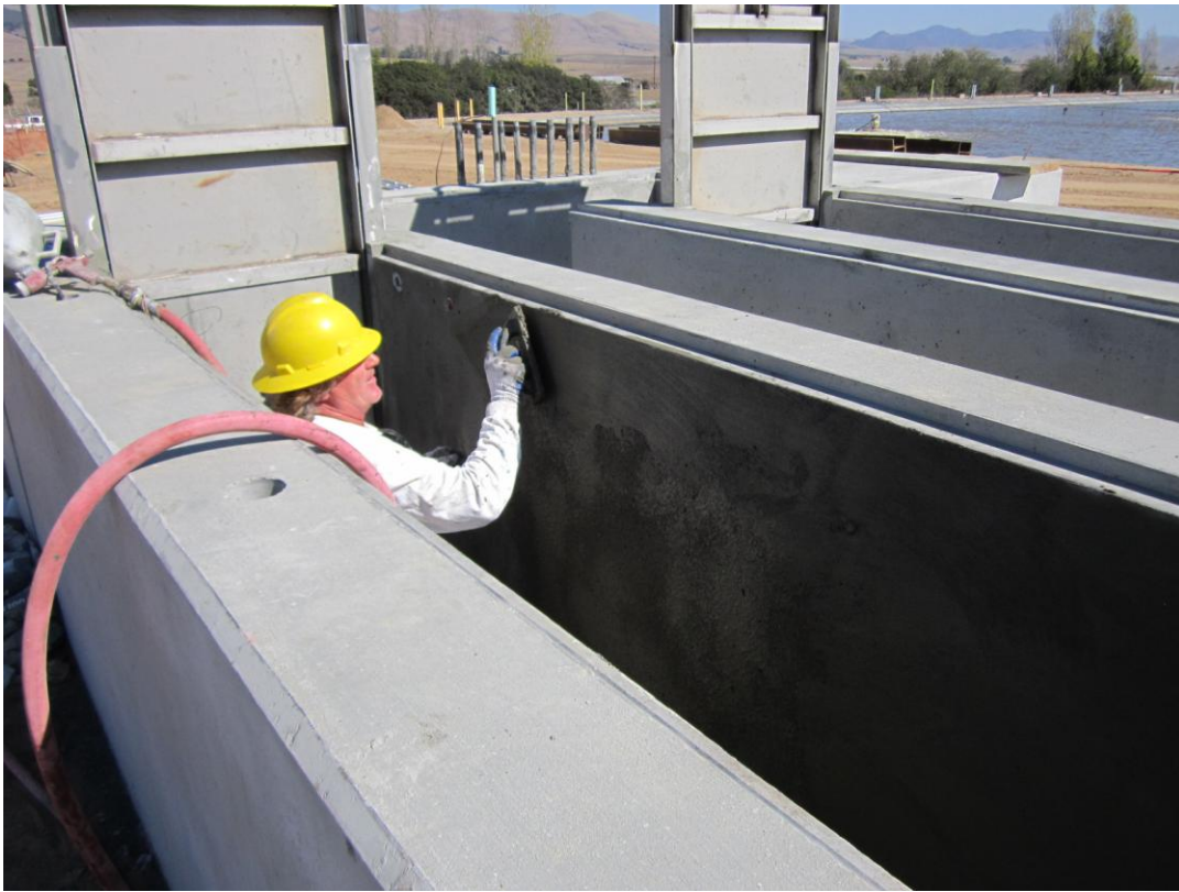
KNK Coating applying non-shrink grout to the Headworks channels in preparation for the Carboline coating.
