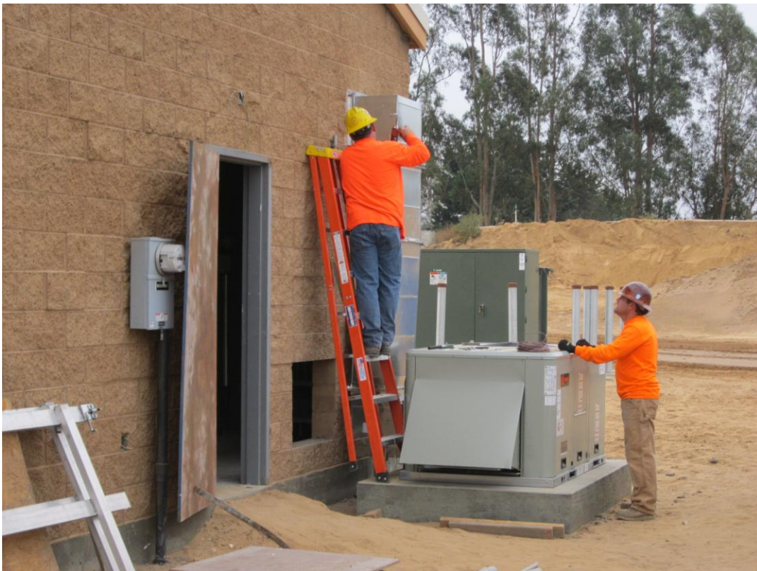
Cushman subcontractor Longs Construction installing the AC unit and ducts to the MCC room.
