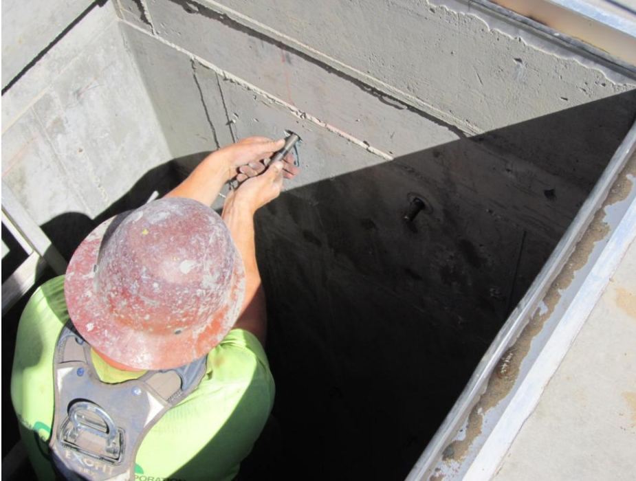
Cushman installing epoxy bolts for access ladder inside the Influent Pump Station.
