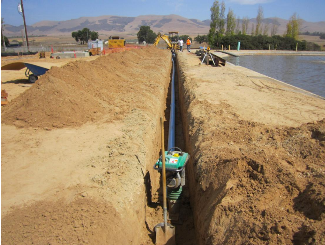
Cushman installing 6-inch NPW line from Influent Pump Station toward Sludge Thickening Building.
