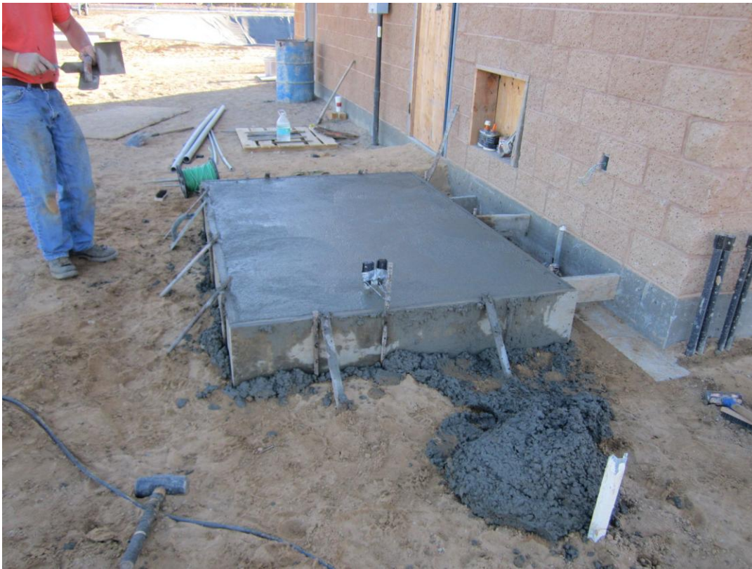
Cushman finishing the concrete slab for the air conditioning unit to the MCC room.
