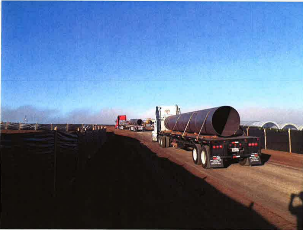
Casing (54-inch diameter) arriving on the north side at the future pump station site.
