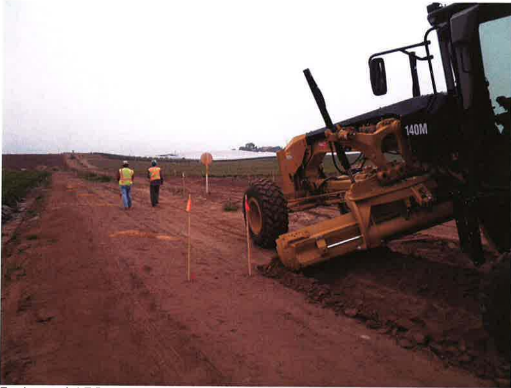
Burke and ARB creating a 12" deep ditch to key in the silt fence on the north side to prevent migration of California Red Legged Frogs onto the site.
