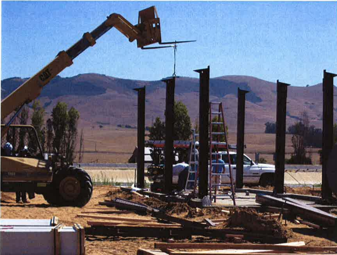
Dueck Construction erecting steel structure at Sludge Thickening System to support canopy.
