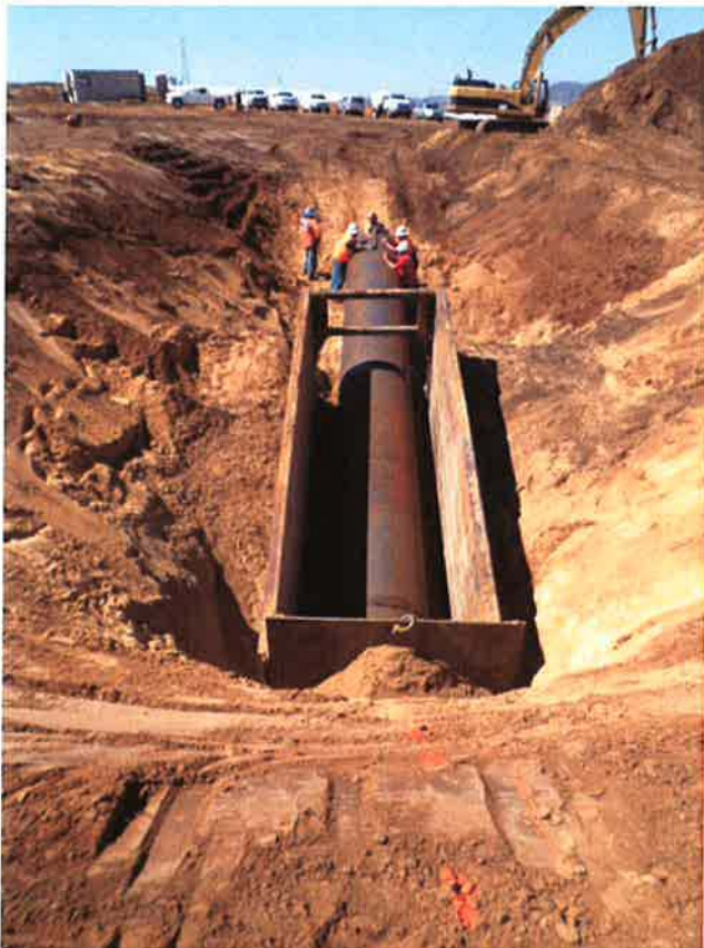
ARB installing the 54-inch diameter casing on the north side of the project.
