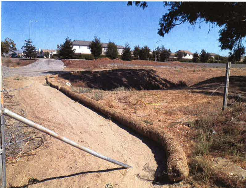
Straw waddles installed for SWPPP around the SBCFC drainage channel near the temporary access road constructed on the south side of the levee.
