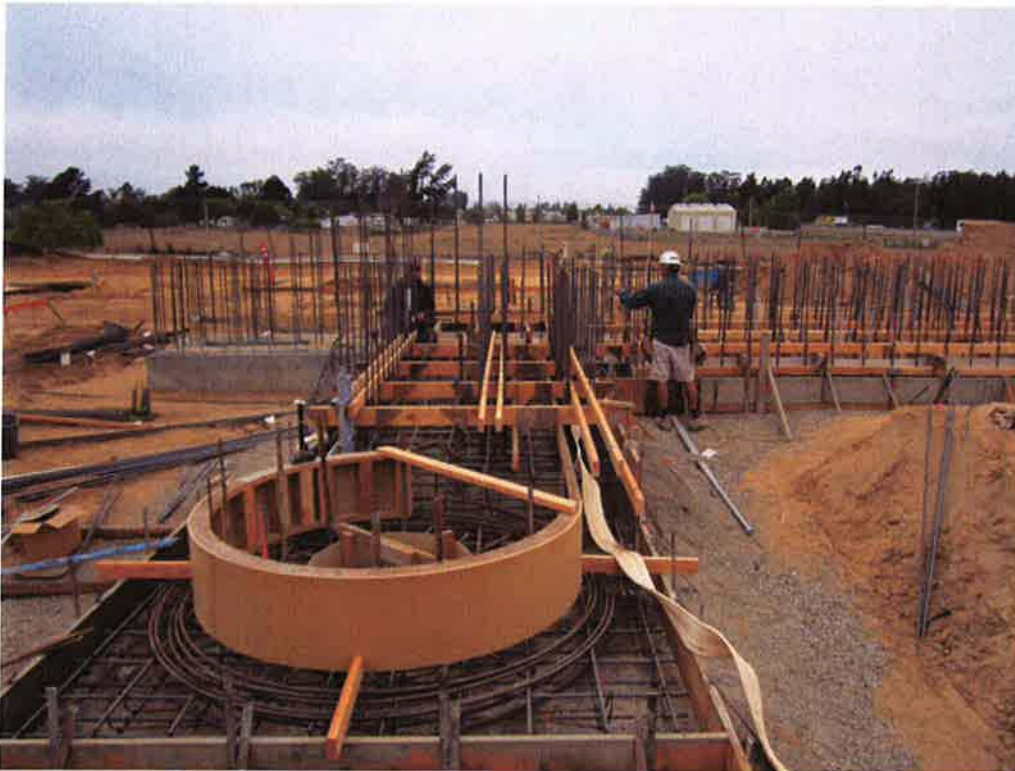
Cushman forming the slab and grit vortex of the Grit Removal System.
