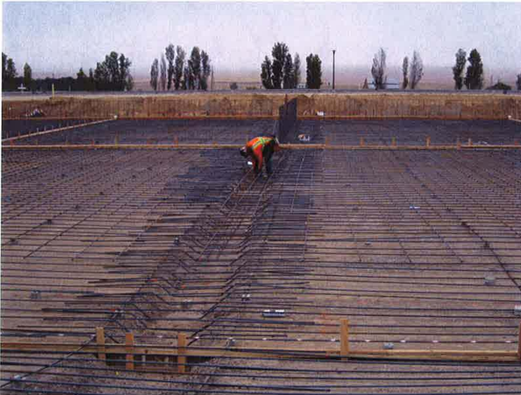
CMC Rebar tying reinforcement at the wall foundations of the Sludge Drying Beds.
