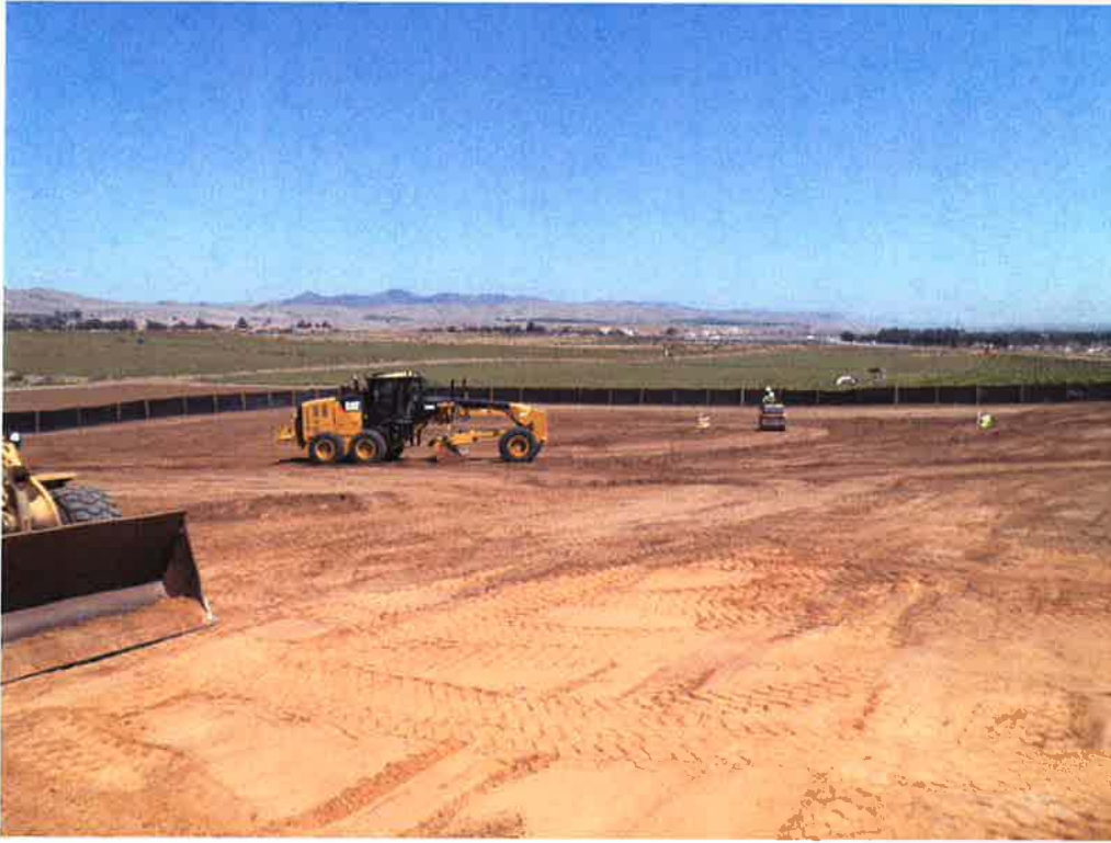
North side of the site at future pump station prepped for installation of the 54-inch diameter casing.
