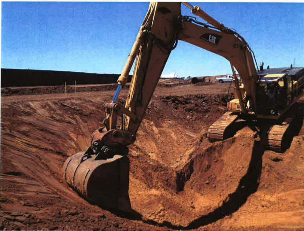
Excavation for the 54-inch diameter casing at the north side of the project.
