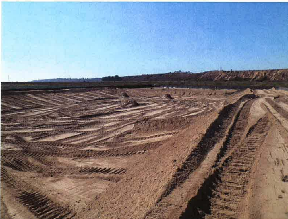
Excavation and preservation of top soil on the south side within the temporary construction easements.
