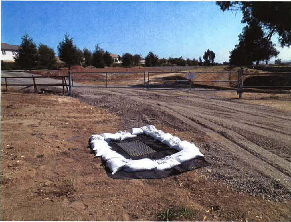
New 12' gate in SBCFC fence (for total width of 24'), and SWPPP installed at catch basin on the south side of the levee along the temporary access road constructed by ARB.
