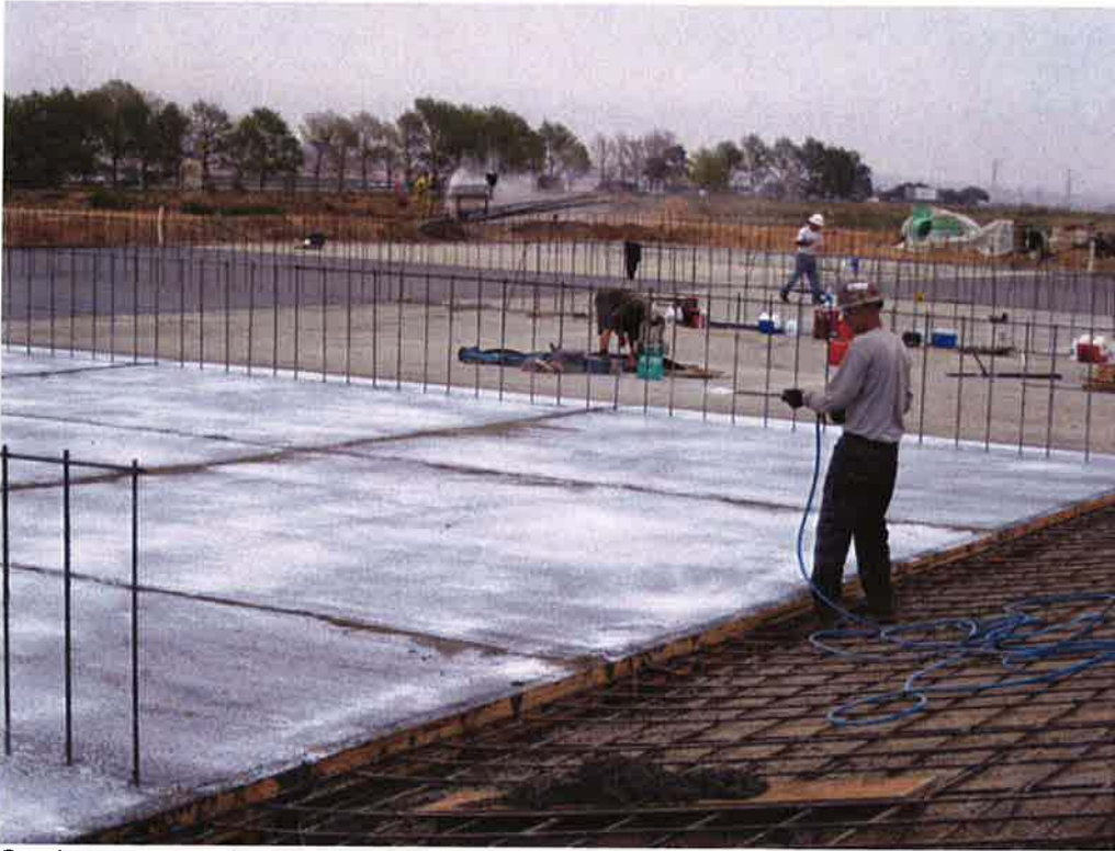
Cushman spraying curing compound on last slab section of Sludge Drying Bed #2 after last concrete pour.
