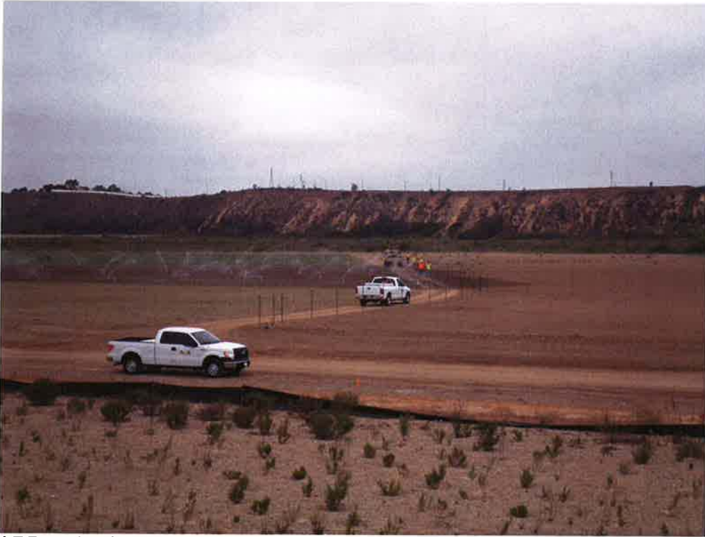
ARB and subcontractor Marborg installing silt fence along temporary construction easements at the south site.
