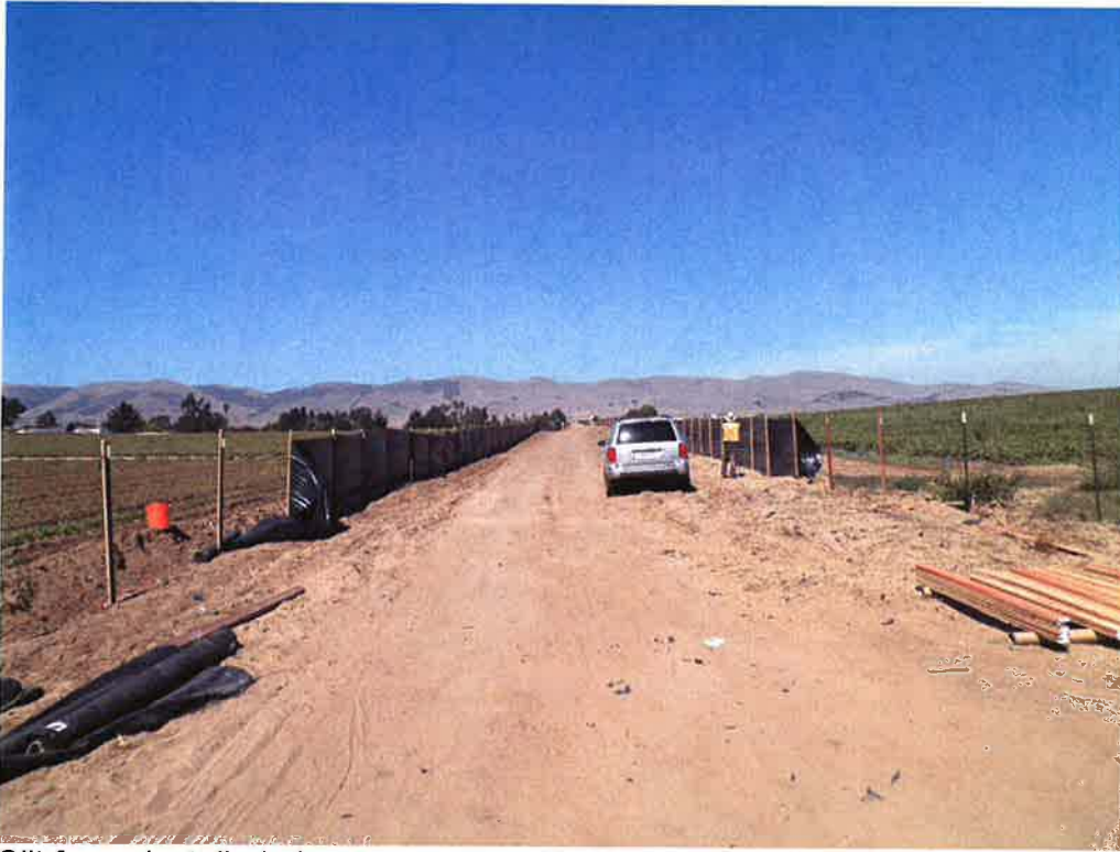
Silt fence installed along access road to the pump station site. Rincon on site to provide monitoring for CRLF's.
