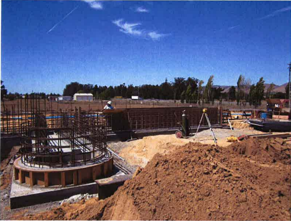
Forming walls of the grit vortex and the interior walls of the Headworks Screening System.
