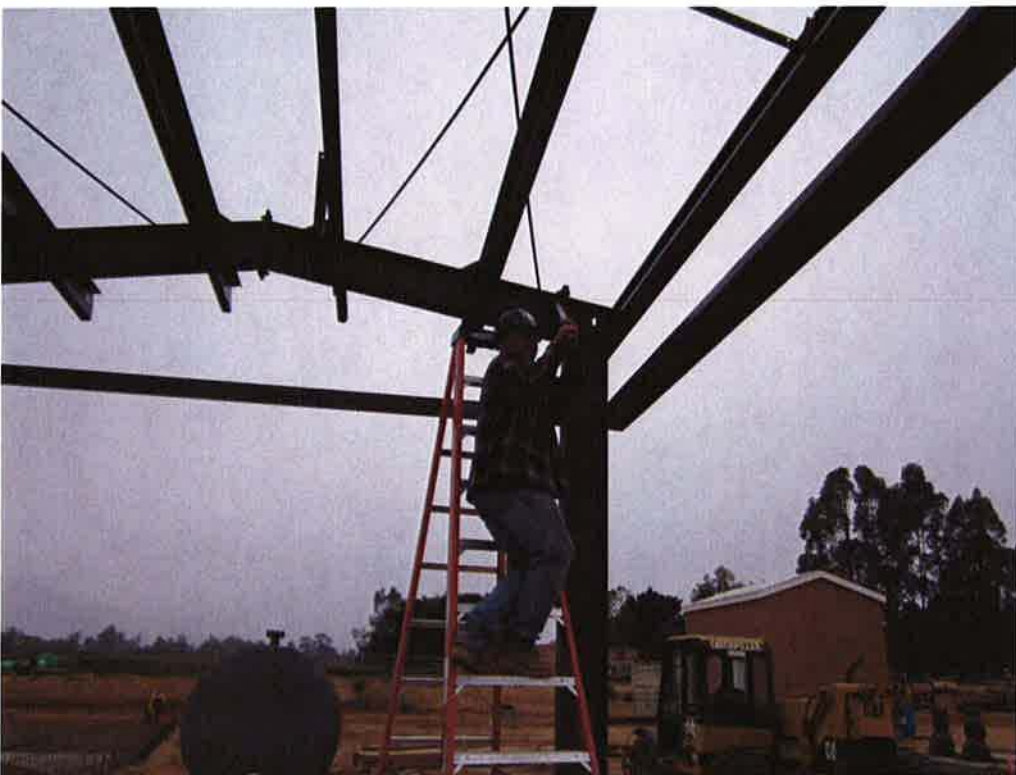
Fugro torque testing the bolts on the structural steel for the canopy.
