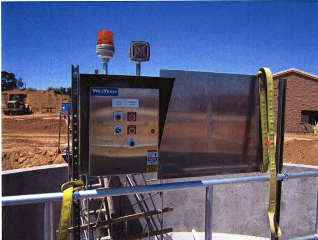
Clarifier mechanism local control panel mounted on bridge at Clarifier #2.
