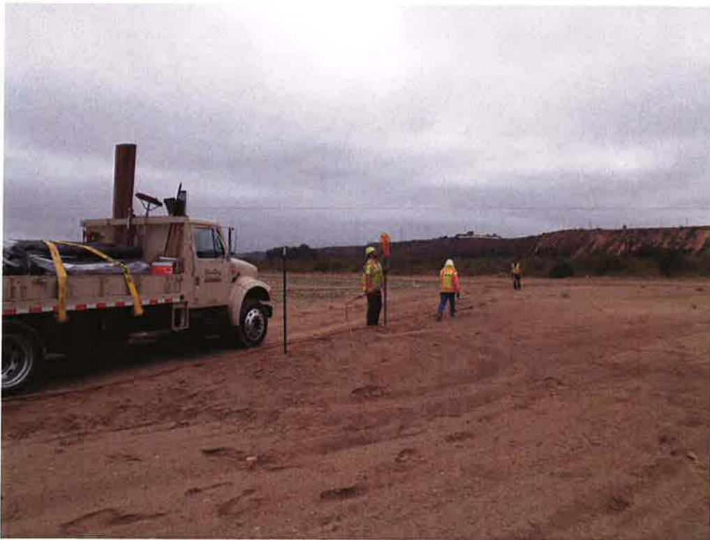
Marborg installing fence posts for 6' silt fence on south side of project.
