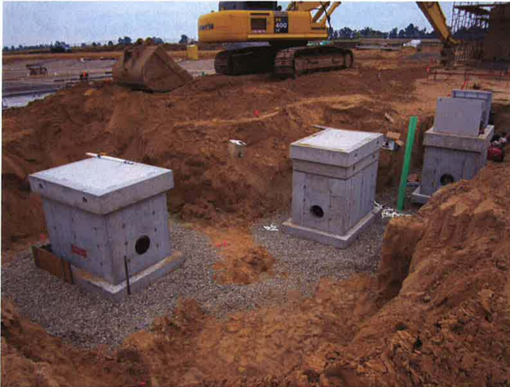
Flow meter vaults installed.
