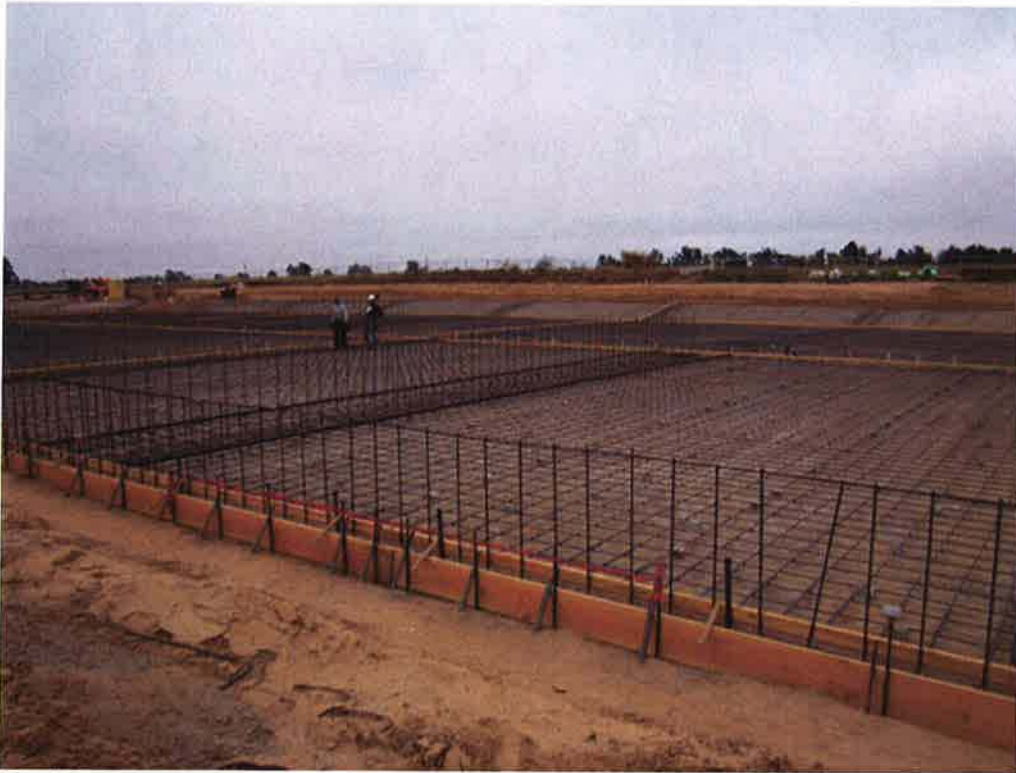
Cushman setting screed guide rails at Drying Bed #1 in preparation for first concrete pour.
