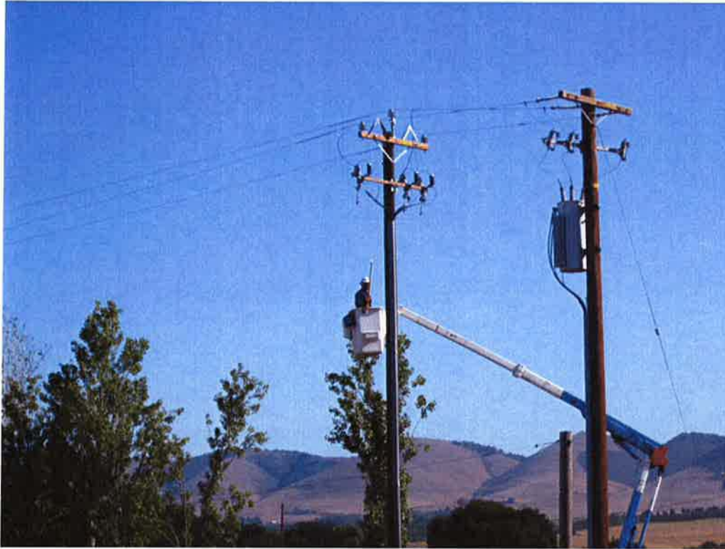
PG&E energizing the new service on August 15, 2013.
