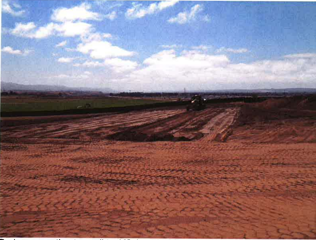
Burke excavating top soil to 18" deep inside pump station temporary construction easement and HDD work area.
