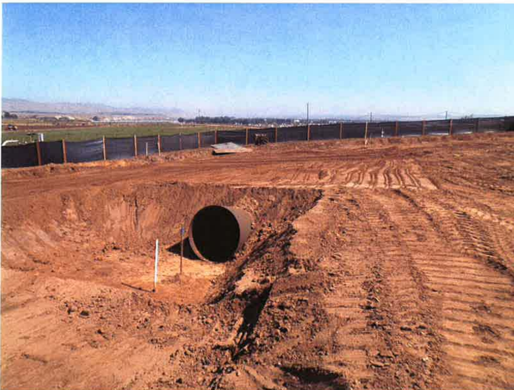
Completed installation of 54-inch diameter casing on north side of the project.
