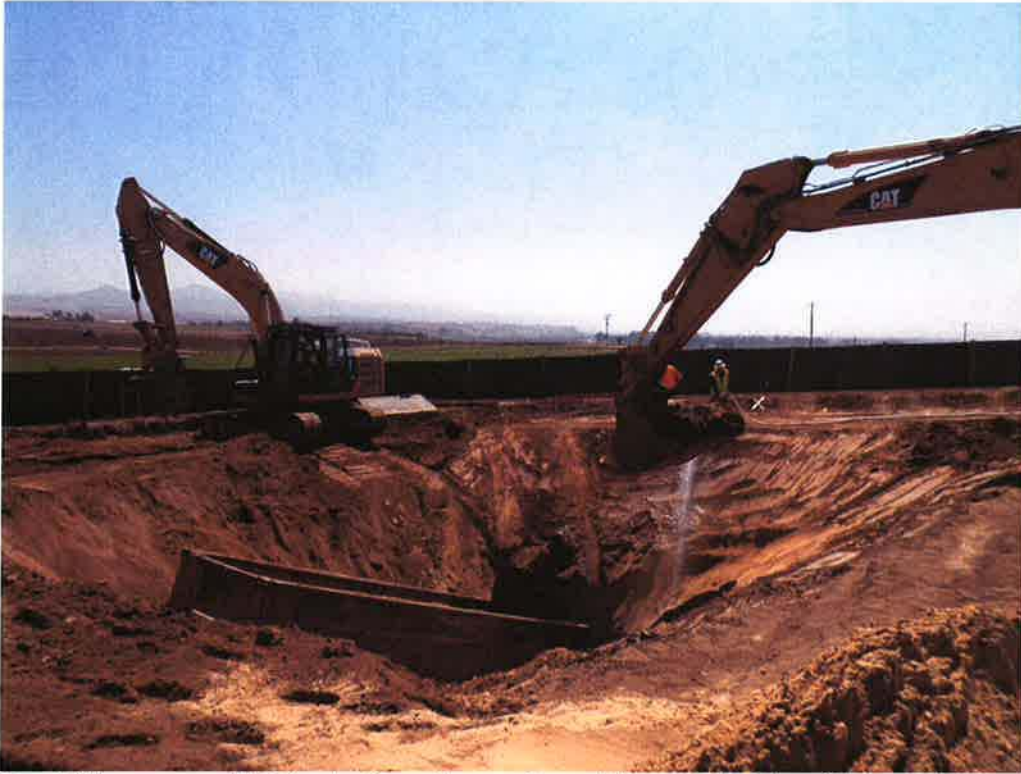
Backfilling around 54-inch diameter casing at the north side of the project.
