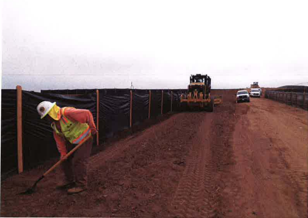
Burke using grader and ARB working by hand to key in the bottom of the silt fence along the access road to prevent CRLF's from migrating onto the site during construction.
