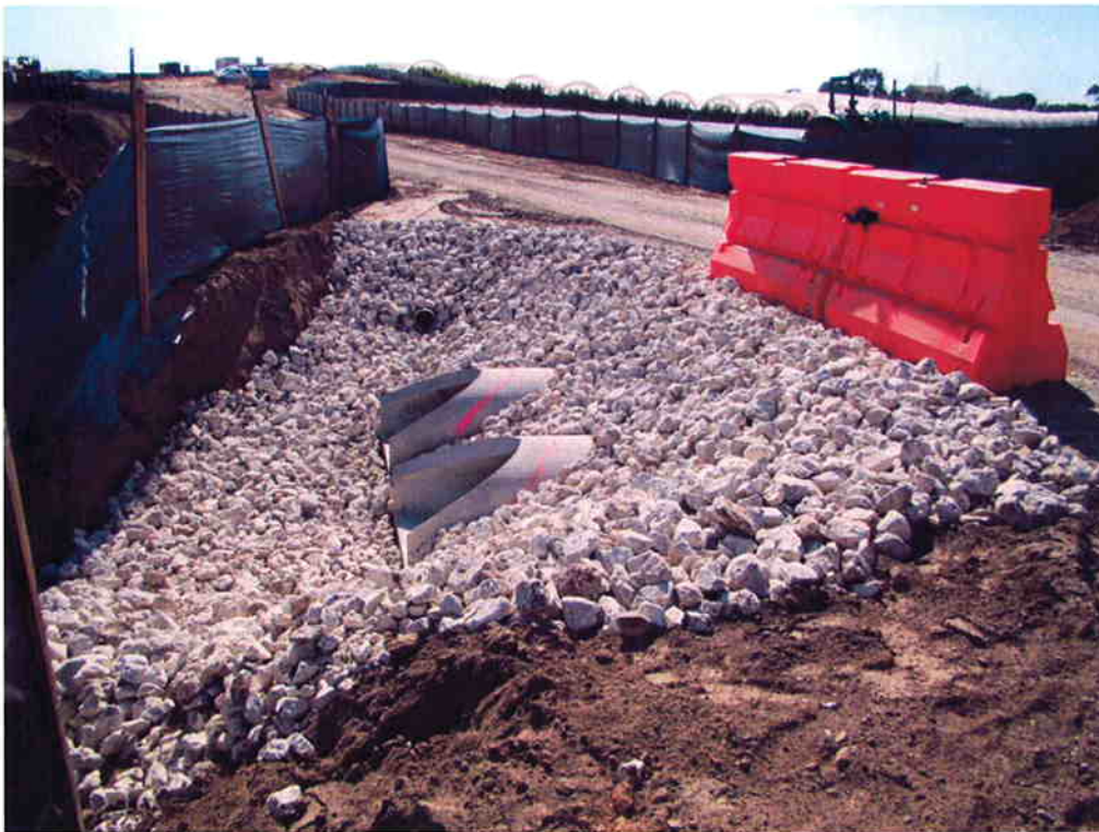
Rock rip-rap placed at both flared ends of the 18-inch RCPs to control erosion.
