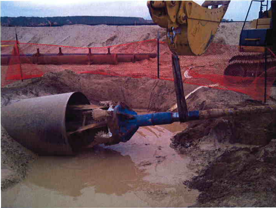
36-inch drill entering 54-inch casing to start next reaming pass from south to north.
