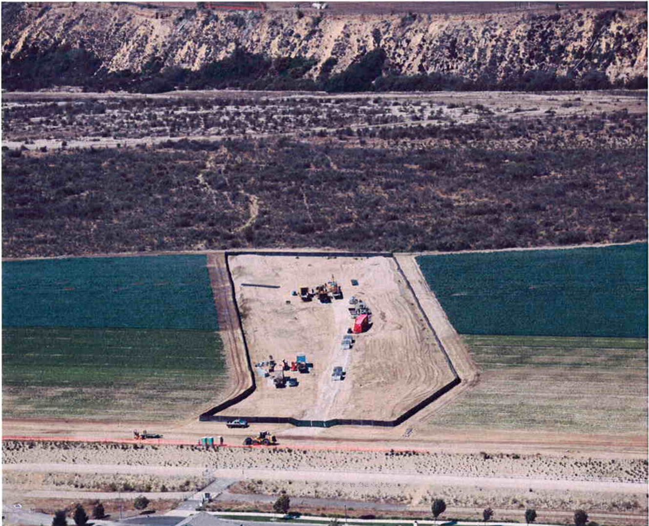
Aerial photo of the south side with ARB drill rig and equipment mobilized.
