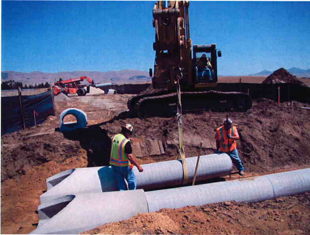
ARB installing the 18-inch RCPs with flared ends over the steel casing.
