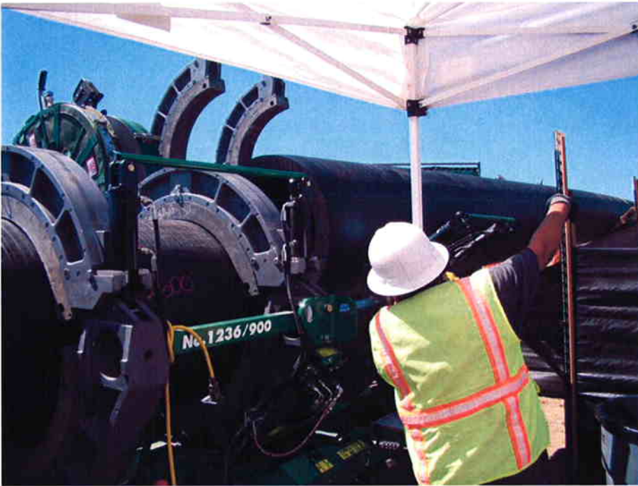
ARB fusion welding operator directing placement of the next section of pipe for welding.
