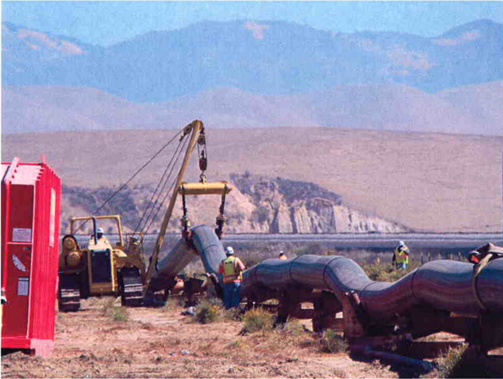
Machine used to pull pipe along rollers when a weld is completed.
