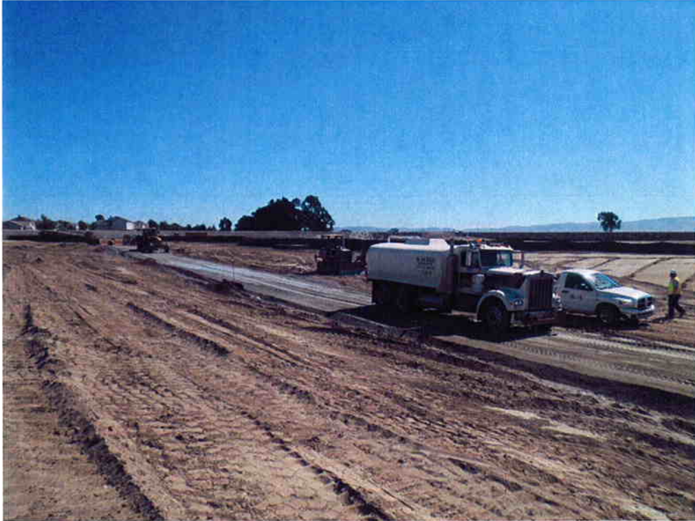
ARB building access road into south site due to soft, uncompacting native soils.
