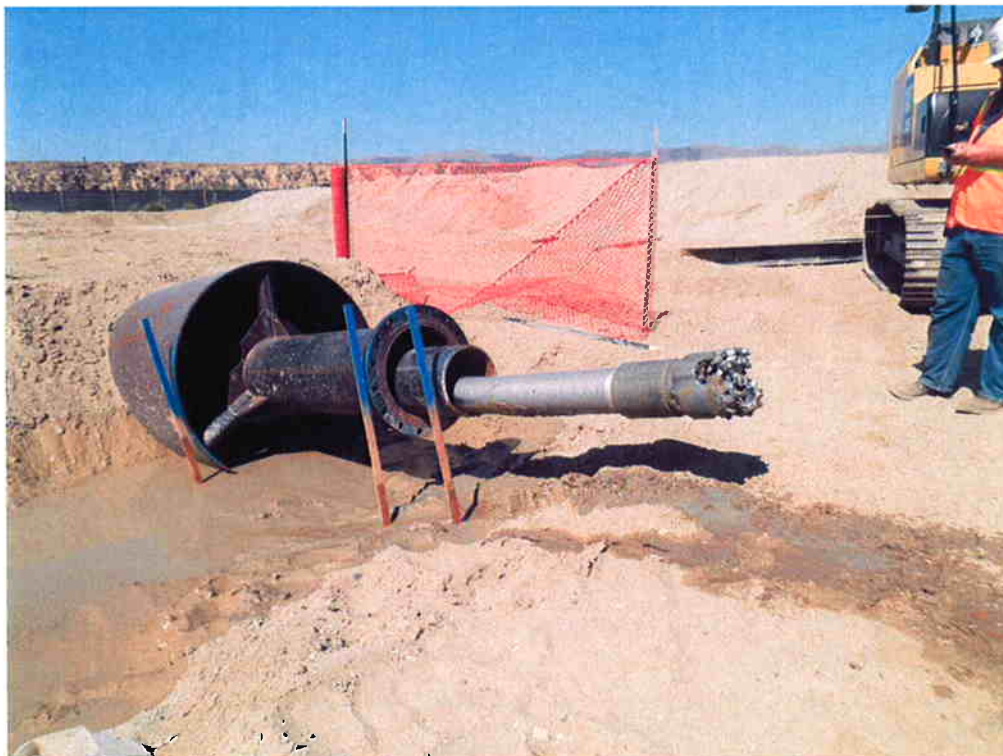
12-inch drill emerging from casing on south site, after drilling from the south site was terminated and started again for a successful completion from the north site to the south site.
