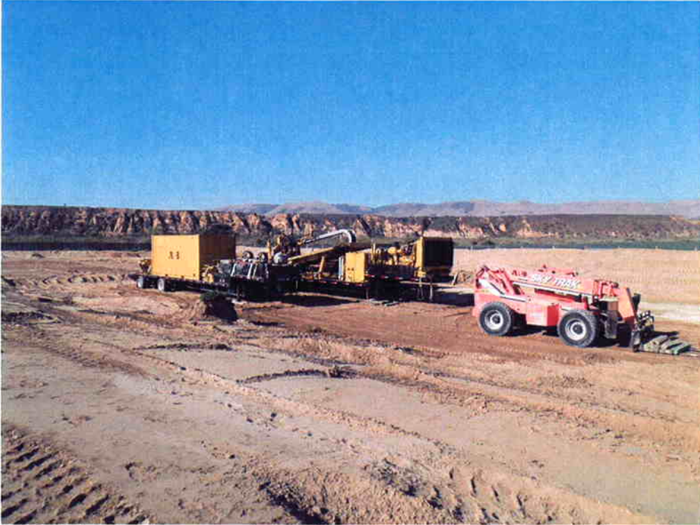
ARB drill rig and equipment mobilized to south site and ARB starting set-up.
