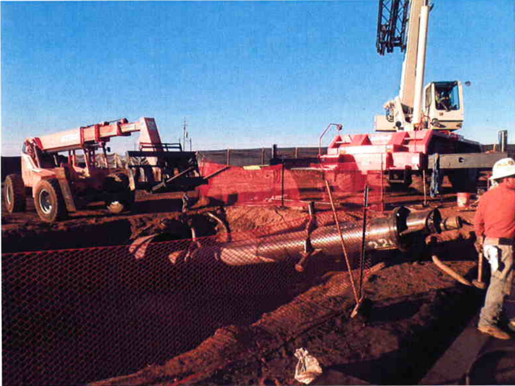
ARB removing centralizer from 54-inch casing to allow the 26-inch drill to come out of the casing.
