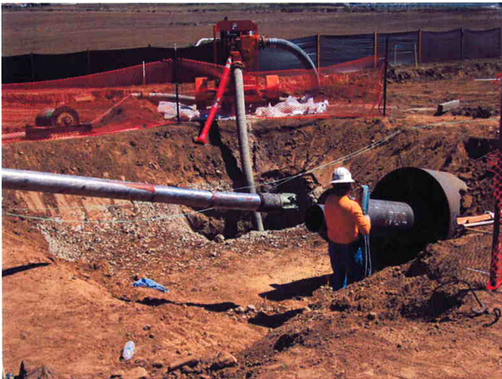
Starting pilot hole drill from the north site after demobilizing from the south site.
