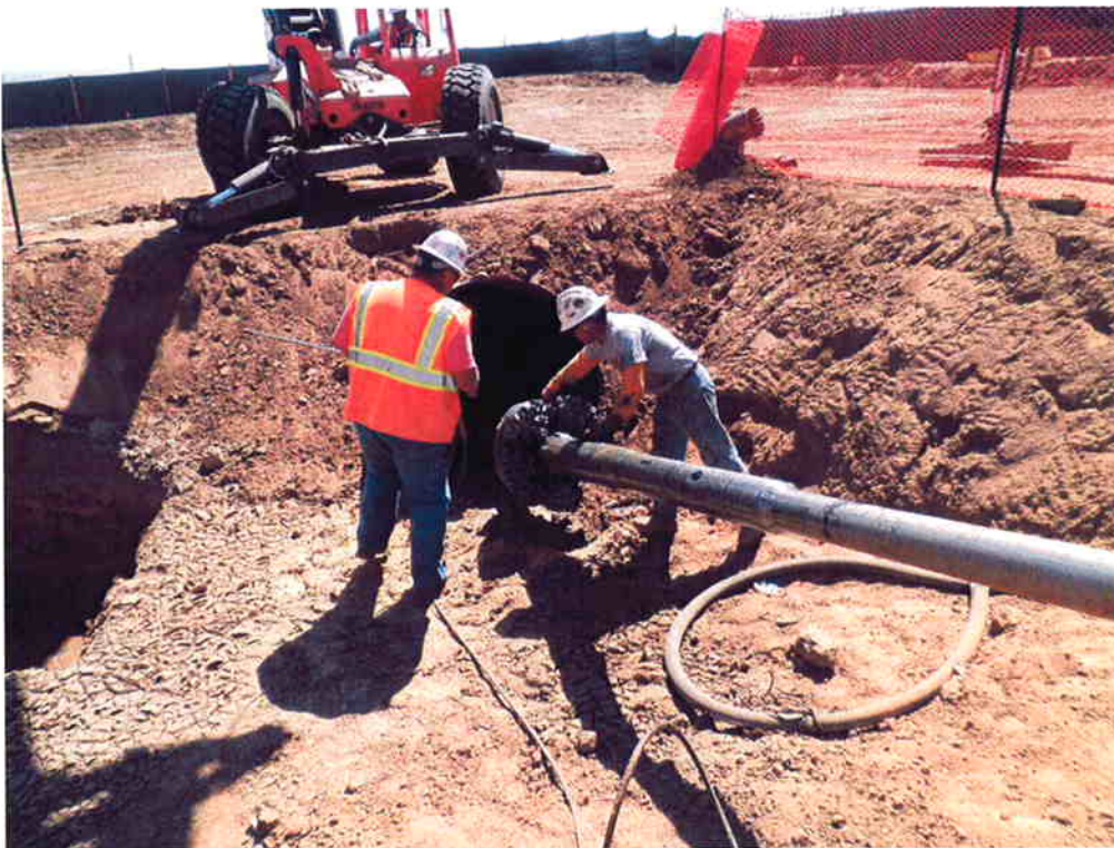
The 26-inch drill emerging from the 54-inch casing completing the 26-inch ream.
