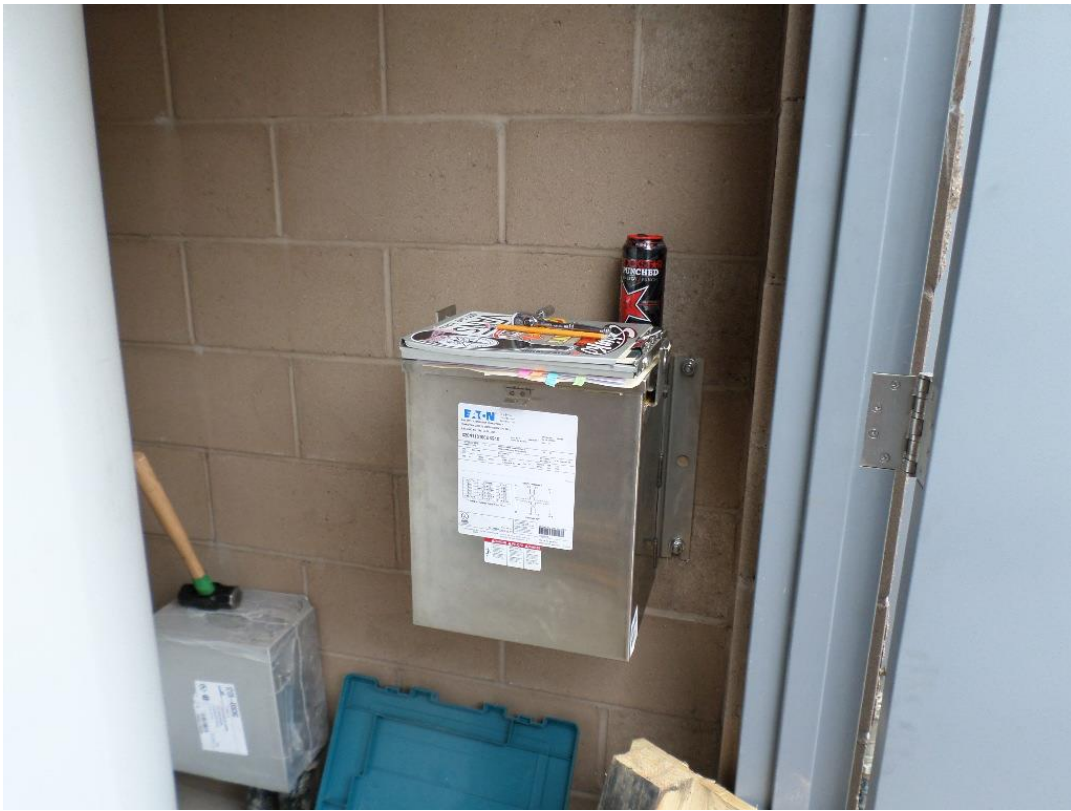
Transformer installed by St. Denis Electric.
