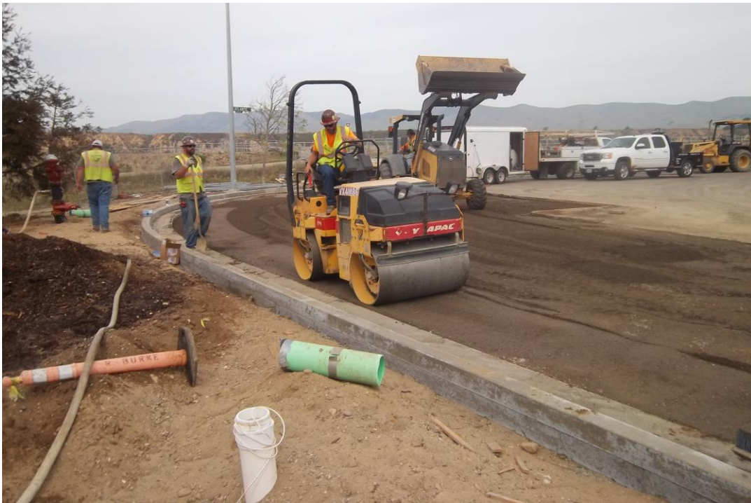
D-KAL compacting aggregate base at Blosser and Atlantic in preparation for final paving.
