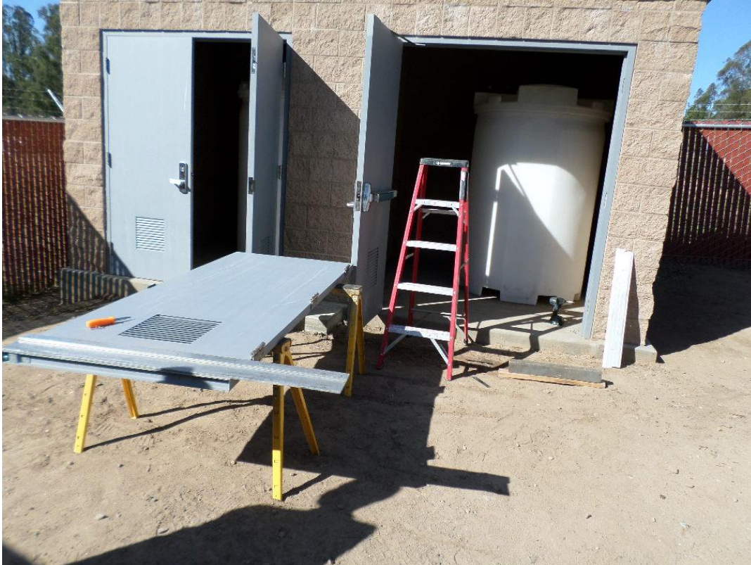
Doors being trimmed by manufacturer to make final fit with door frame.
