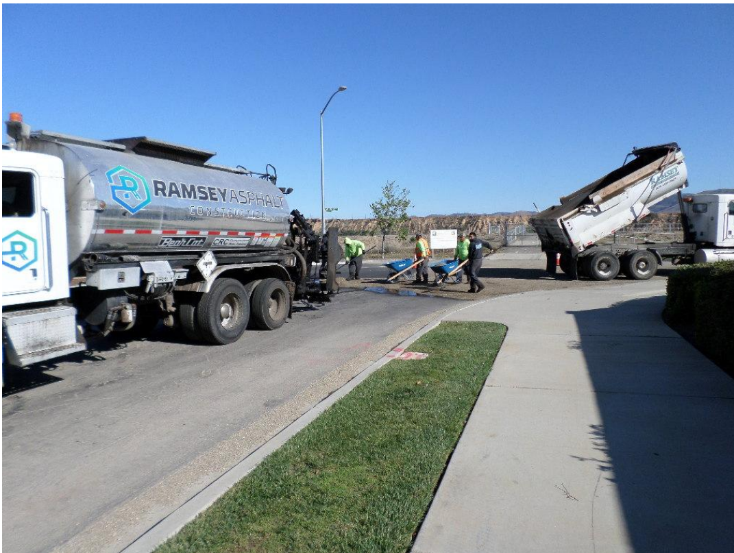
Ramsey Asphalt placing slurry seal at Blosser and Atlantic per the request of the City of Santa Maria.
