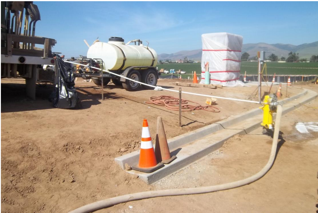
D-KAL using a “water buffalo” to inject chlorine into the pipeline at BP #4 and flush to the end at Taylor and Blosser to achieve 6 ppm throughout the line.
