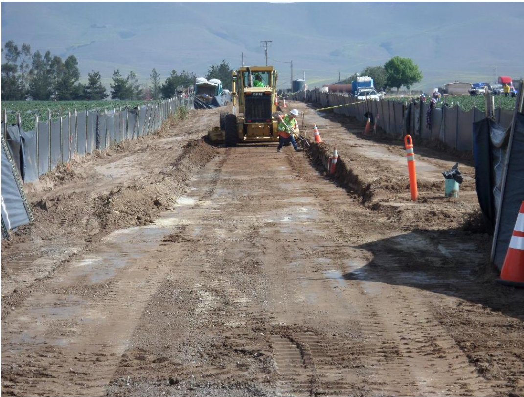
Spieß cutting the access road to subgrade to build permanent access road.
