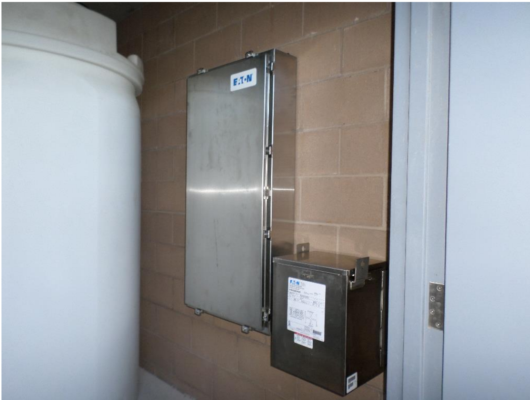
Electrical panel and transformer installed by St. Denis Electric.
