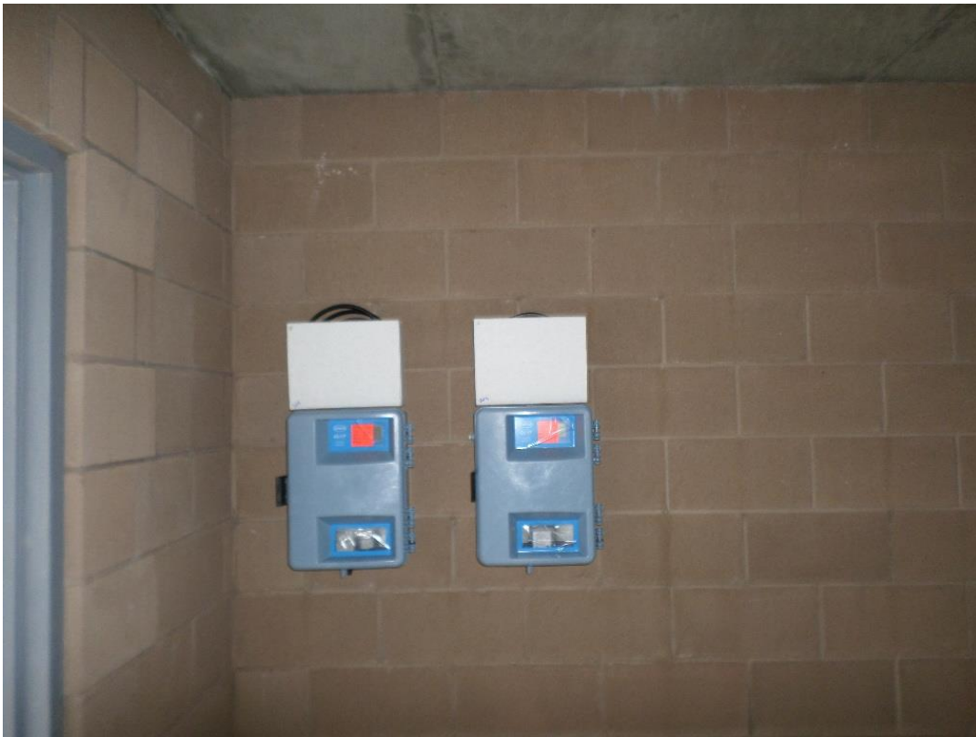
Chlorine analyzers installed by St. Denis Electric.
