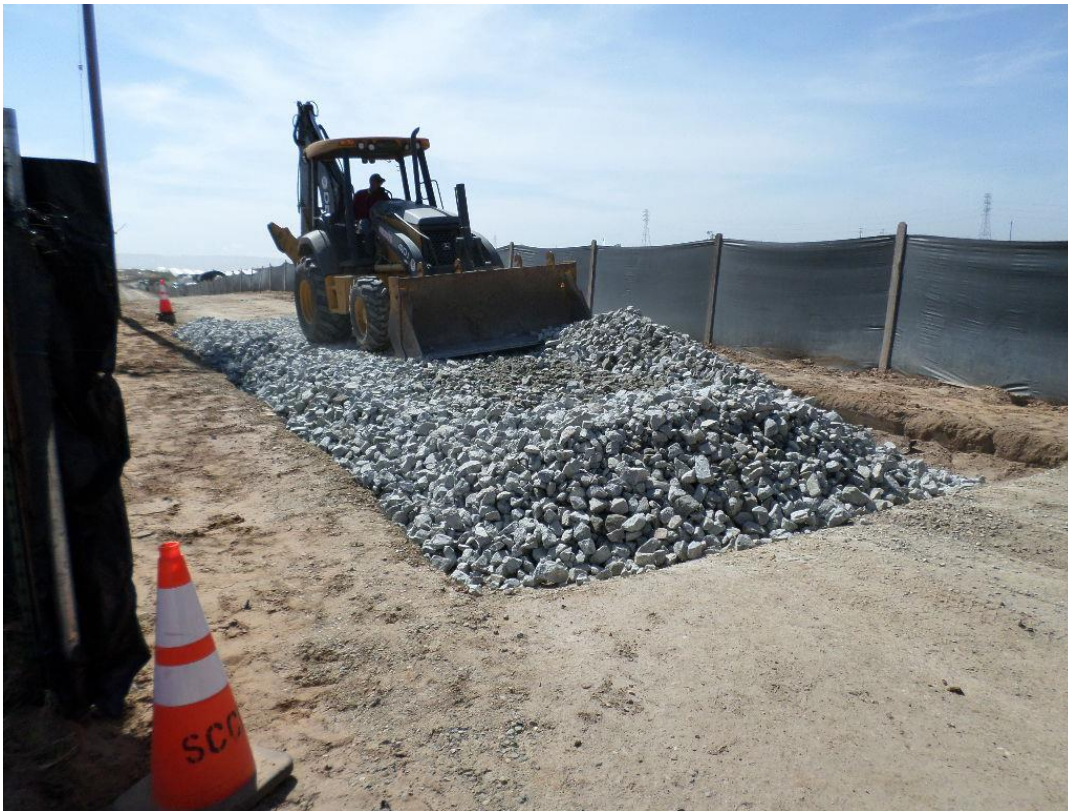
Spieß installing tracking control at the beginning of the permanent access road.
