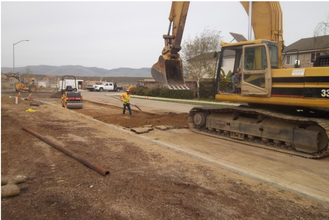
D-KAL removing sawcut pavement along trench edges in preparation for final paving at Blosser and Atlantic.
