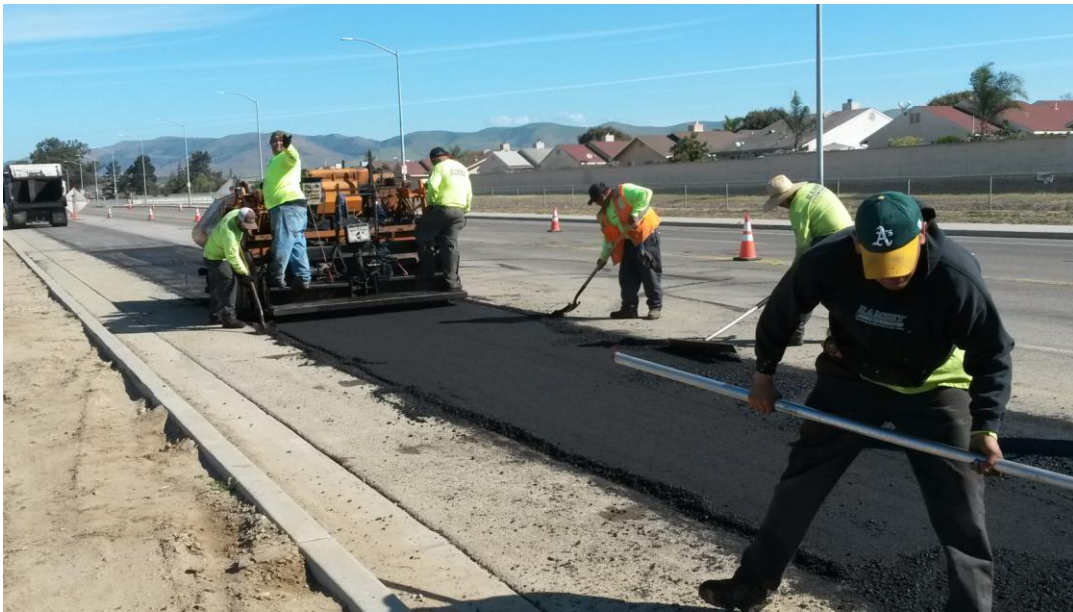
Ramsey Asphalt completing final paving at end of the pipe in Blosser at Taylor.
