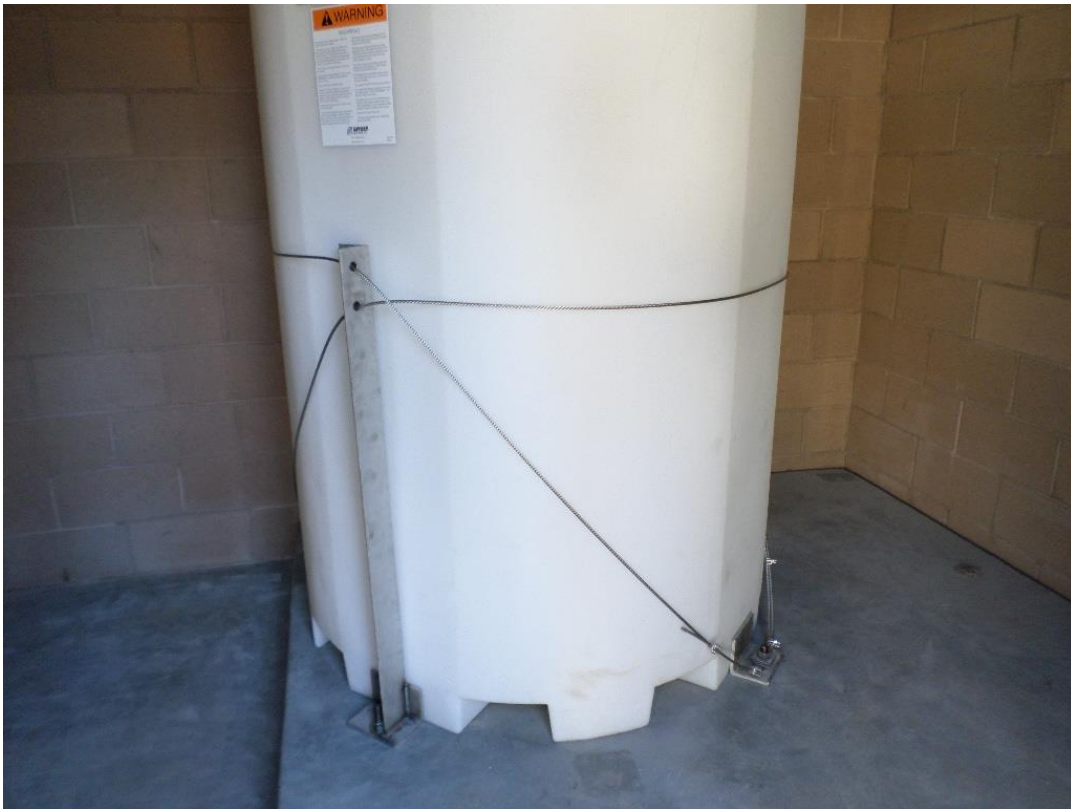
Chemical tank installed with tie-downs.
