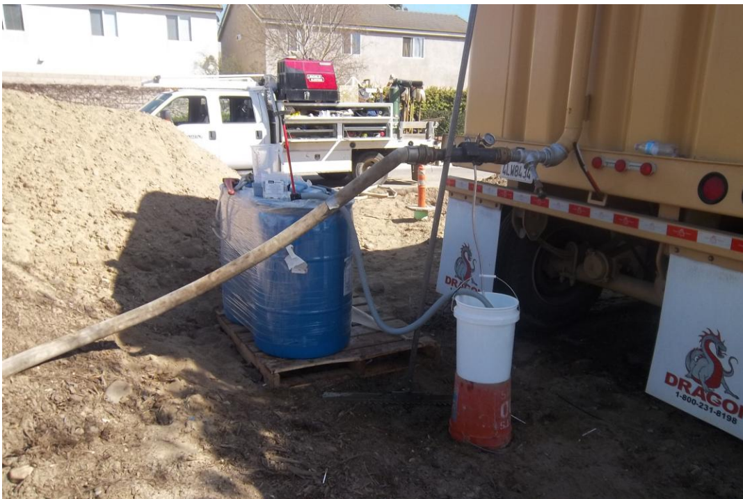
Dechlorination process at Baker tank.
