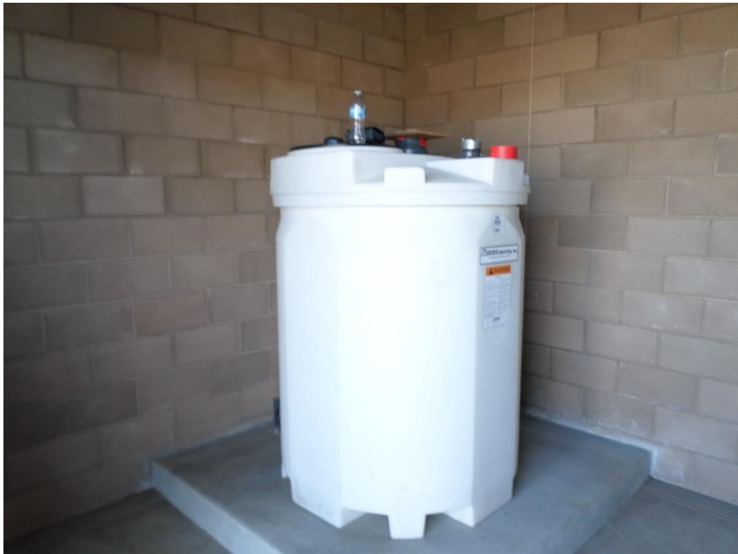
Chemical tank installed at pump station.
