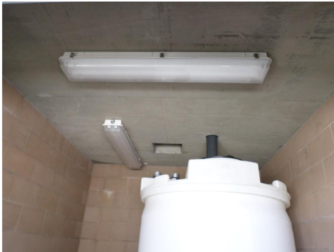
Lights installed by St. Denis Electric inside chemical building, chemical tank installed by Spiess.
