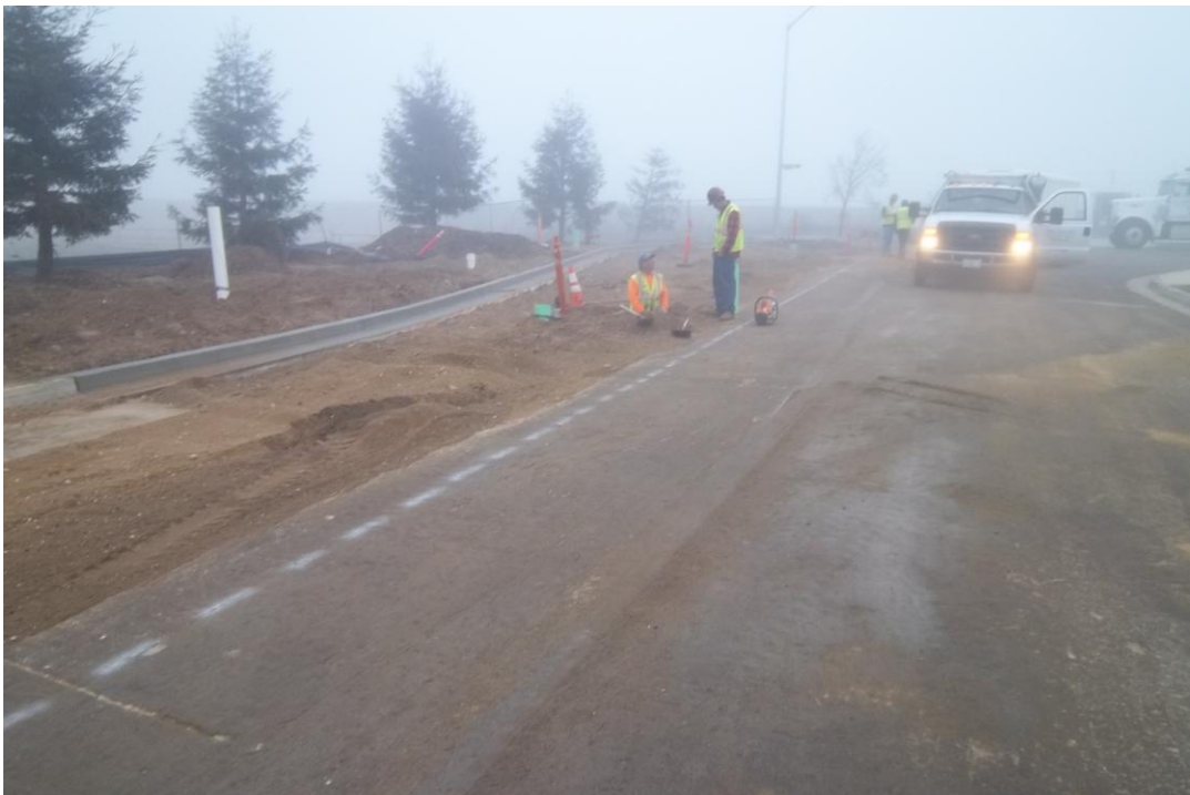
D-KAL preparing to sawcut trench for final paving section at Blosser and Atlantic.
