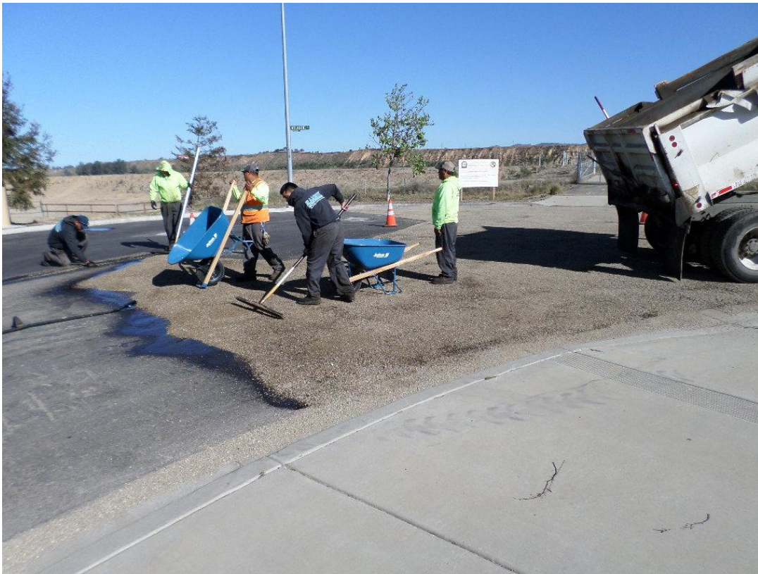
Ramsey Asphalt placing slurry at Blosser and Atlantic per the request of the City of Santa Maria.
