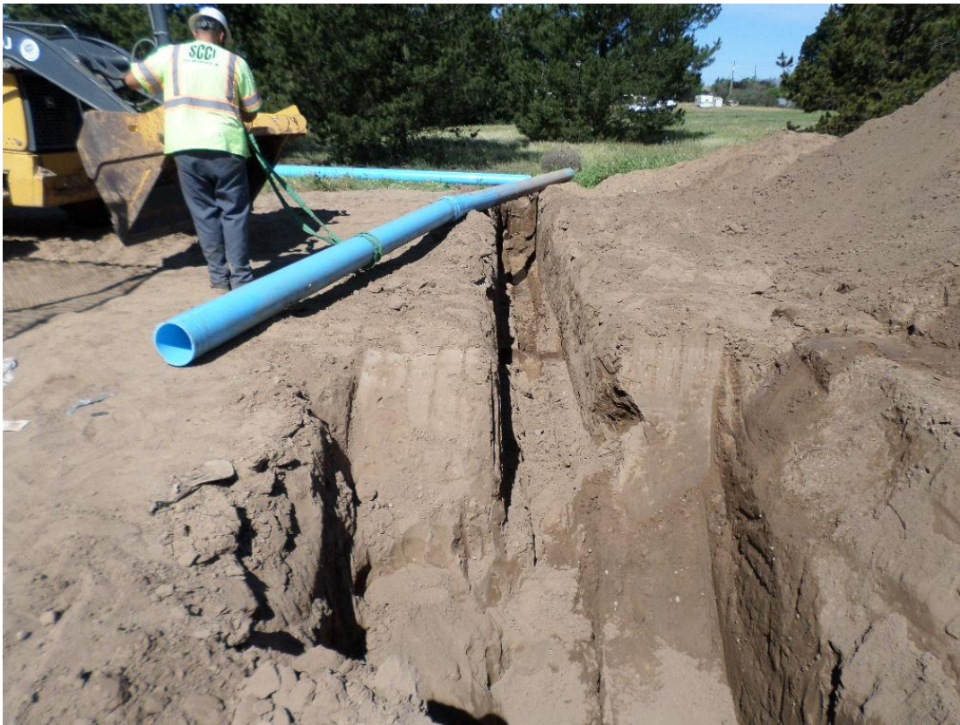
Removing temporary bypass piping after the final tie-in was completed at the PRV vaults.
