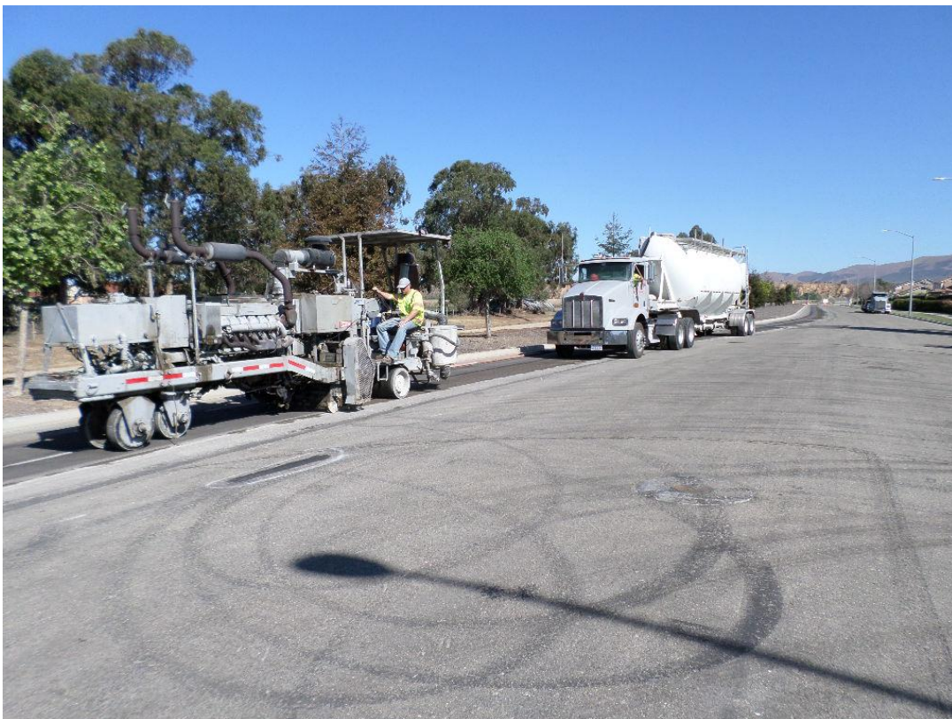
Grinding of the trench being performed under Ramsey Asphalt per the request of the City of Santa Maria.
