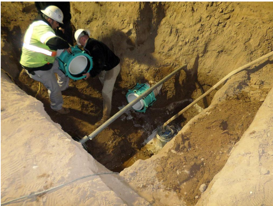
Spiess completing final tie-in on District's existing water main at PRV vault.
