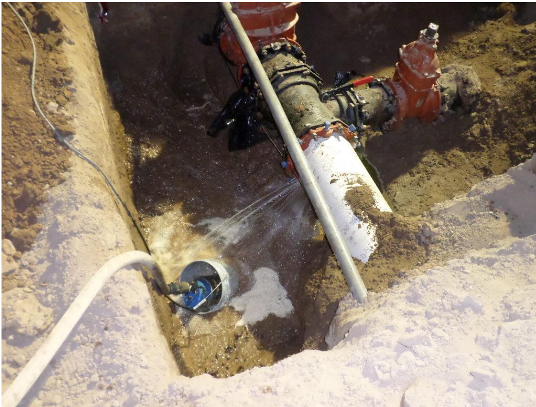
Spiess performing night work to drain the District's existing 12-inch water line and remove tee used for temporary bypass.
