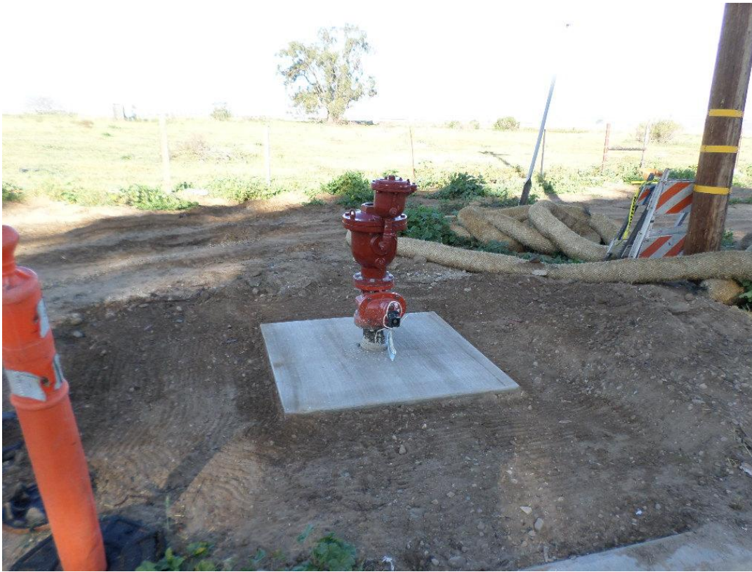
Combination air release valve installed and pad poured prior to cover being installed.
