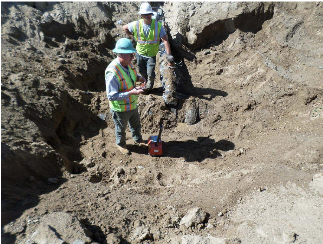
Fugro on site at Blosser and Atlantic where D-KAL has removed the test plate and is backfilling in preparation for paving.
