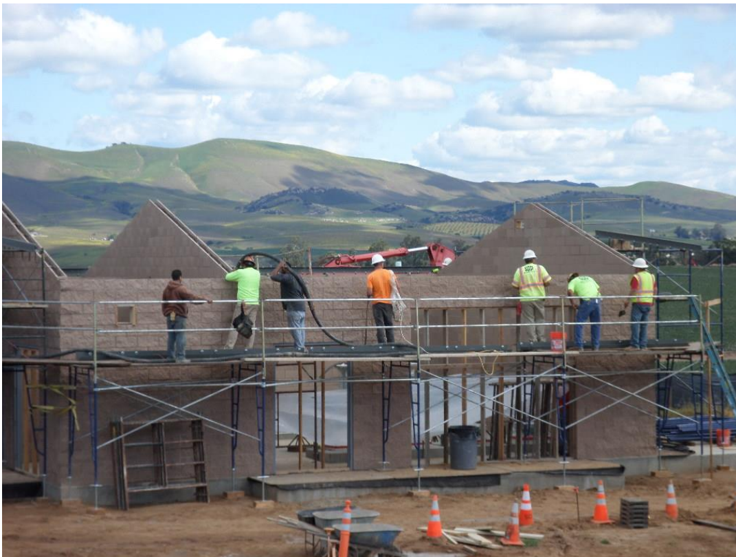
Boydston Masonry pouring final grout while Spieß set steel plates for roof.
