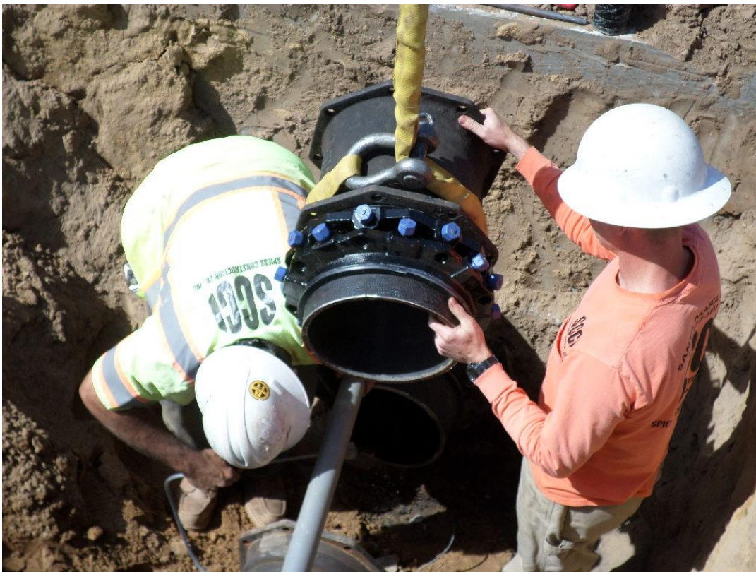
Spies making the final tie-in to the 12-inch water line at the PRV vault.
