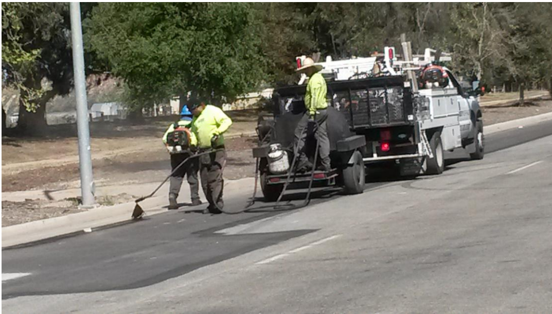
Ramsey Asphalt re-oiling trench edges of previously paved areas and oiling rock pockets in pavement.
