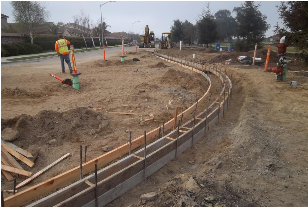
D-KAL forming curb and gutter replacement at Blosser Road and Atlantic Place.
