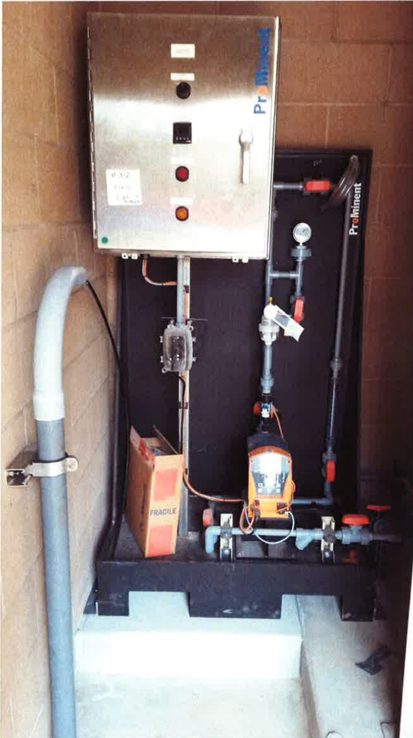
Chemical feed skid delivered and installed.
