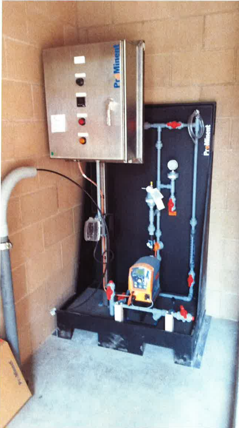
Chemical metering skid installed.
