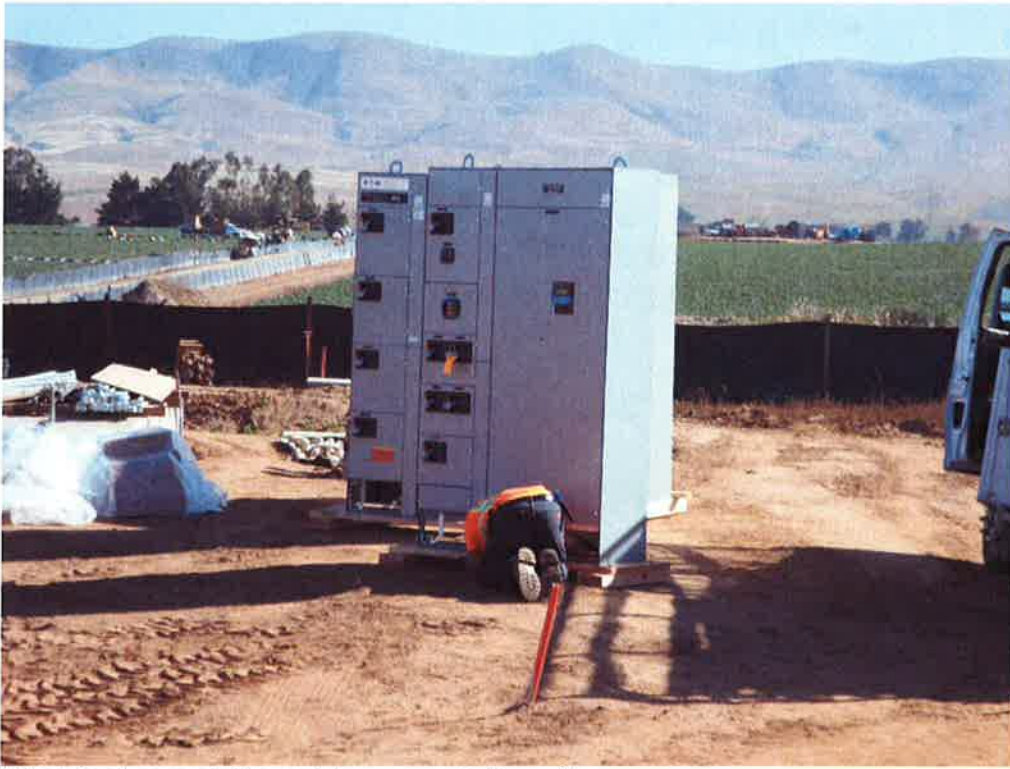
Electrical gear delivered to pump station site.
