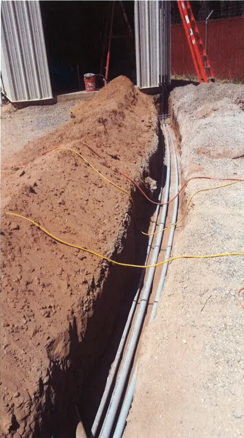
St. Denis Electric installing underground conduit from existing building to new chemical building.
