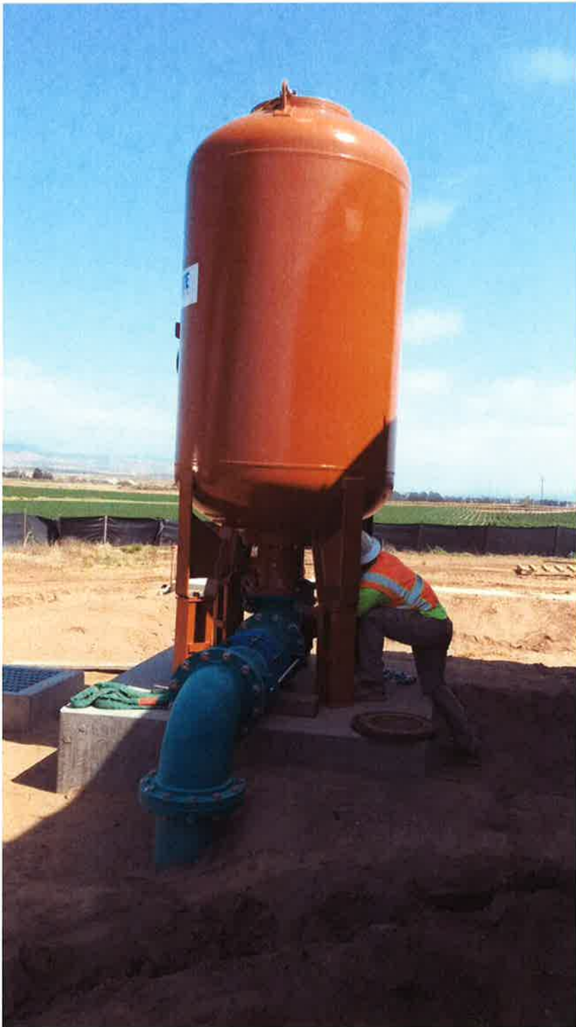
Surge tank in place on concrete pad.
