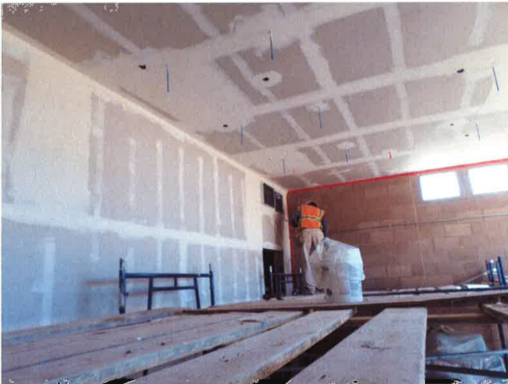
Ely Dodson Construction applying topping to sheet rock at pump station building.
