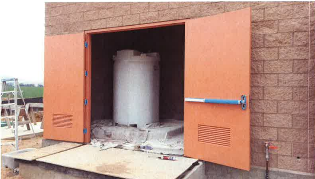
Coast Painting applying prime coat to interiors of doors at pump station.
