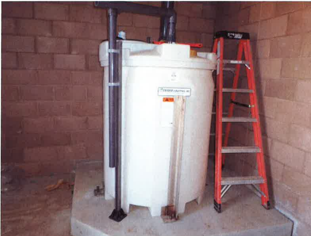
Spiess installing chemical tank hold downs and fill piping in both chemical rooms.
