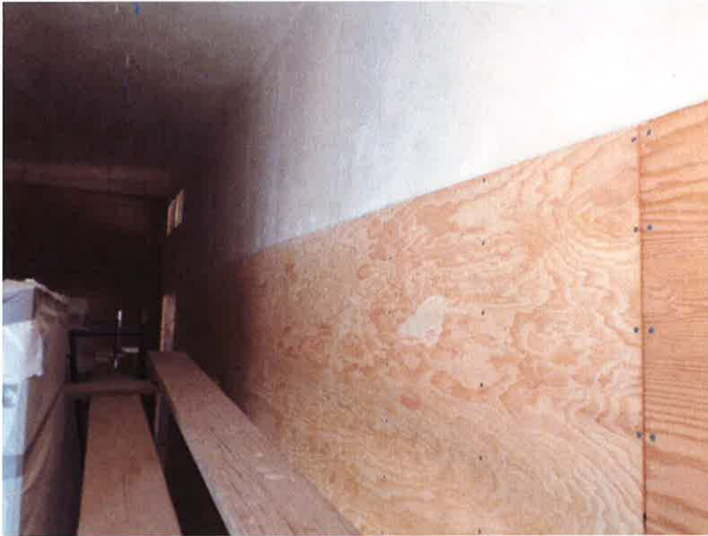
Ely Dodson Construction installing plywood on wall between pump room and electrical room.
