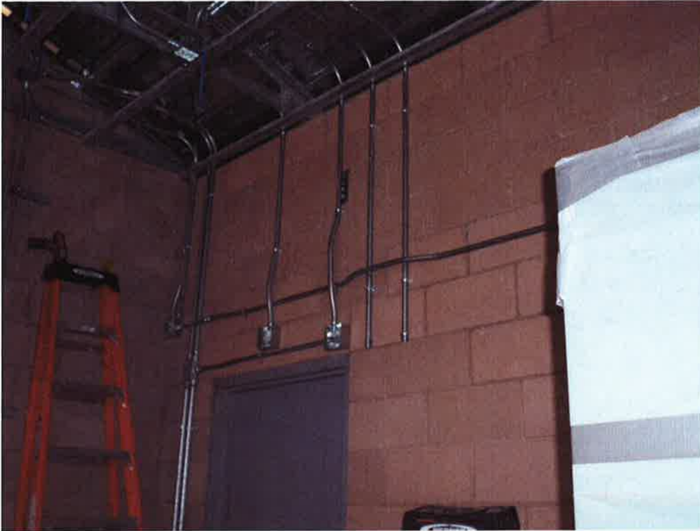
St. Denis Electric installing conduit and receptacles inside electrical room at pump station.
