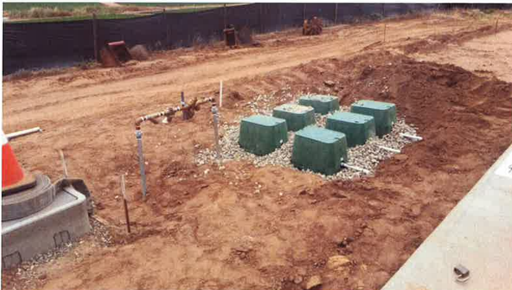
Controllers and meters installed for landscaping at pump station site.
