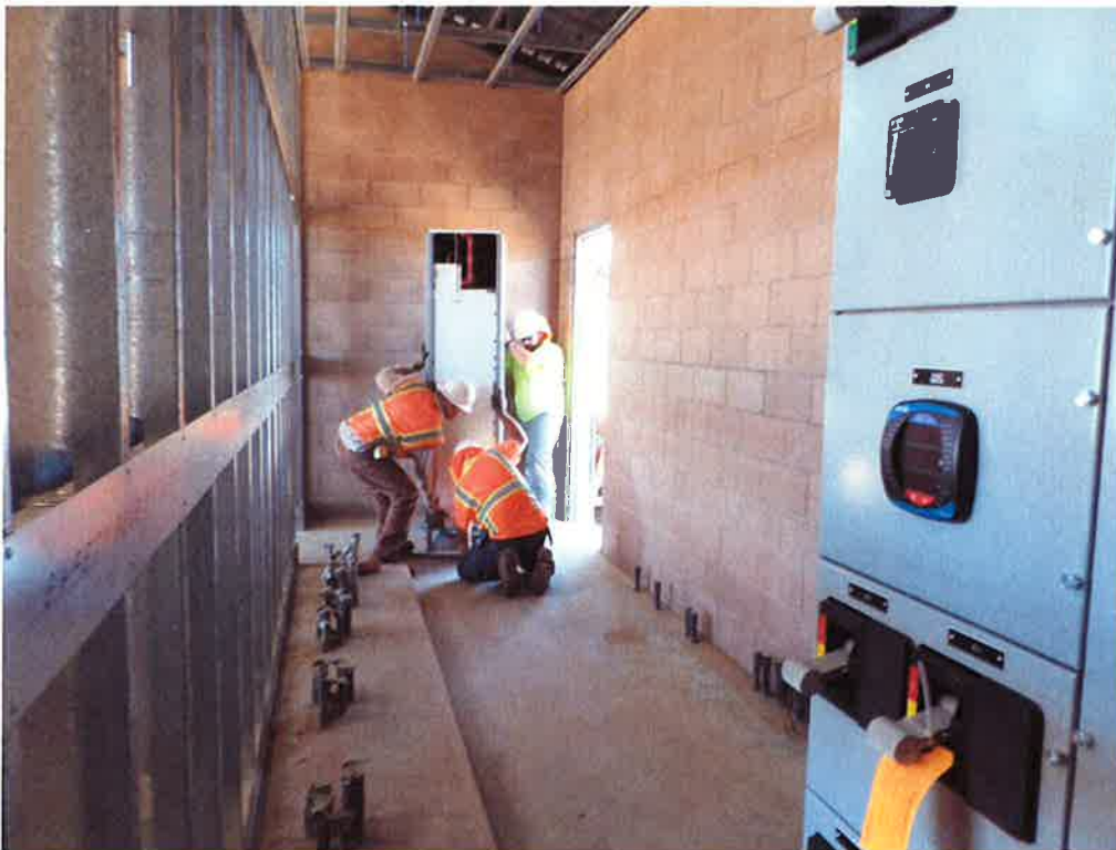
Spiess and St. Denis Electric staging electrical equipment inside pump station building.
