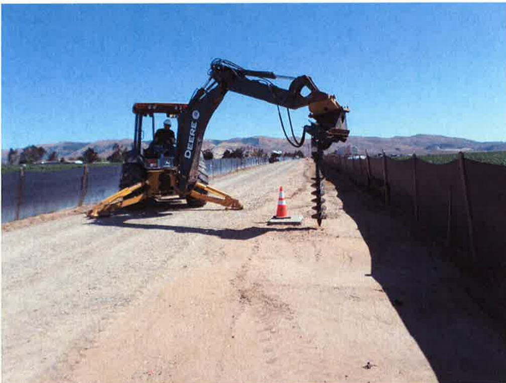
Spiess auguring holes in access road for bollards at AT&T pull boxes and other appurtenances.
