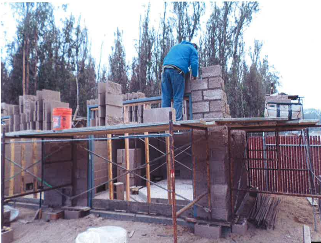
Rocky Boydston Masonry working on second course of block at chemical building.
