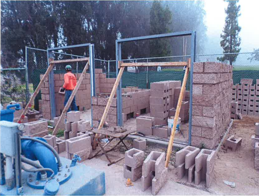
Door frames installed by Spiess and Rocky Boydston Masonry installing block walls at the chemical building.
