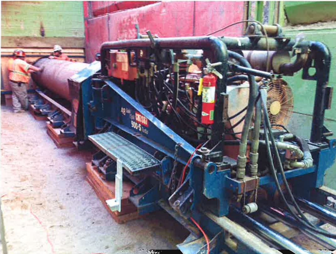
Pacific Boring operating bore and jack machine to begin boring first 36" steel casing section.
