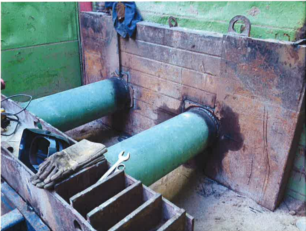
Pacific Boring installing back brace located behind the bore and jack machine.
