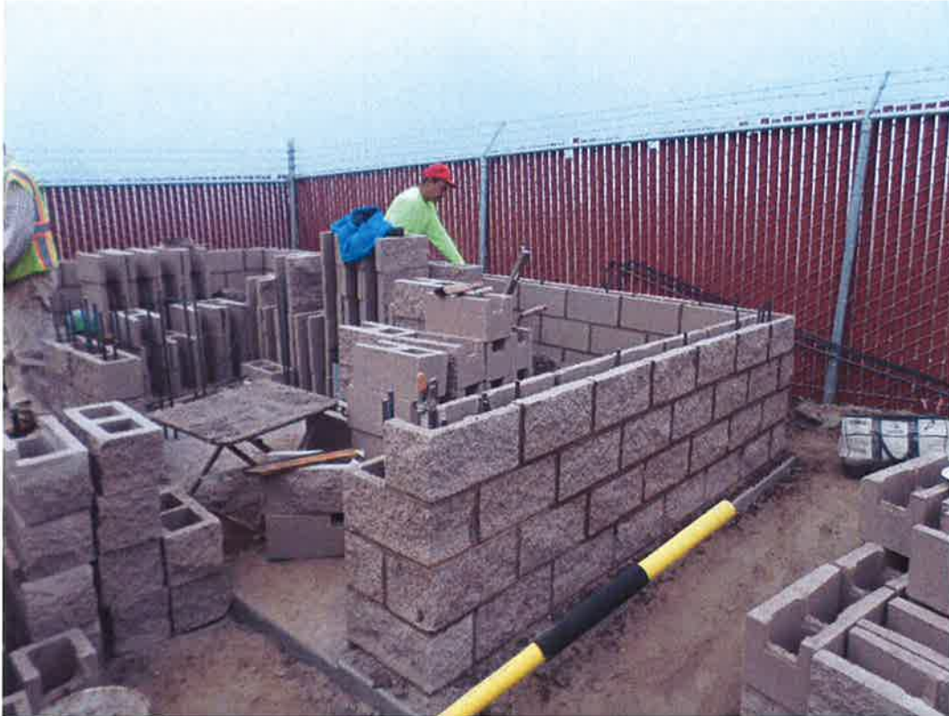
Rocky Boydston Masonry installing first course of block walls for the chemical building.
