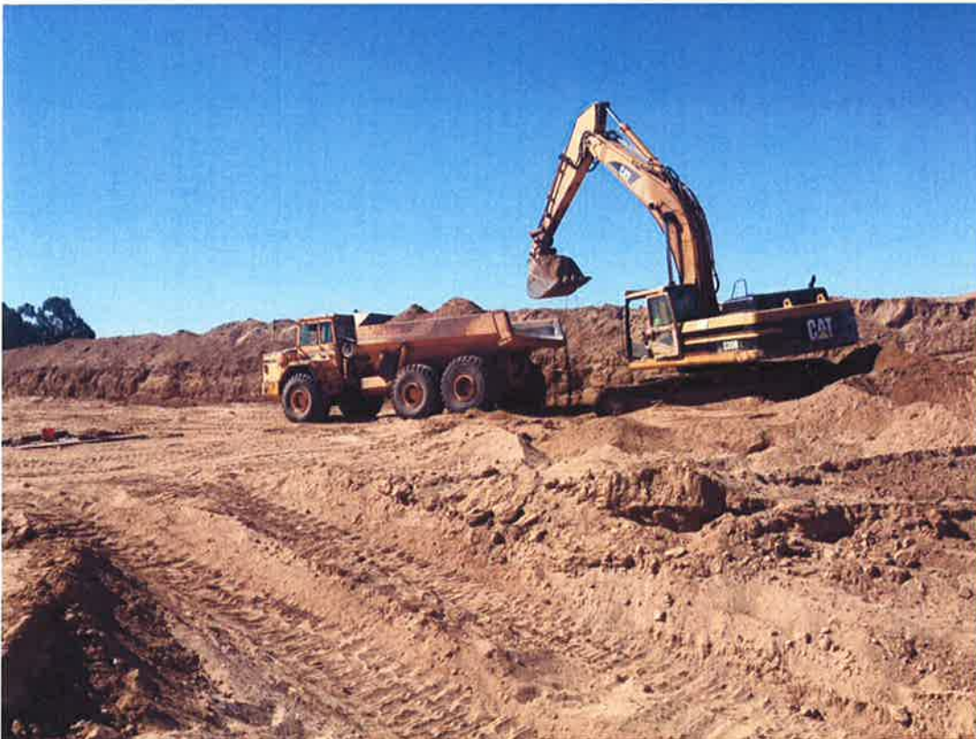
D-KAL hauling native material off-site to be screened and returned for use as backfill.
