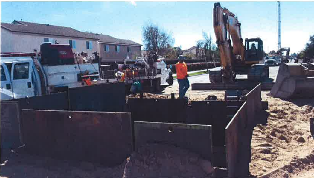
First layer of steel plates driving down between I-beams at receiving pit.
