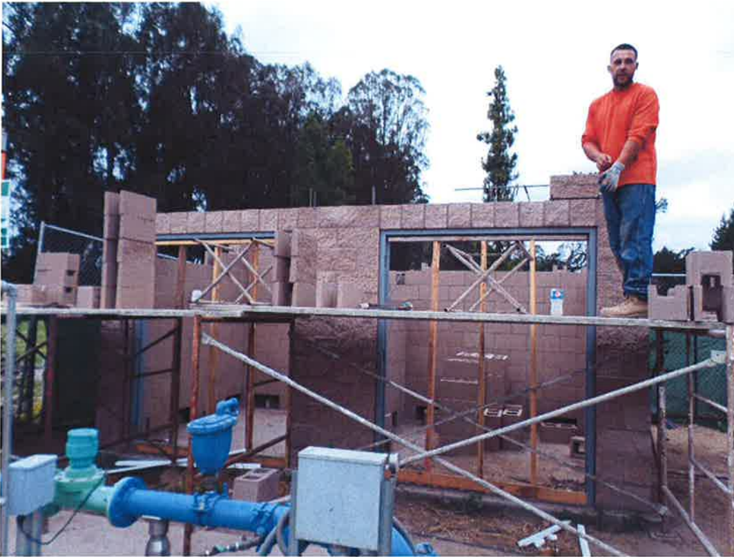
Rocky Boydston Masonry installing second course of block walls at chemical building.
