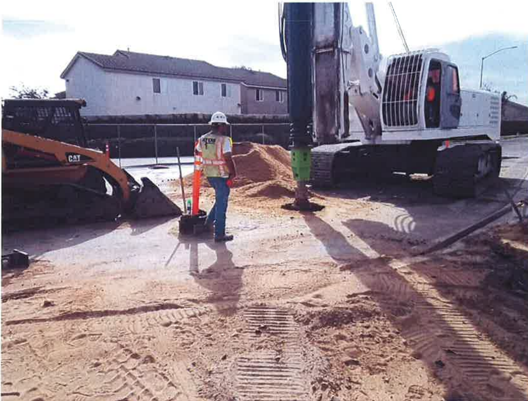
D-KAL subcontractor Meyers Drilling installing steel I-beams in Blosser Road for the receiving pit.
