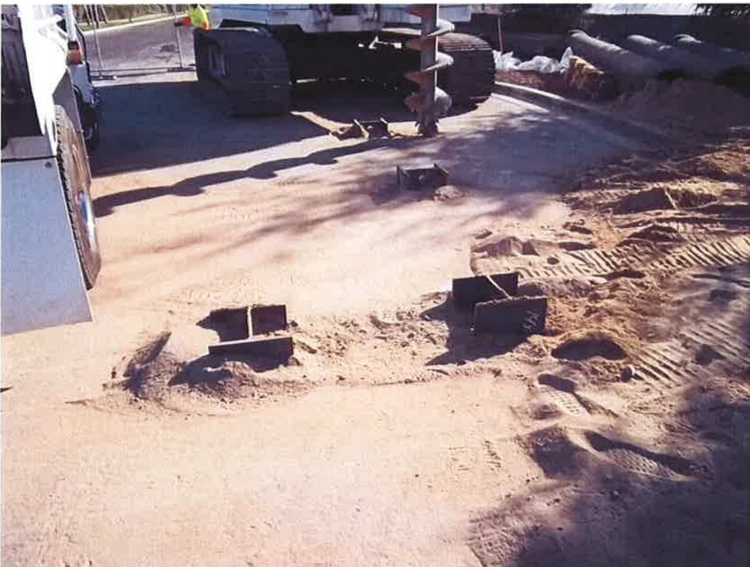
I-beams in place in Blosser Road for steel plate supports in the receiving pit.
