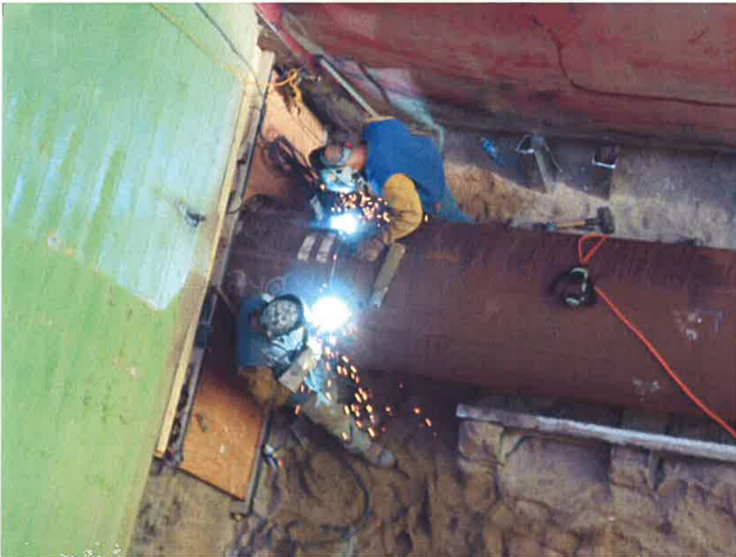
Pacific Boring welding another section of 36-inch casing to the one installed.
