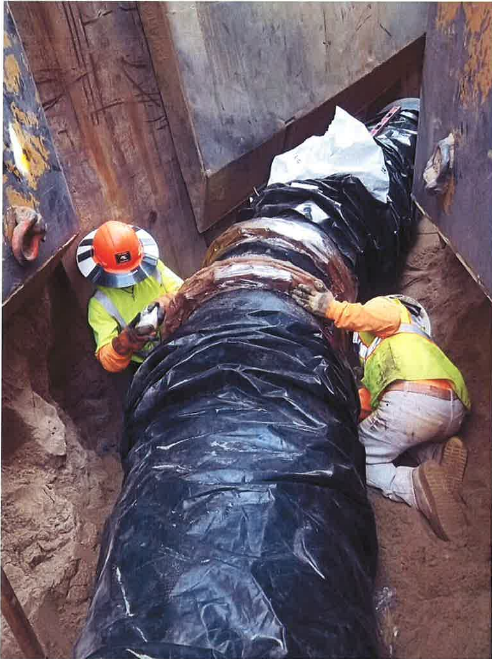
D-KAL installing wax tape on joints of the 22-1/2 bend fitting on the deep trench pipe.
