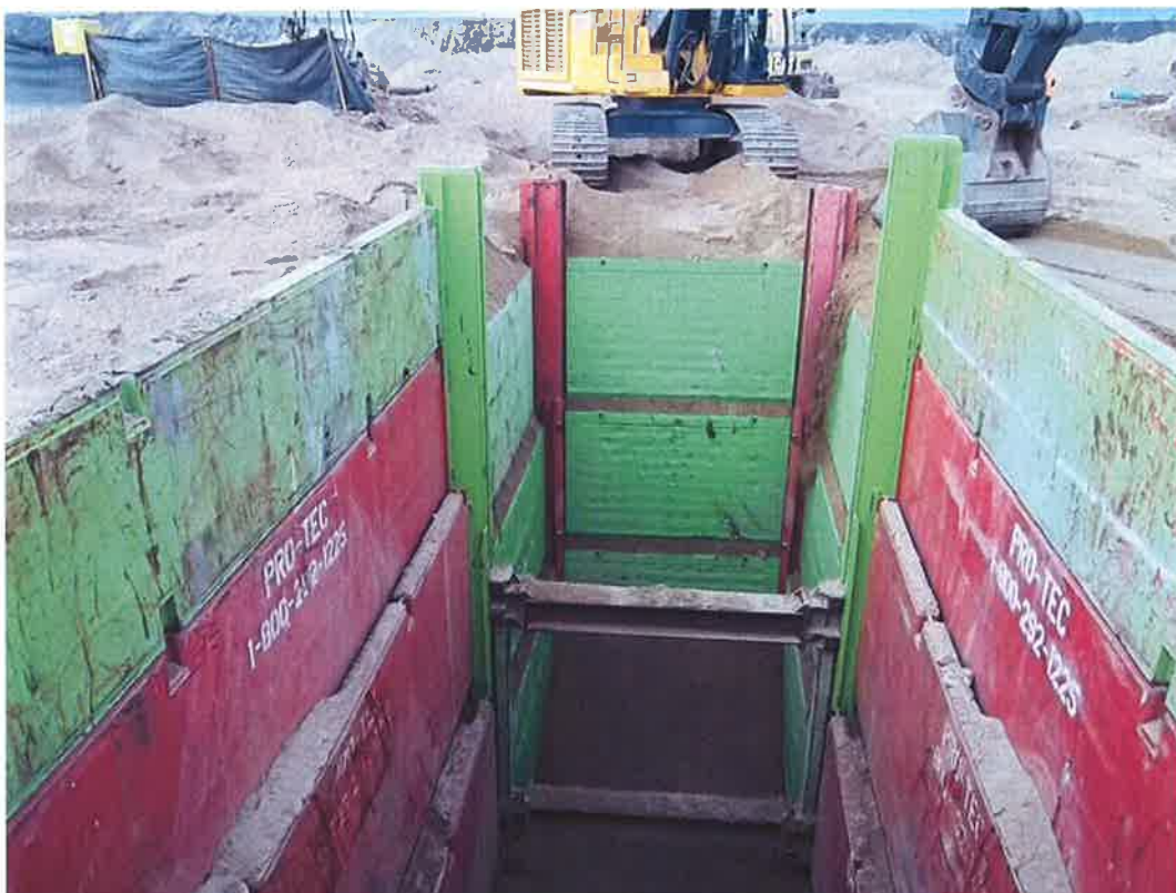
D-KAL continuing excavation of bore and jack pit and installation of slip shoring.
