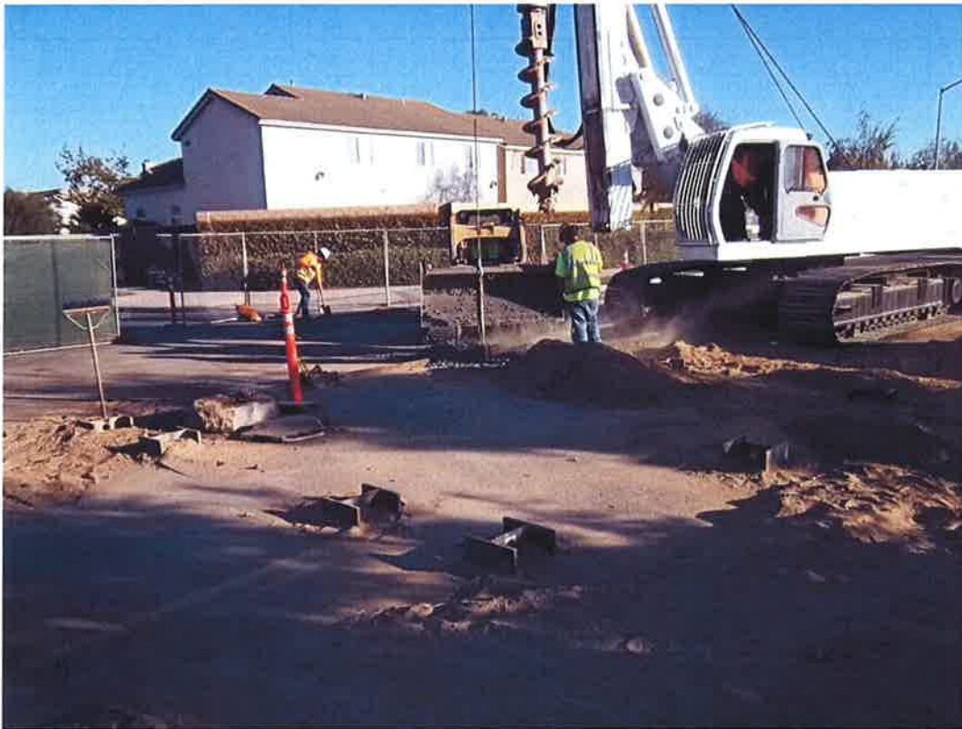
Meyers Drilling finishing installation of I-beams in Blosser Road for steel plate supports in receiving pit.
