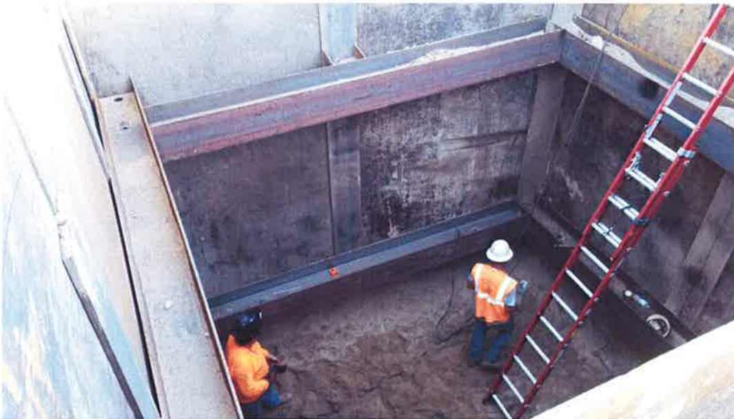
D-KAL welding second layer of horizontal supports inside the receiving pit at approximately 16 feet.
