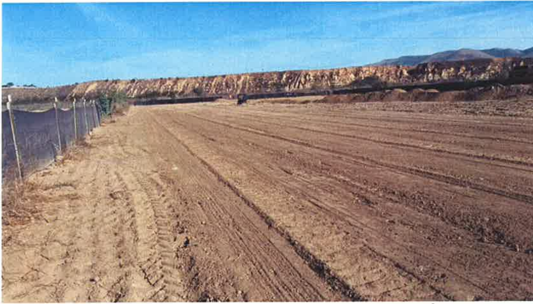
Agricultural topsoil restored up to silt fence along west side of temporary construction easement.
