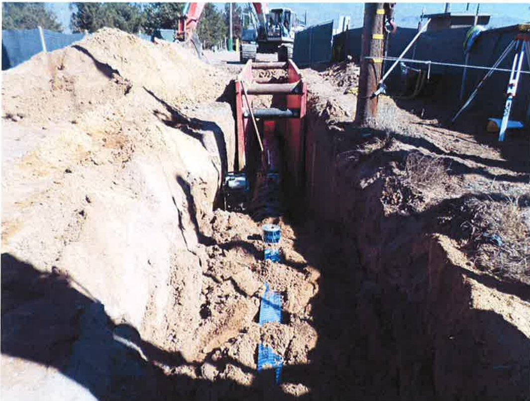
Spiess installing the 24-inch DIP past the PG&E power pole at the edge of the access road while the pole is supported by PG&E.
