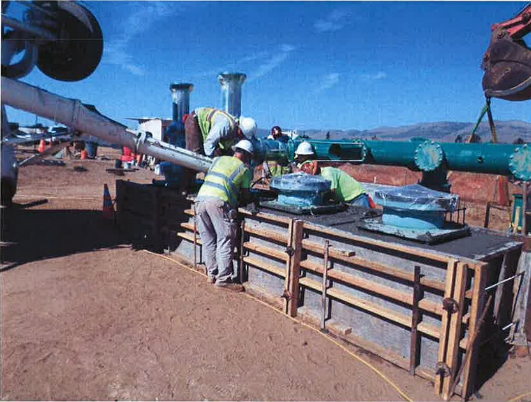
Spies pouring the pump pedestals at the same time as the discharge pipe encasement.
