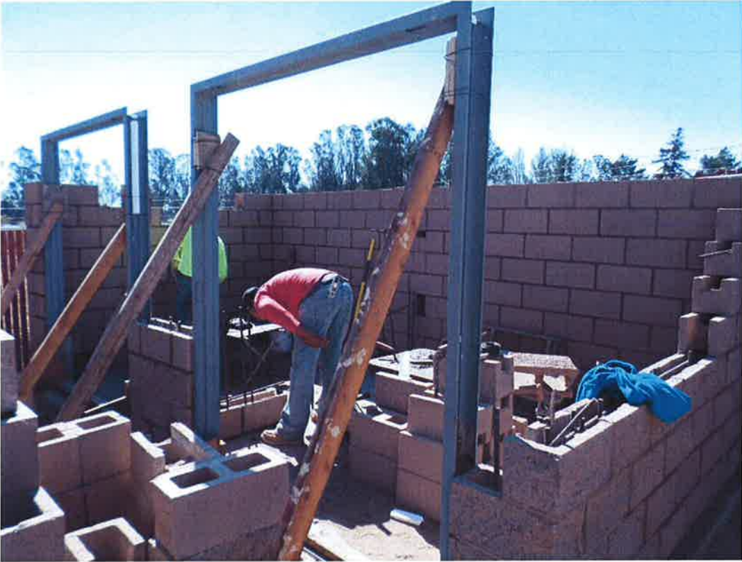
Door frames set by Spiess and Rocky Boydston Masonry constructing block walls at the chemical building up to 5'-4".
