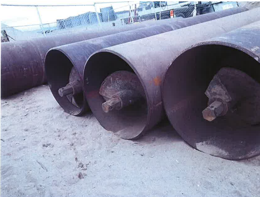
Steel casing staged for installing into bore and jack pit, with auger sections inside.
