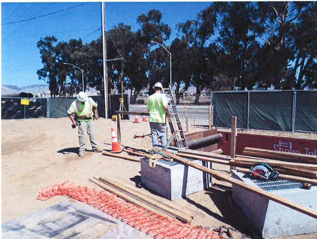
Spieß installing the safety hand rail around the top of the vault shoring.
