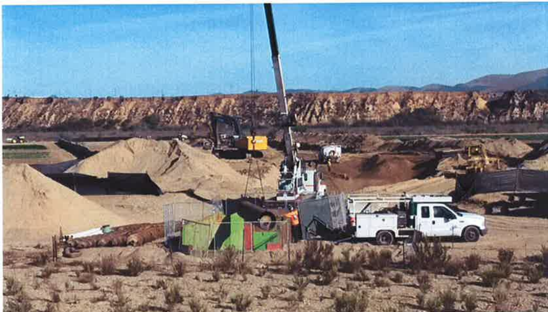
Pacific Boring placing another section of 36-inch steel casing pipe and auger into bore and jack pit.
