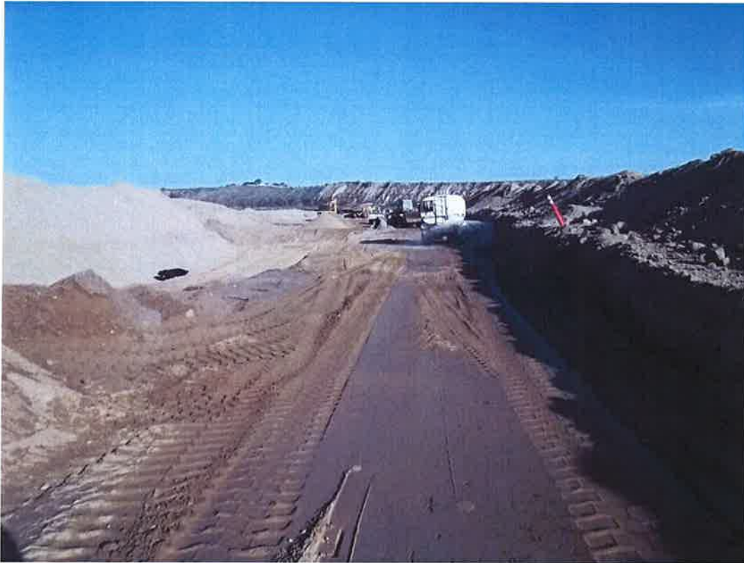
D-KAL watering and maintaining access road along deep trench in river area.
