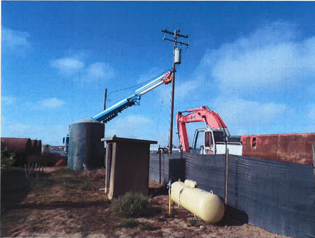
PG&E supporting power pole at edge of access road while Spiess installs the 24-inch DIP.
