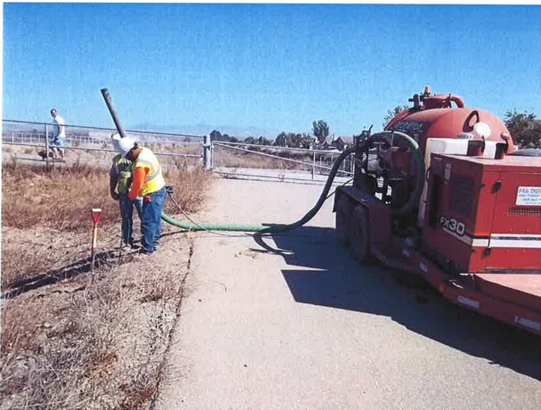
D-KAL installing settlement monitors on the levee to monitor any changes during the bore and jack operation.
