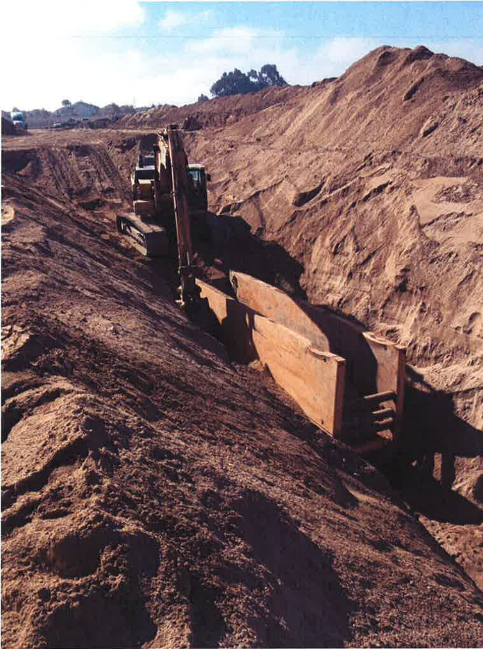
D-KAL excavating beside trench shield to set it in place for more pipe installation.
