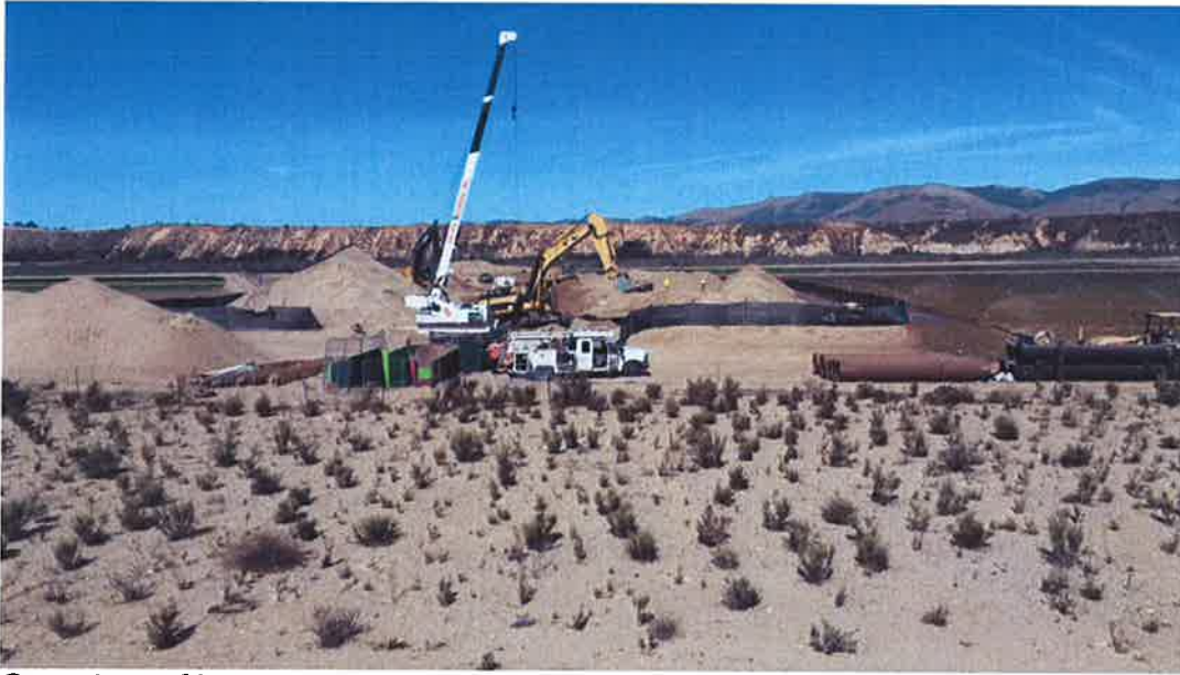
Overview of bore and jack pit and Pacific Boring operation in river area.
