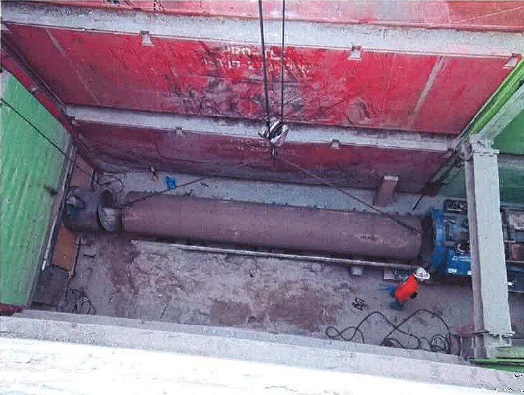
Pacific Boring installing another section of 36-inch steel casing pipe into bore and jack pit.
