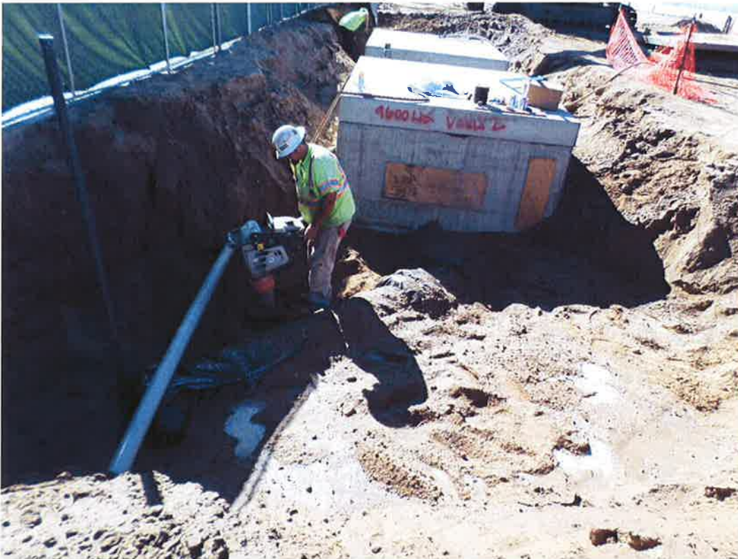
Piping to and from vaults installed and Spieß backfilling and compacting around piping and 4-inch Verizon line.
