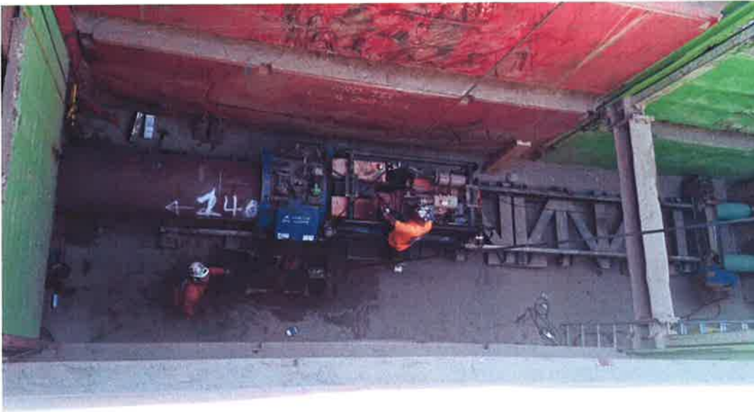
Removing material from bore and jack pit with clam shell and crane.
