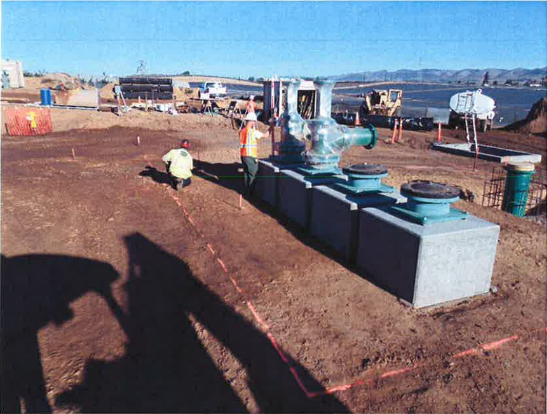
Pump pedestals poured and forms removed. Spiess laying out pump station building foundation.
