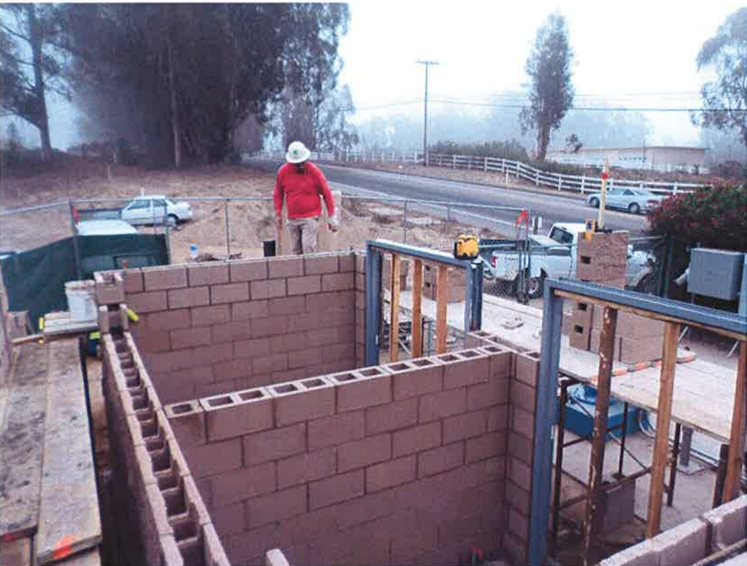
Rocky Boydston Masonry installing second course of block walls at chemical building.
