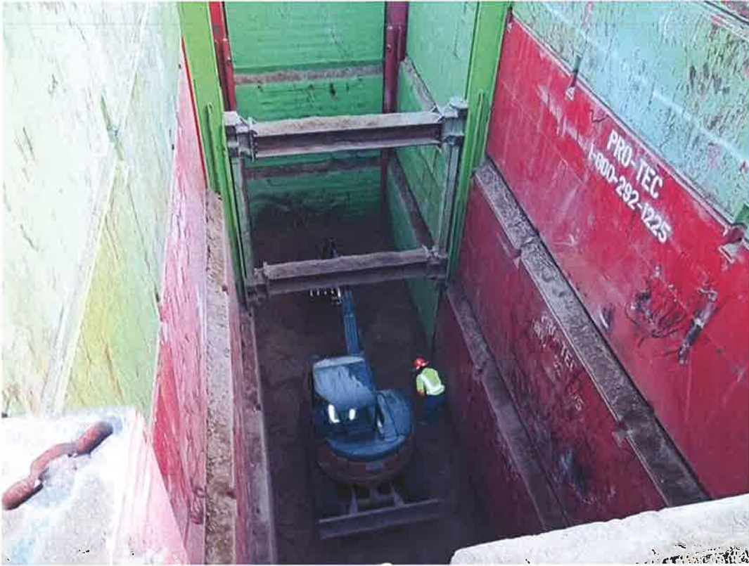
D-KAL using mini-excavator in the bottom of the bore and jack pit to reach grade.
