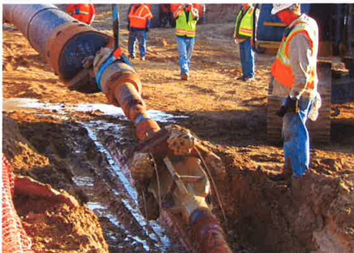
Figure 10. Reamer returns being checked before reamer leads the way for the swivel head and pipe.
