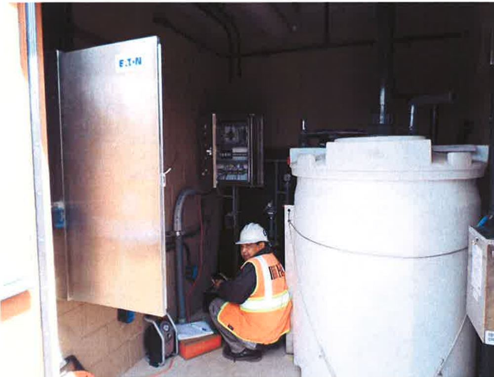
Hopkins testing chemical feed pump.
