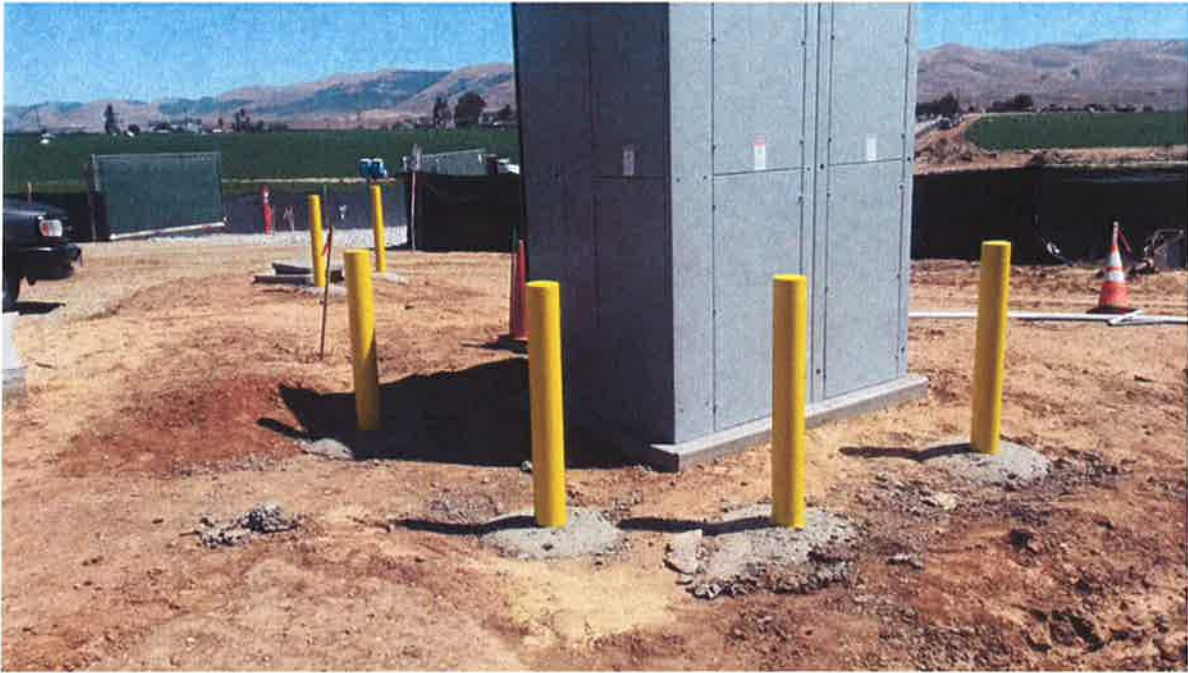
Bollards coated at PG&E electrical control panel.
