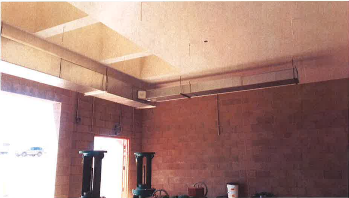
HVAC ducts installed in pump room.
