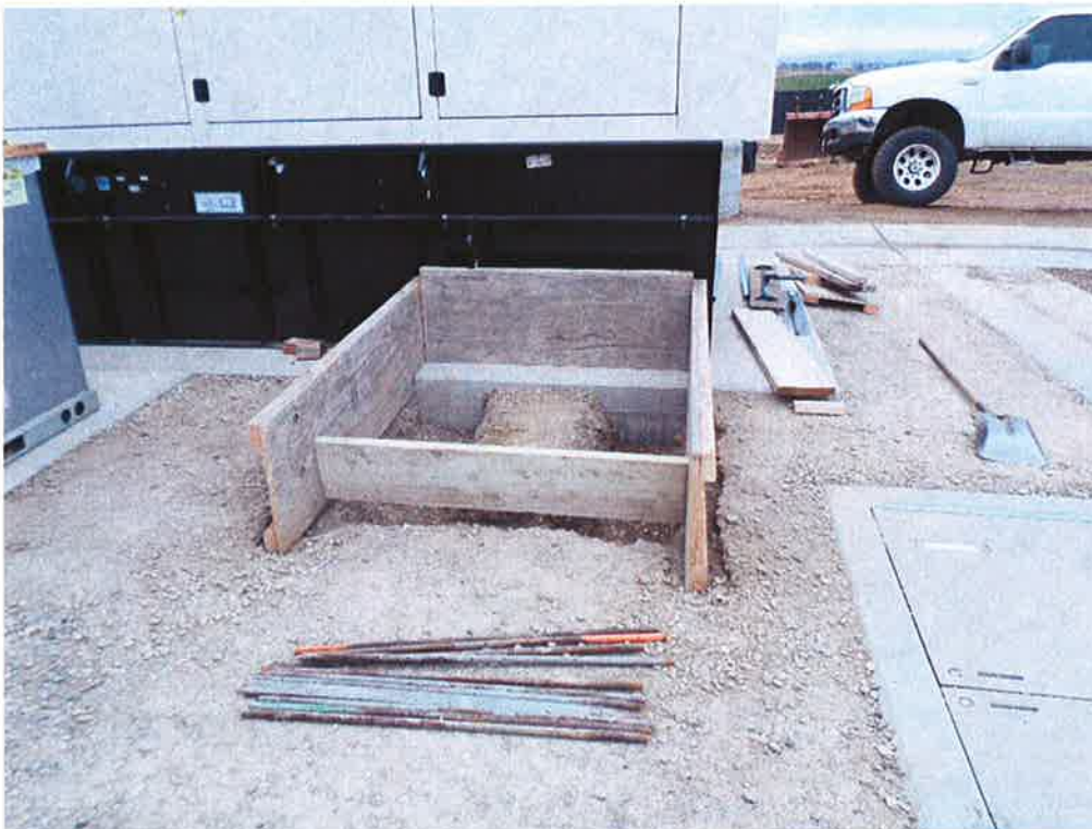
Spies forming steps to access emergency generator.
