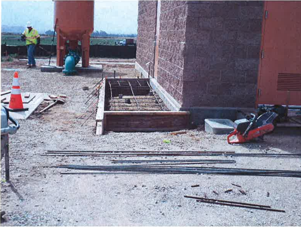
Spieß forming sidewalk to electrical room.
