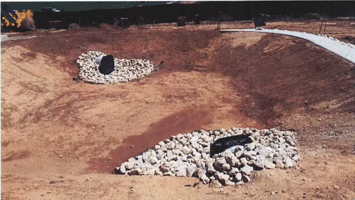
Retention basin with fabric and drain rock installed at storm drain inlets.
