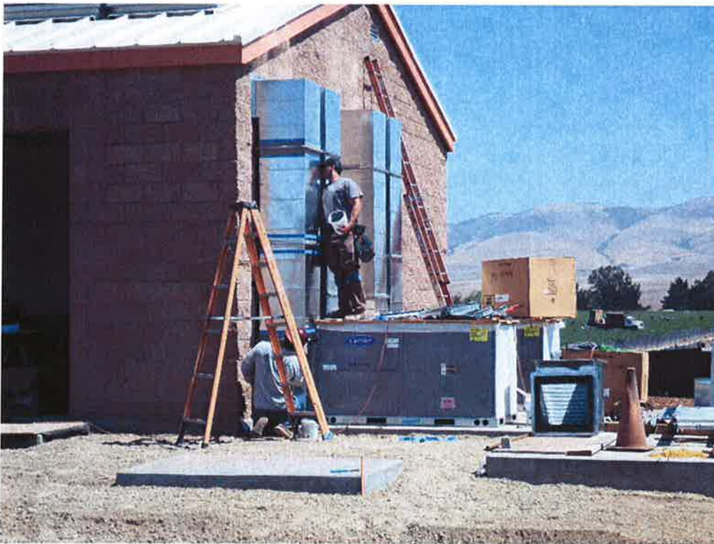
Exterior HVAC ducts installed.
