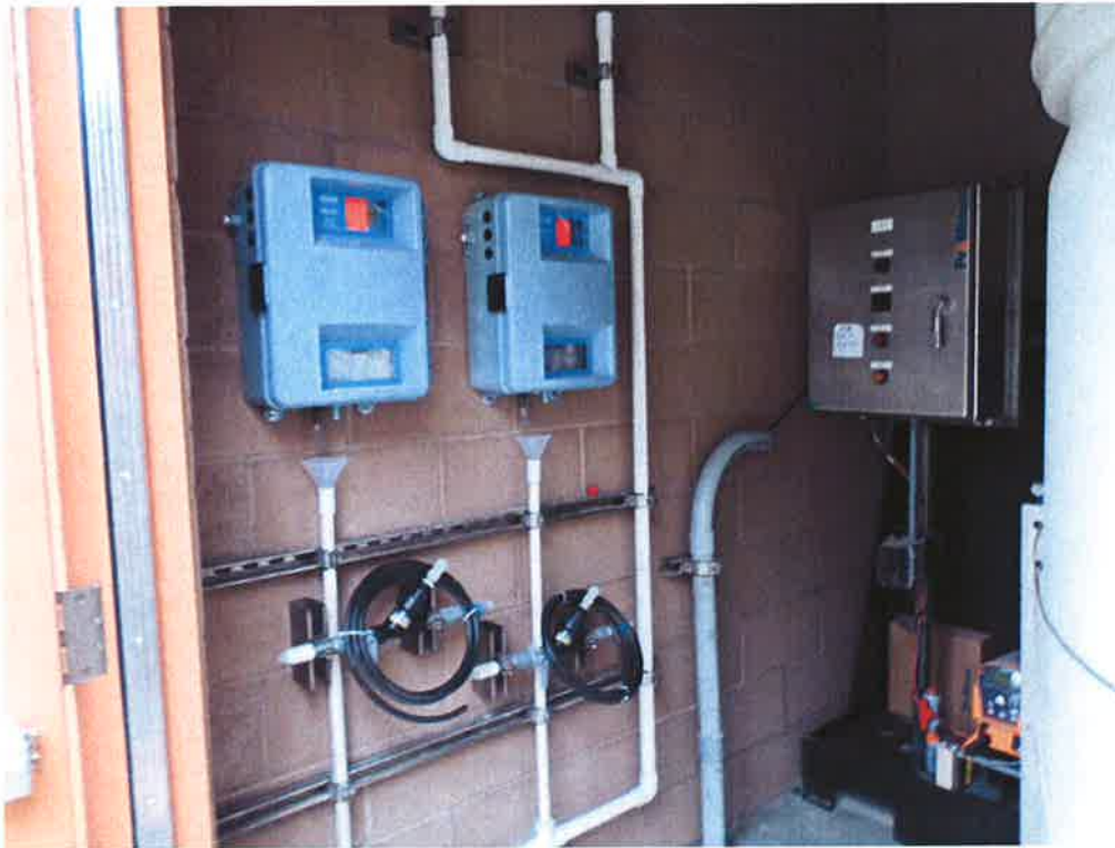
Chemical analyzer piping installed.
