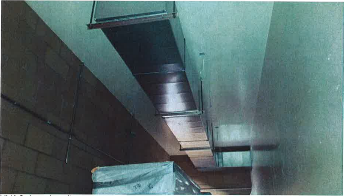
HVAC ducts installed in electrical room.
