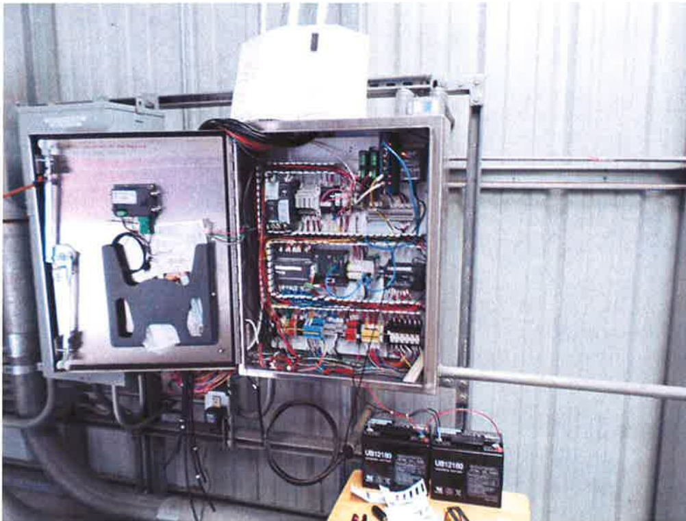
PLC panel and wiring.
