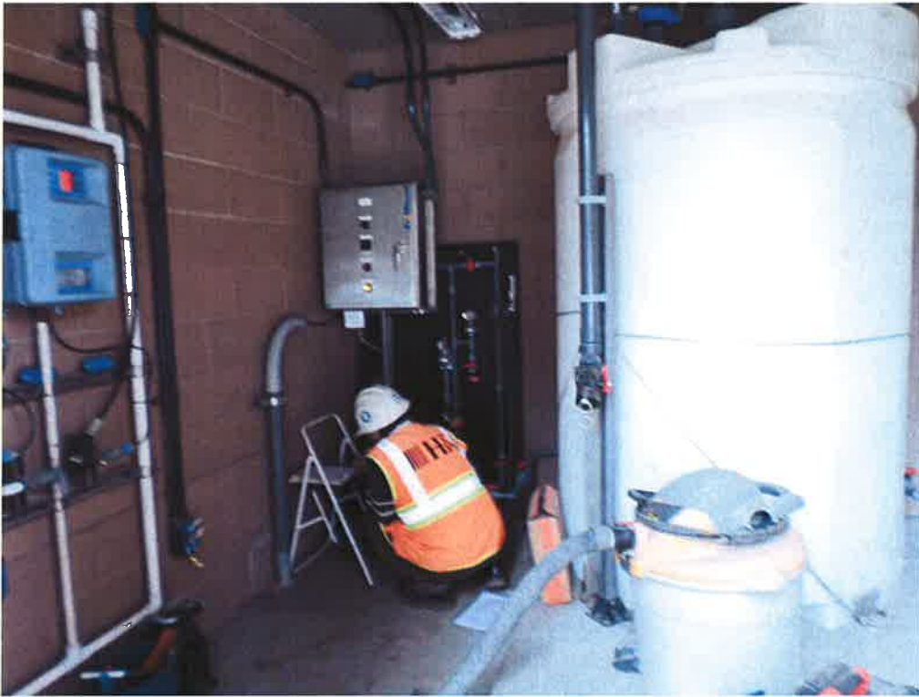
Testing chemical pumps.
