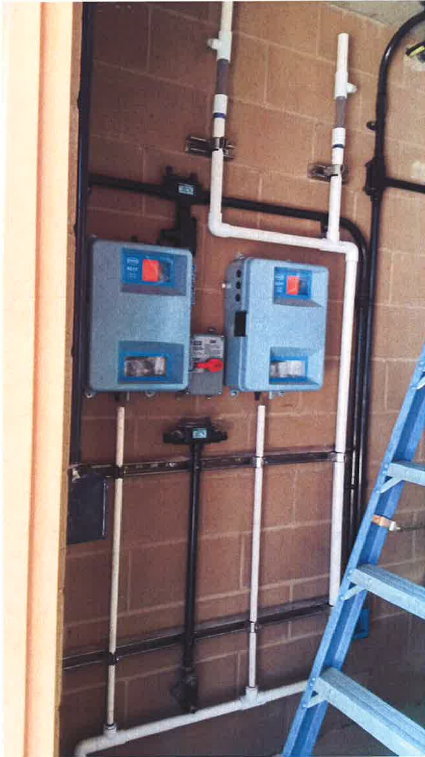
Chlorine analyzers installed.
