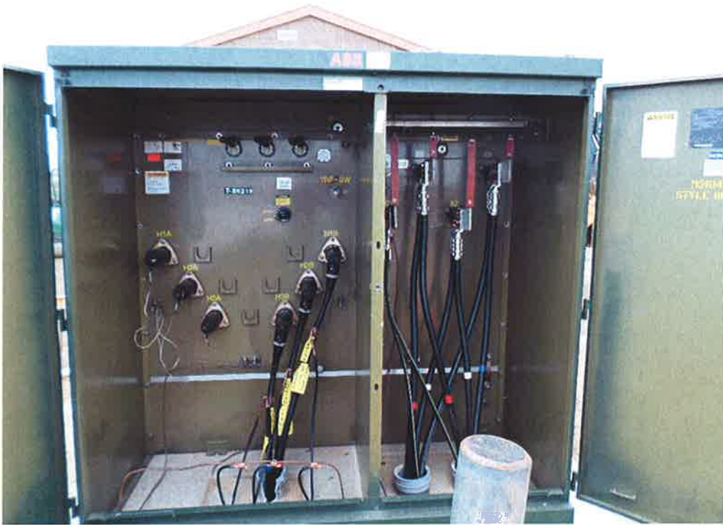
Electrical service terminated by PG&E at transformer.
