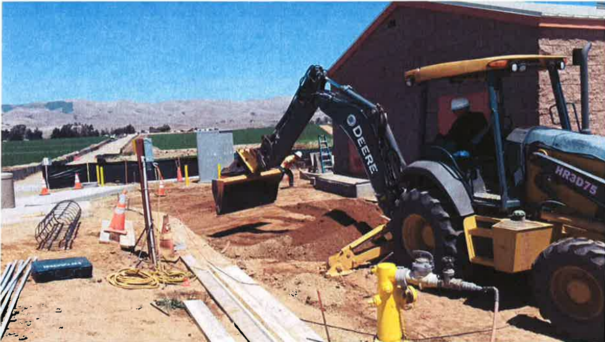
Spiess continuing to remove native material around site in preparation for installation of aggregate Base driveway.
