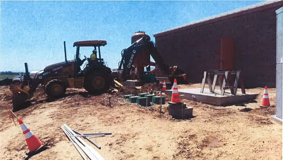
Spiess removing native material to prepare site for aggregate base installation for driveway.
