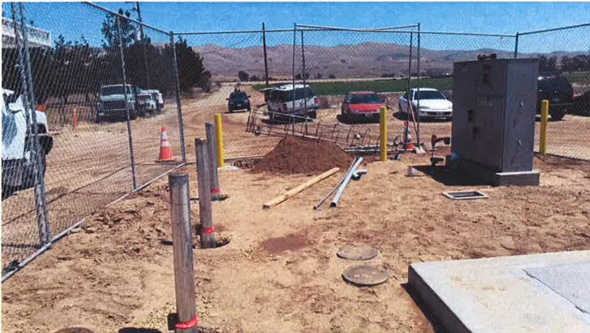
St. Denis Electric drilling for the SCADA antenna base at the PRV vault.
