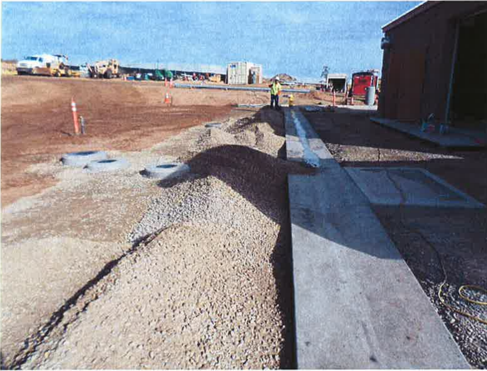
Spies placing aggregate base around valve cans and V-ditch for finish grade.
