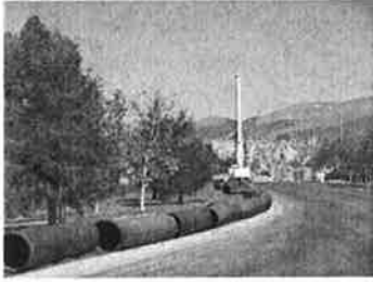
Piping on Blosser Road in Santa Maria - October 2014
