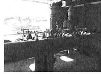
Supplemental water pump station - June 2015
