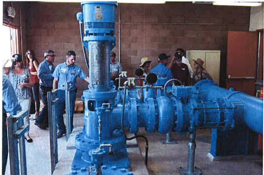
A ribbon-cutting for the Nipomo Community Services District's supplemental water project was held Wednesday, Sept. 9, 2015. These pumps restore water pressure after the water comes uphill from Santa Maria.
