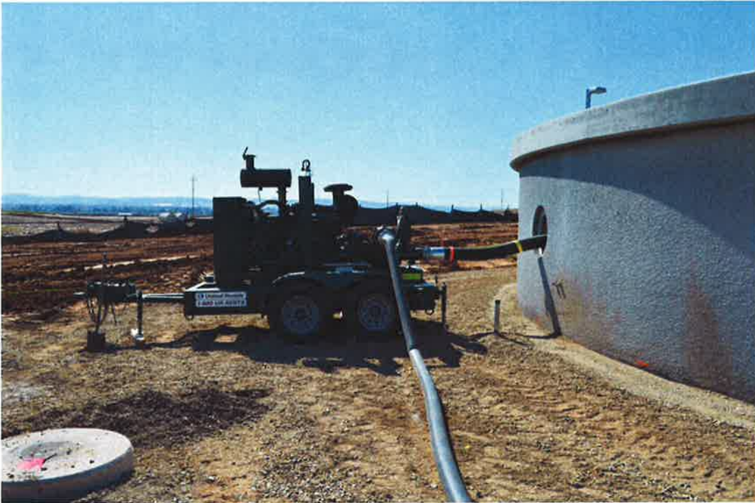
Trailer pump set up and draining reservoir to prepare for cleaning and disinfection.
