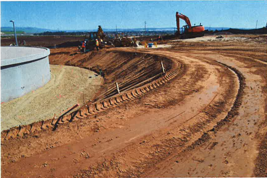
Shallow v-ditch graded around the top of the slope to prevent erosion of 3:1 slope.
