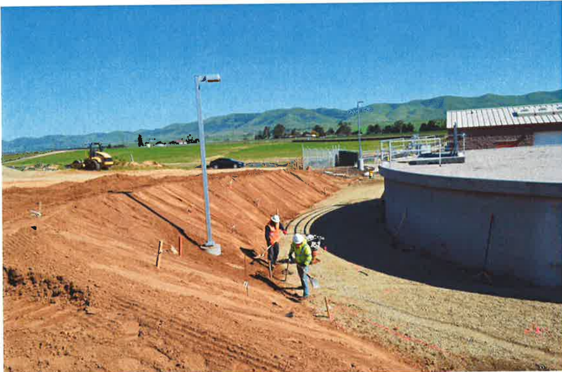
PHC fine grading around outside of Class II AB to prepare for curb and gutter.
