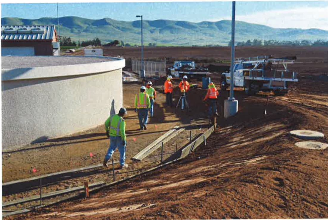
Lopez Engineering on site to form and pour concrete curb and gutter, v-ditches and splash pad.
