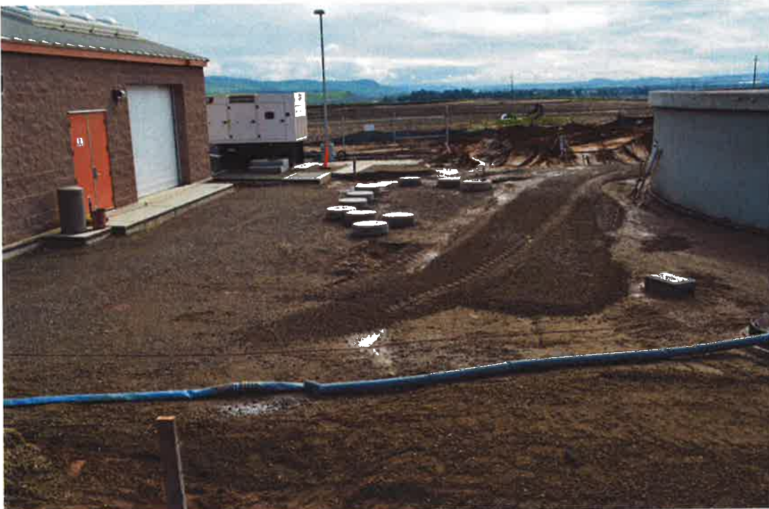
PHC placing Class II AB around reservoir.
