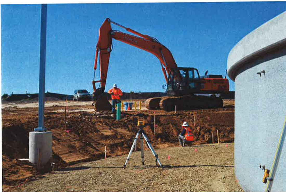
PHC checking and setting grades to prepare for construction of curb and gutter.
