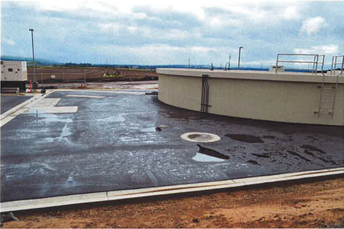
Ponding water after rain where areas will need to be repaired to drain.
