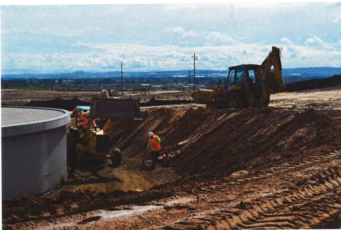
PHC placing Class II AB around reservoir.
