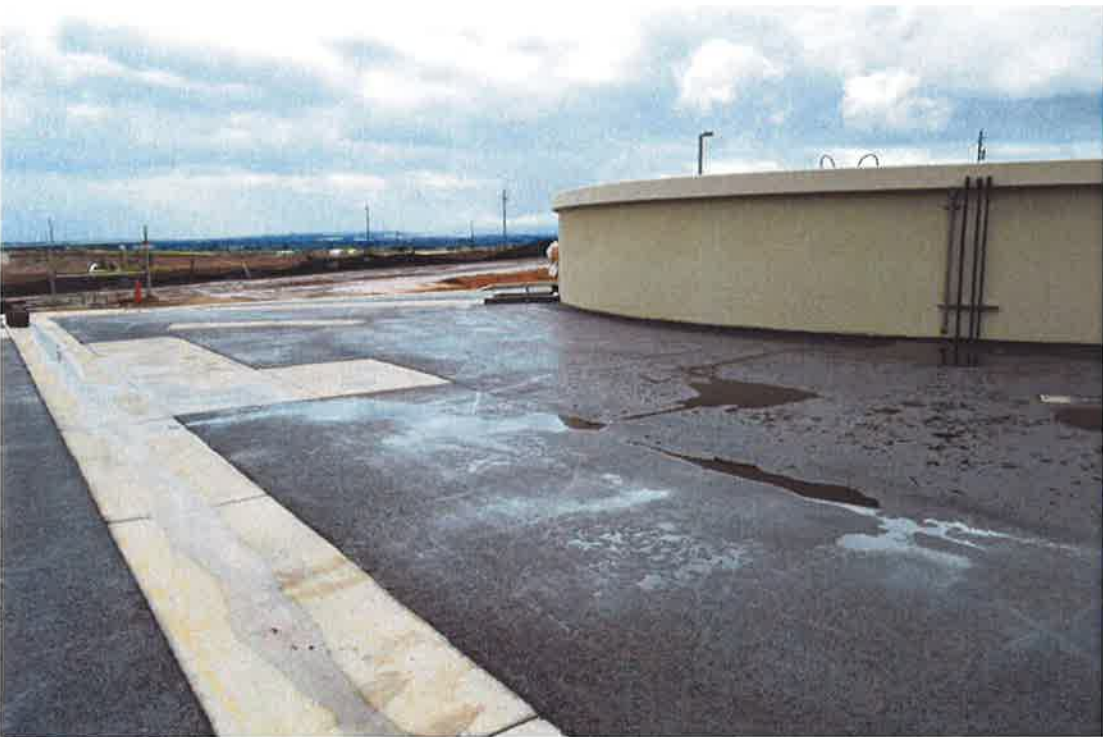
Ponding water after rain, concrete v-ditch flowing.
