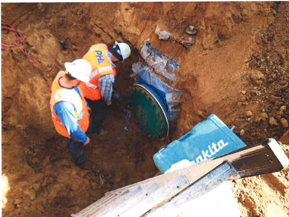
Connection to the reservoir inlet piping exposed at valve with blind flange.
