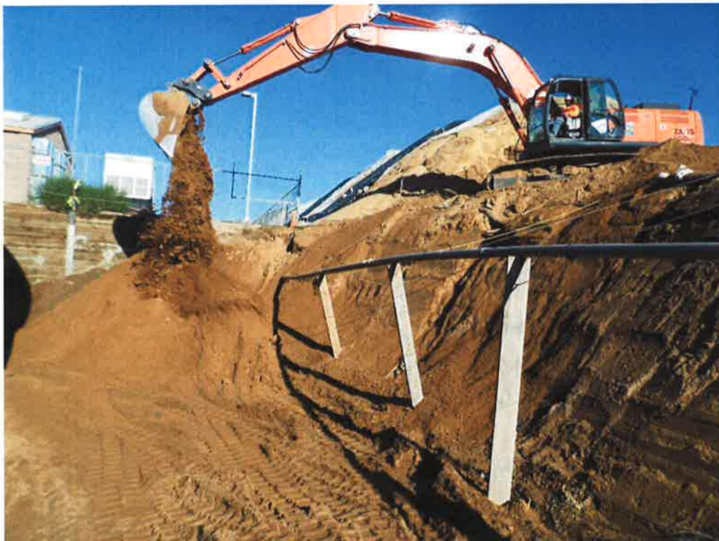
PHC using stockpile material to backfill around reservoir while avoiding electrical service to site.
