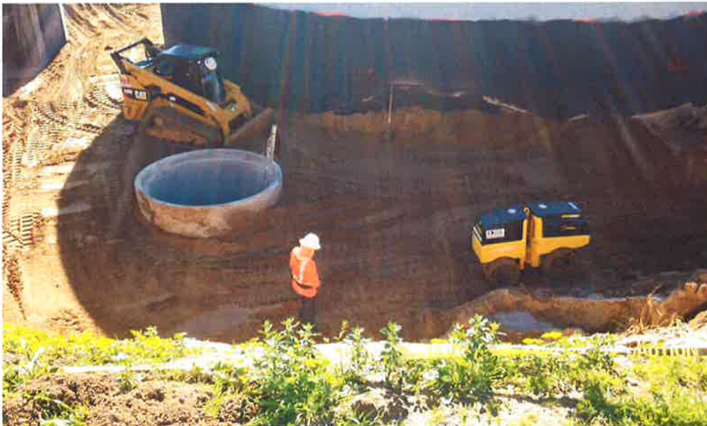
PHC using remote compactor to compact material over future reservoir pipe extension.
