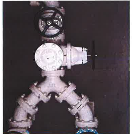
Lift station, wetwell, piping, pump and site improvement design plans and specifications were part of this project.
