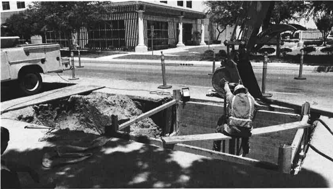
A major water main project on McCoy Lane, just west of Skyway Drive in Santa Maria. (Sean Larsen / KCOY photo)
