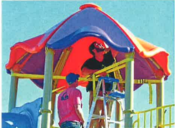
Workers build the new playground at Armstrong Park in Santa Maria on Wednesday. LEM WOOD, STAFF
