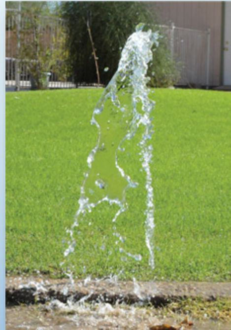
Broken sprinkler head
