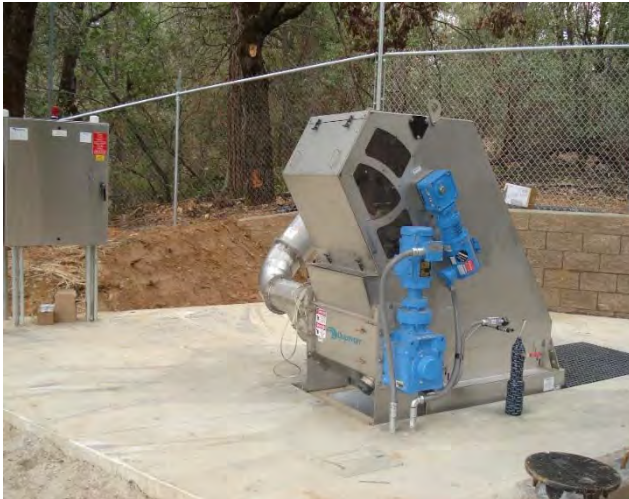
Duperon Low-Flow FlexRake® and washer compactor
