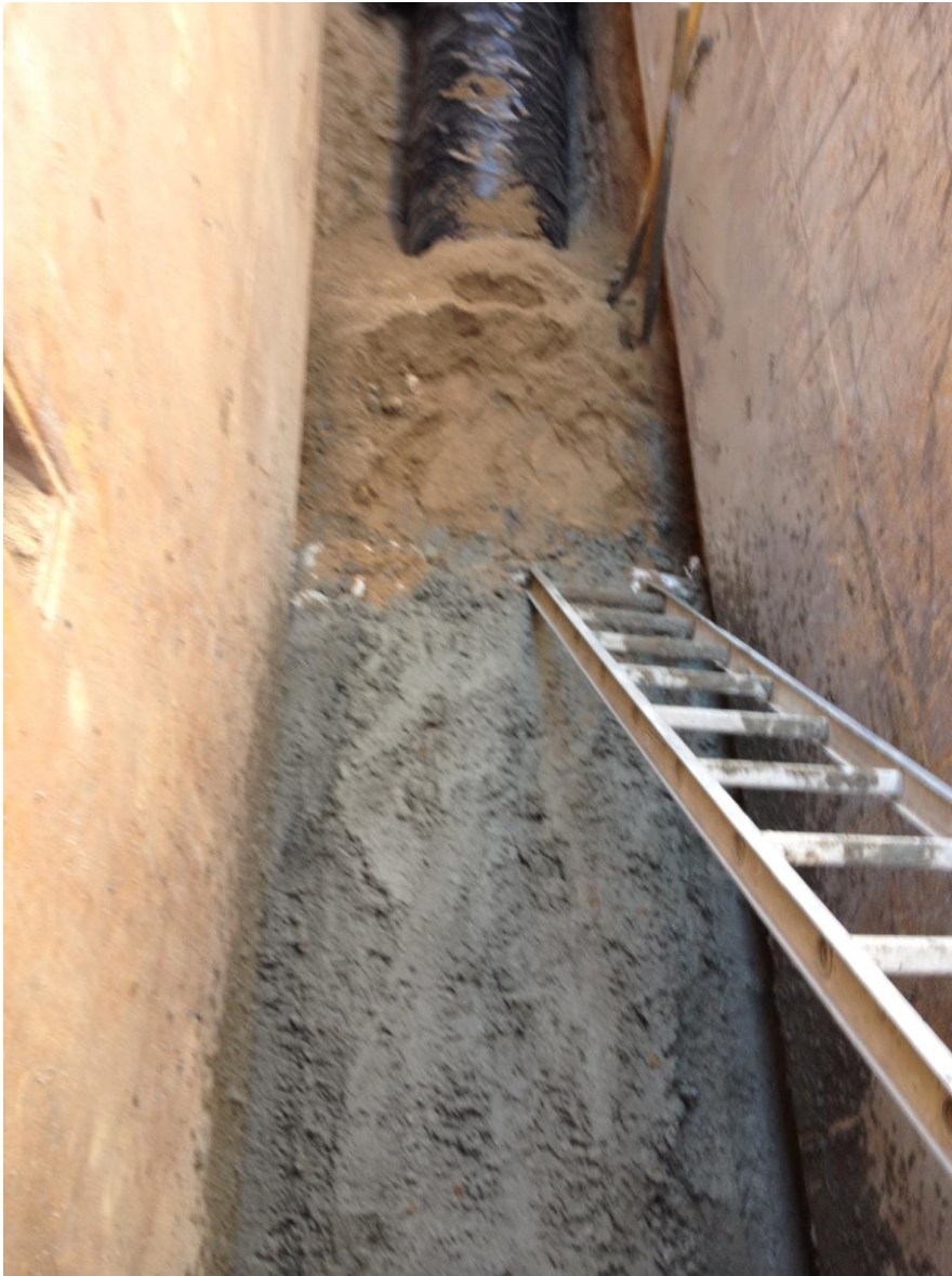
Concrete encasement poured over the connection between the HDPE pipe and the 24-inch DI pipe.
