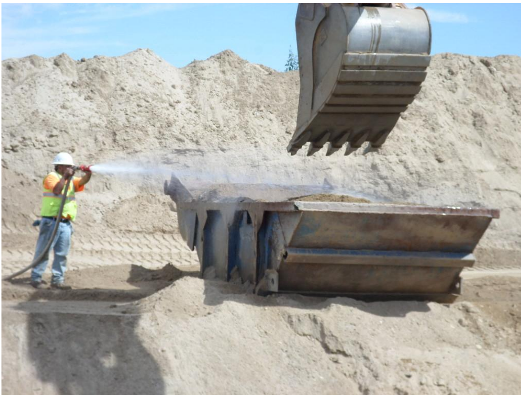
Sled D-KAL is using to separate pipe bedding and pipe zone sand from native material.
