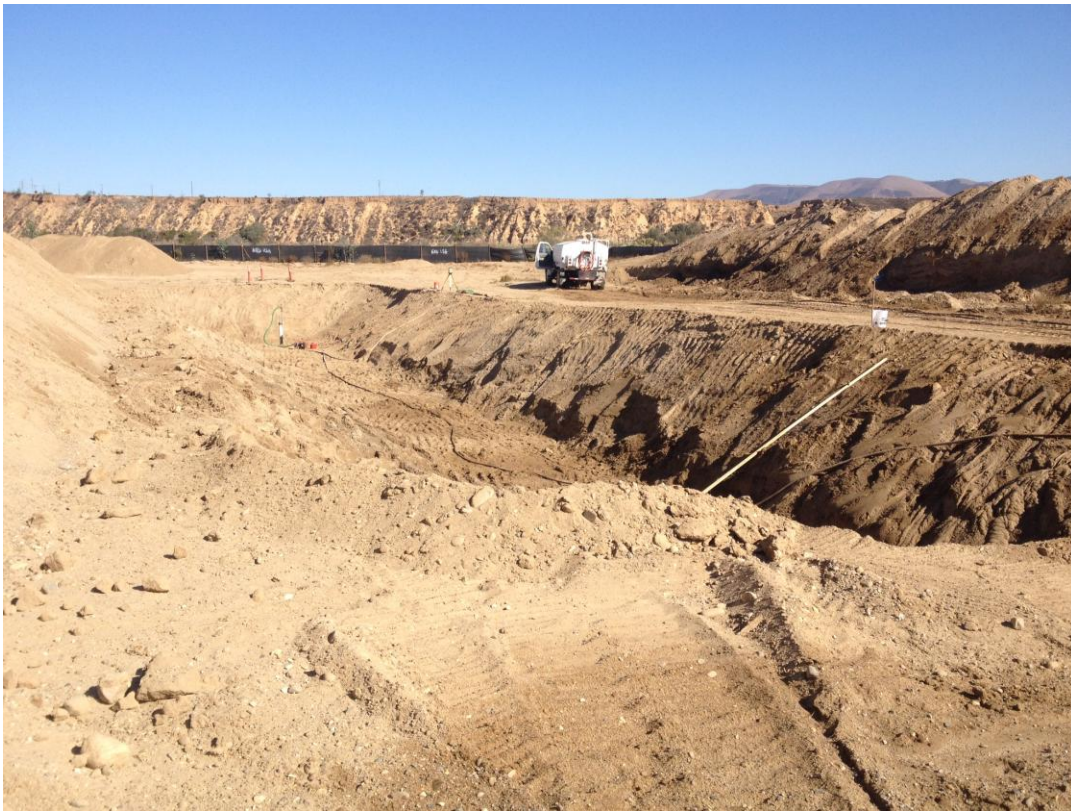
Riser at the end of the HDPE pipe exposed, D-KAL laying back slopes as they excavate.
