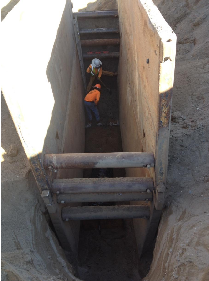
D-KAL backfilling over the 24-inch DI pipe and preparing for pouring the concrete encasement at the connection point.
