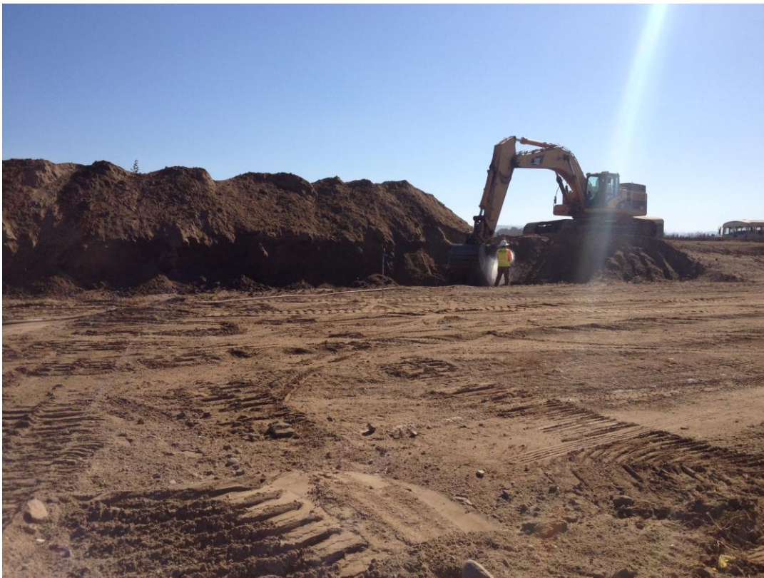
D-KAL preserving top soil by clearing from the trench area and stockpiling to the sides.
