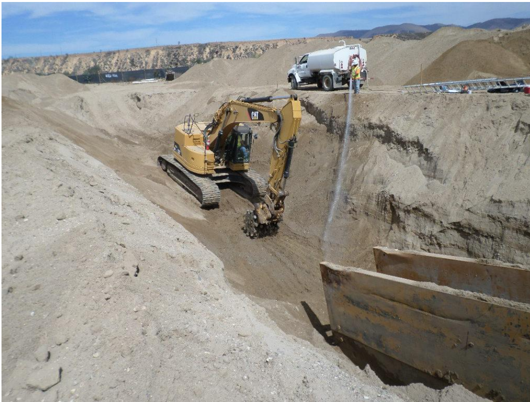
D-KAL moving trench shoring and backfilling and compacting over already installed pipe.
