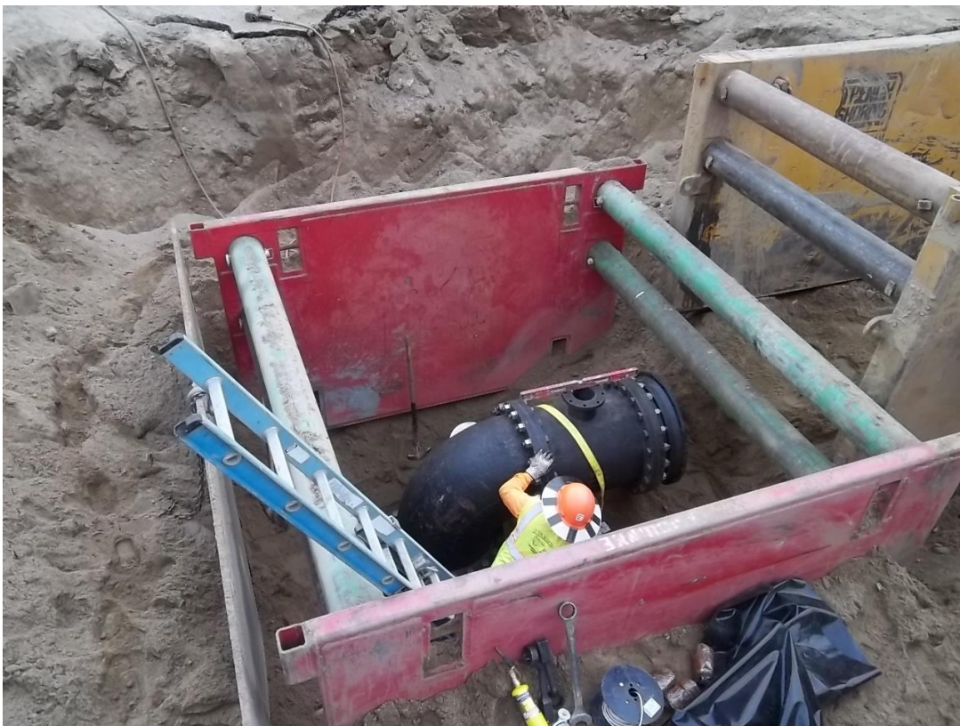
D-KAL successfully installing the 90 degree elbow to the 3 foot section of pipe which was installed due to the vertical pipe being out of round.
