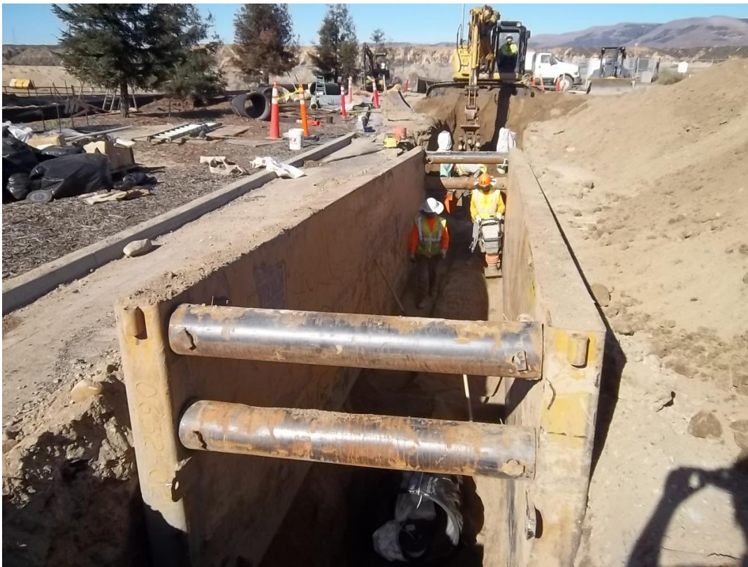
D-KAL installing 24-inch DIP in Blosser Road south of the receiving pit.
