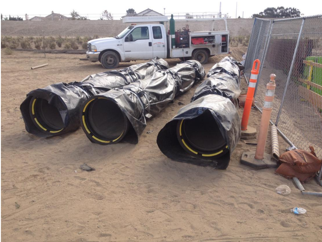
Ductile iron pipe wrapped in plastic with spacers installed, and ready for pushing through casing.
