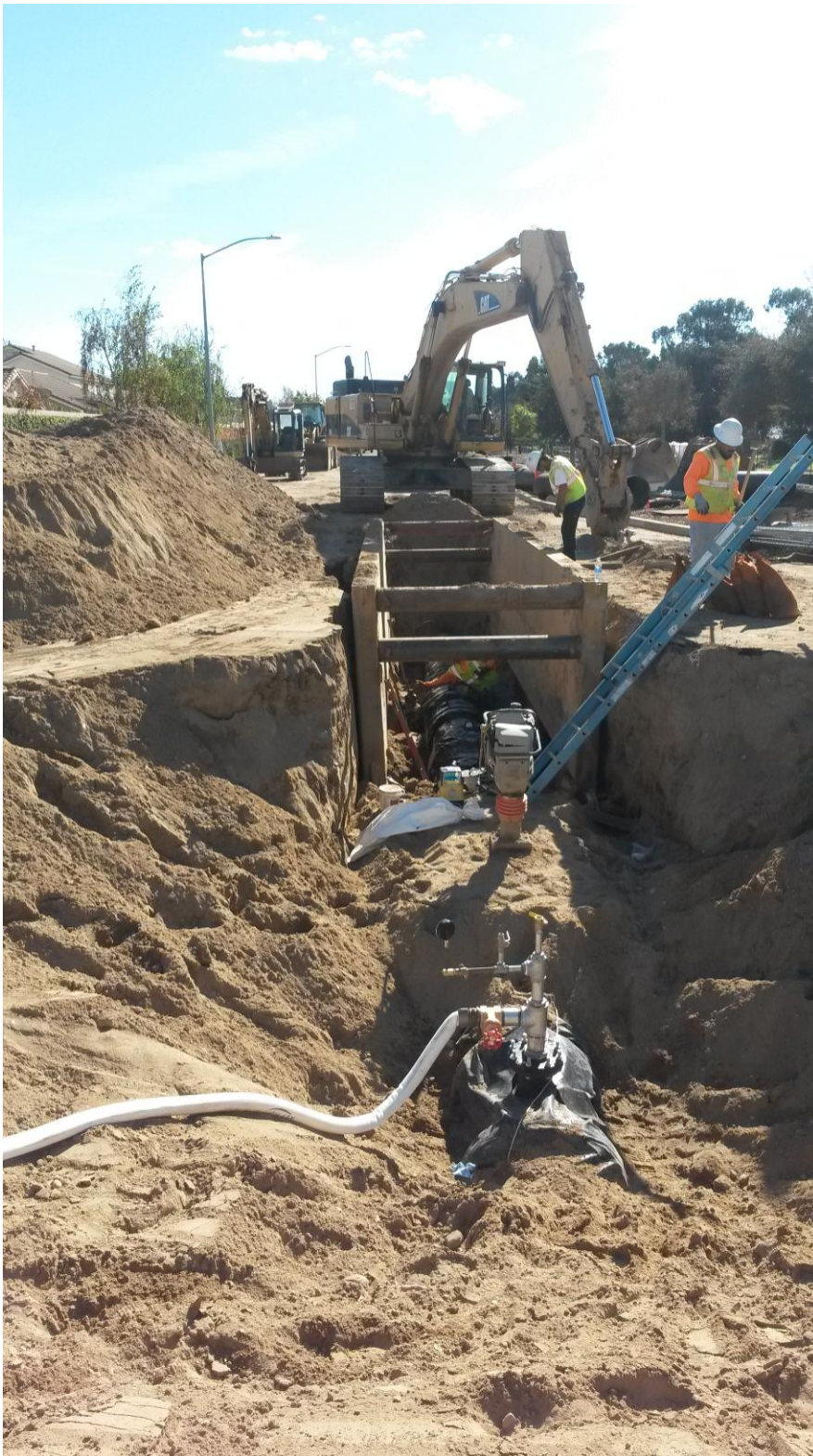
D-KAL installing pipe in Blosser Road and preparing to pressure test the section from the receiving pit to the BP #4 site.
