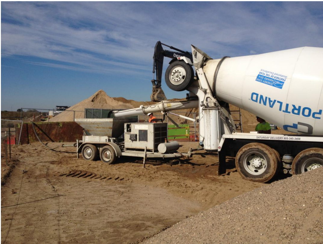
Filling grout pump and hopper for grouting the casing under the levee.
