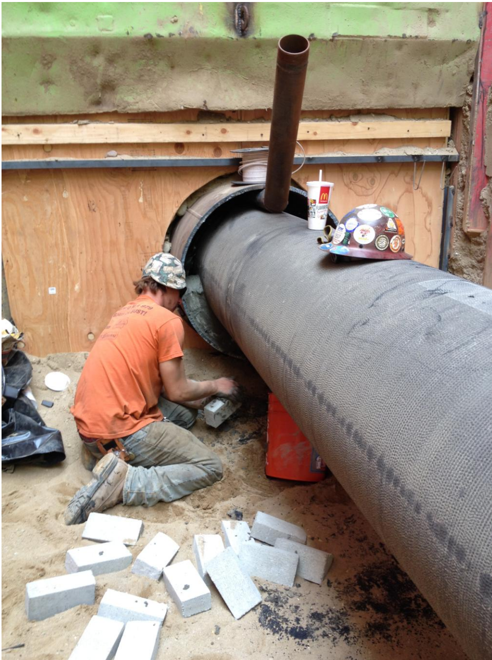
Pacific Boring installing bulkhead after pushing the 24-inch DIP into the casing.
