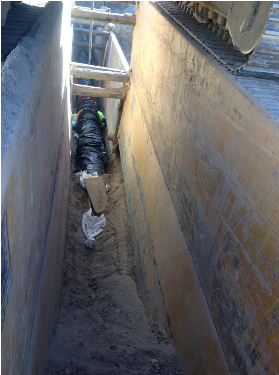
D-KAL connecting the deep trench section of 24-inch DIP to the section installed under the levee.
