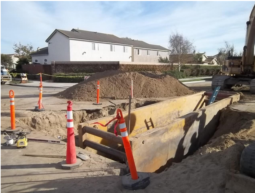
Trench shoring installed at the top of the receiving pit excavation to install the 90 degree bend onto the vertical segment of pipe.
