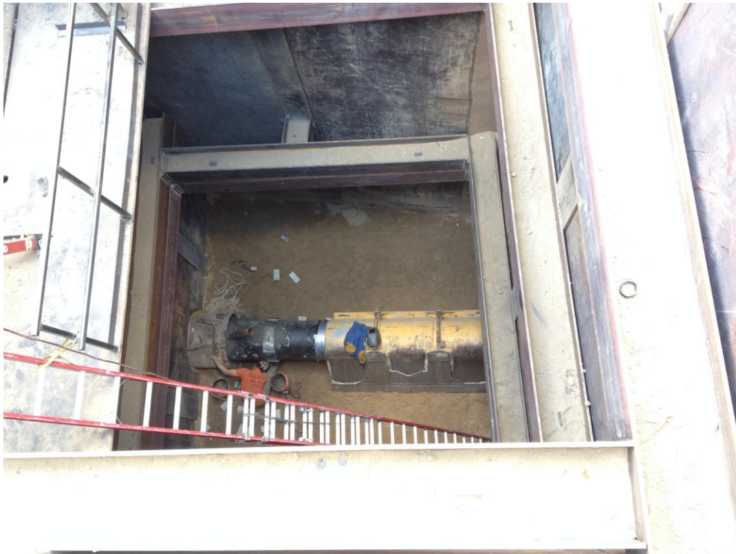
D-KAL placing bulkhead at the receiving end of the 36-inch steel casing in preparation for pressure grouting the casing.
