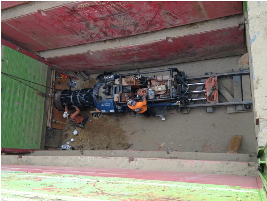
Pacific Boring completing pushing of one segment of 24-inch DIP into casing under levee.
