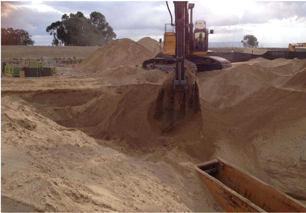
D-KAL completing the last 100 feet of 24-inch DIP installation to connect to the bore and jack section.
