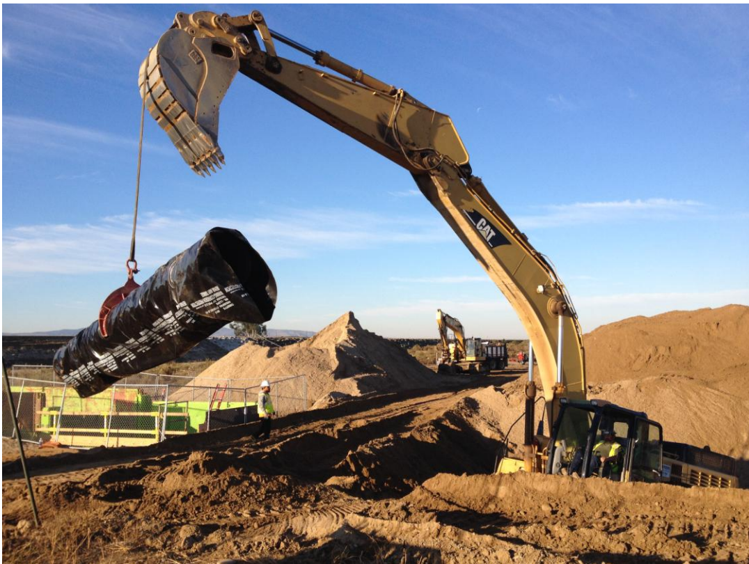
Installing 24-inch DIP in final segment of pipe in the river area.
