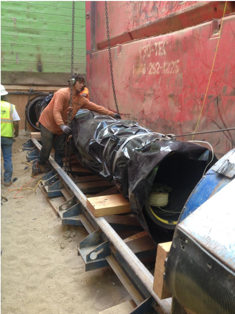
Pacific Boring positioning 24-inch DIP for pushing through the casing under the levee.
