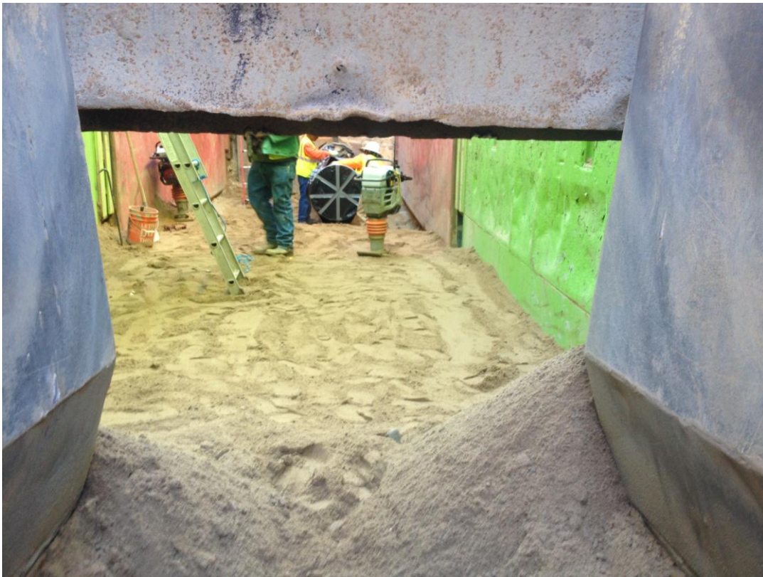
Opening in shoring for 24-inch DIP under the levee to connect to deep trench section.
