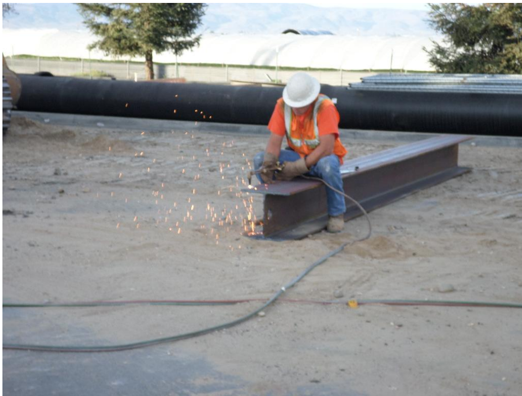
D-KAL cutting I beams to fit into final whaler support system in receiving pit.
