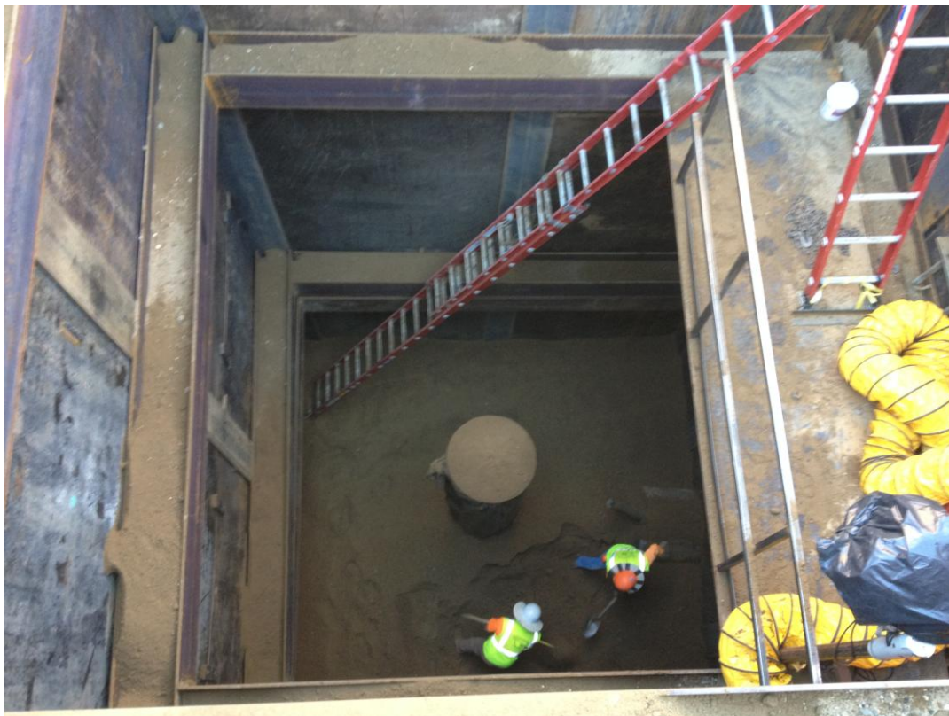
Vertical section of the 24-inch DIP being installed as D-KAL backfills receiving pit and removes shoring.
