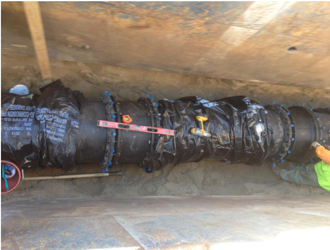
Connection of the deep trench pipe to the section installed by bore and jack under the levee, completing the pipe installation in the river area.
