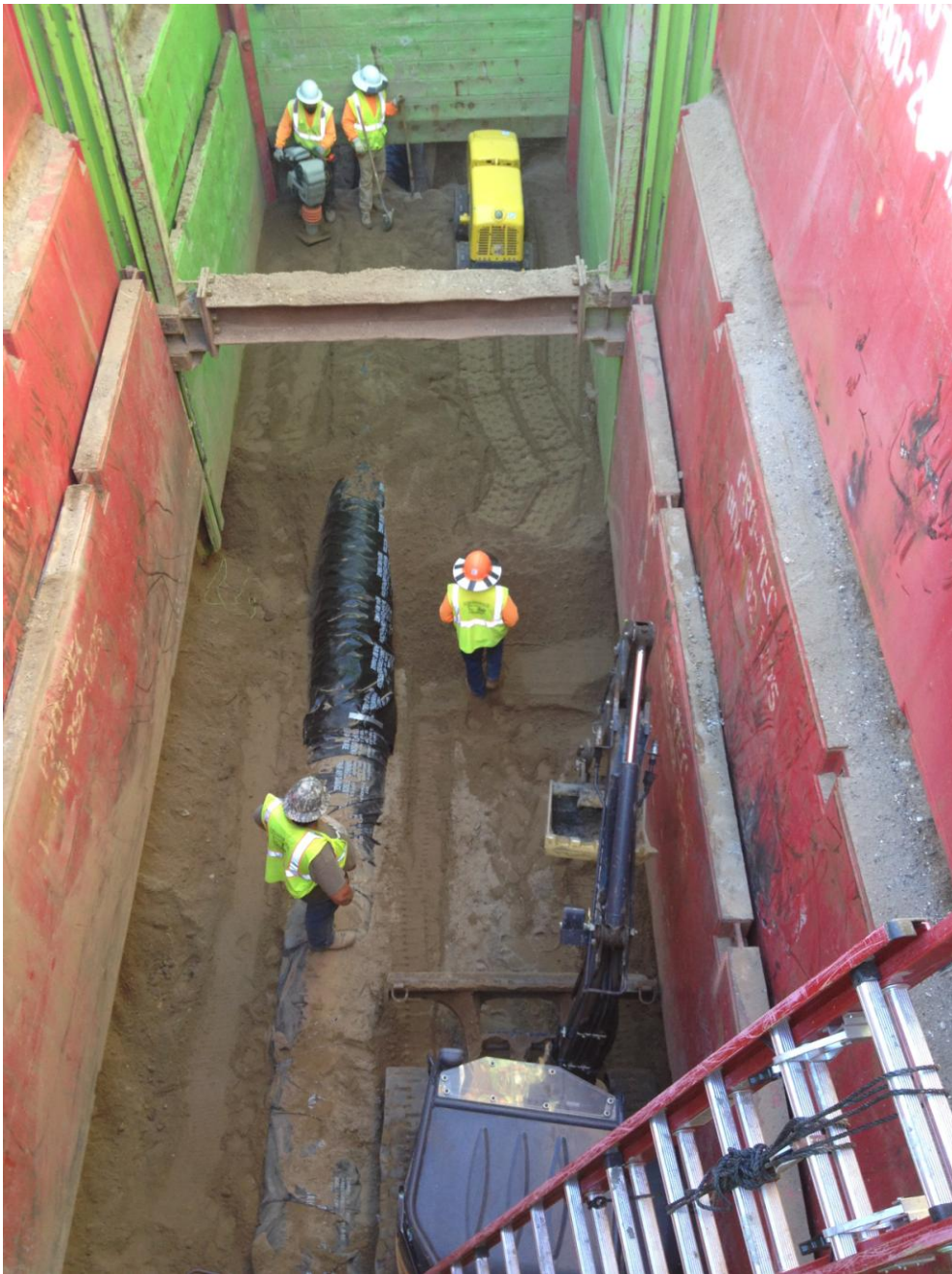
D-KAL compacting with whackers and using the remote control compactor to backfill around 24-inch DIP segment inside the bore and jack pit.
