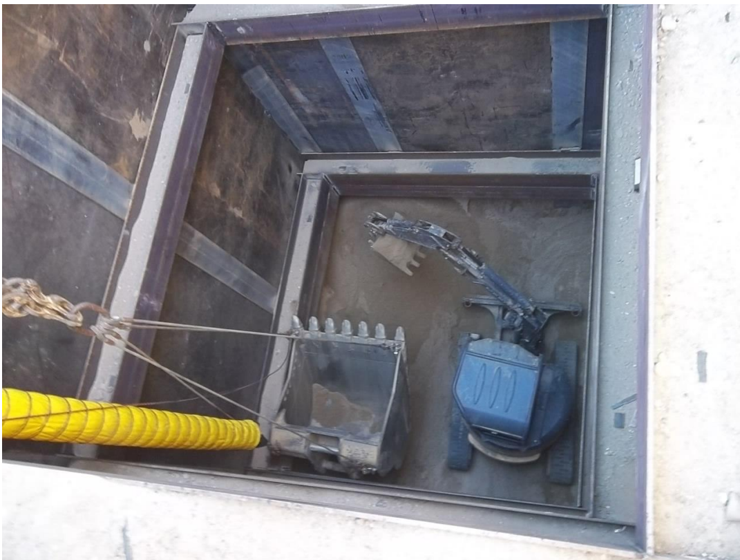
D-KAL using modified clam shell bucket and mini excavator inside receiving pit to excavate material down to final grade.
