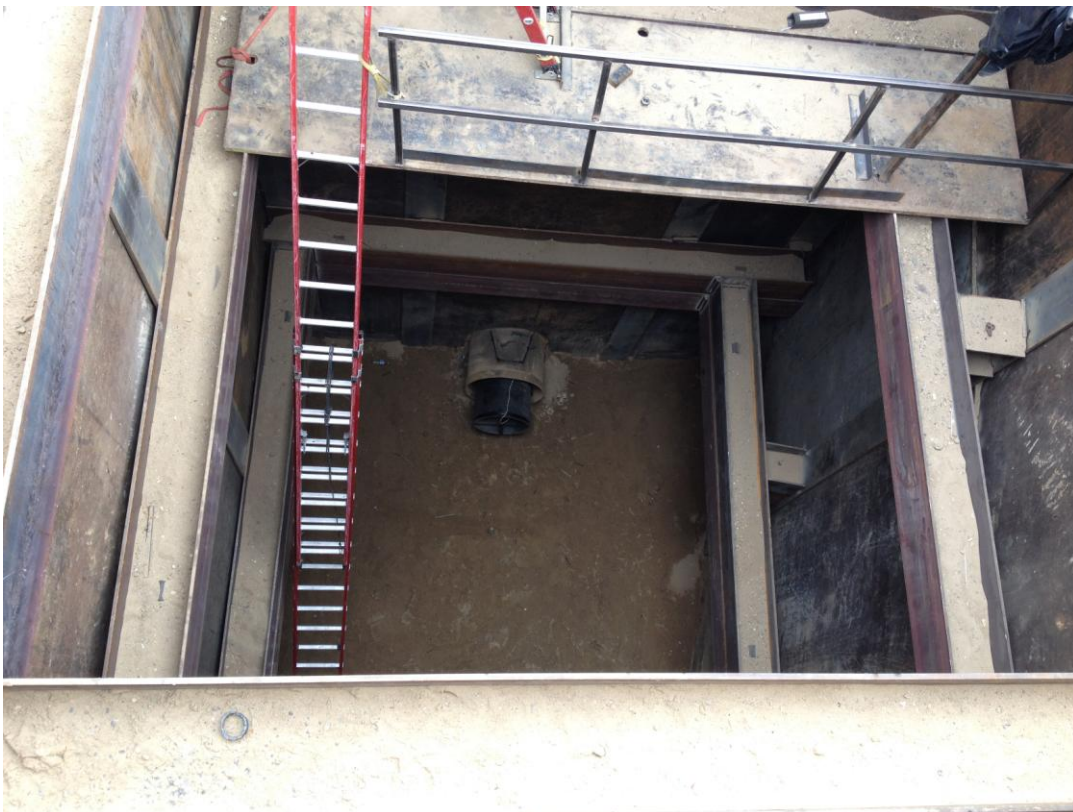
24-inch DIP received after being pushed through the casing under the levee.
