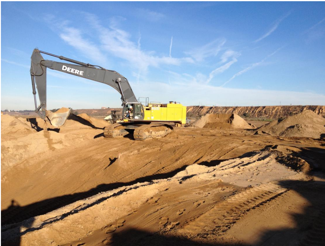
D-KAL backfilling over final segment of the 24-inch DIP in the river area.
