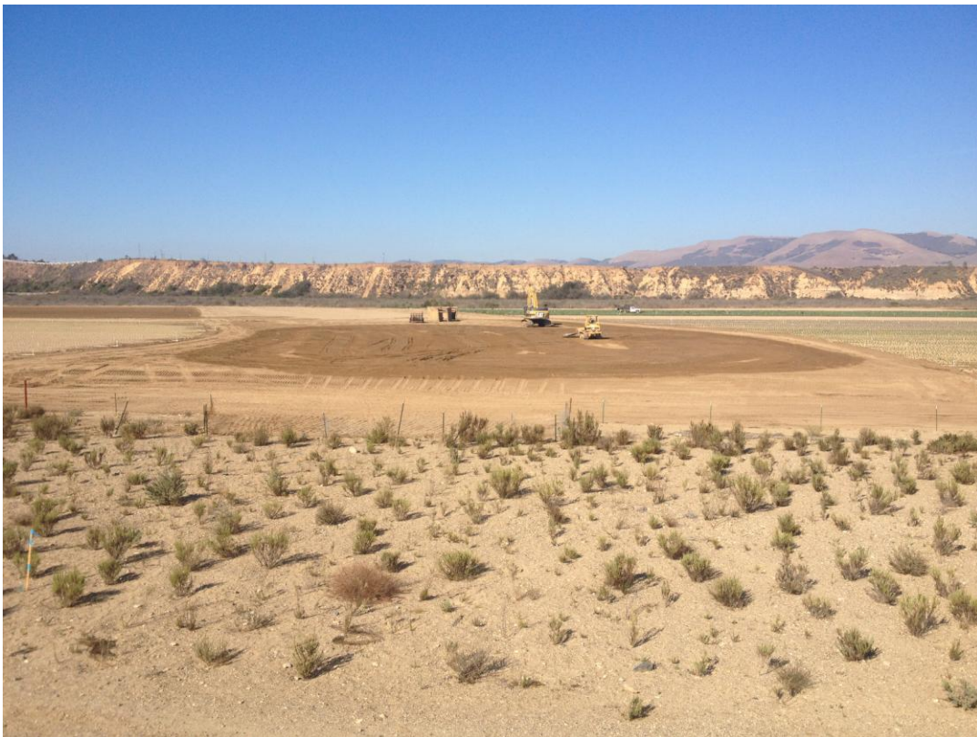
Final restoration of agricultural topsoil and farm access road in river area.
