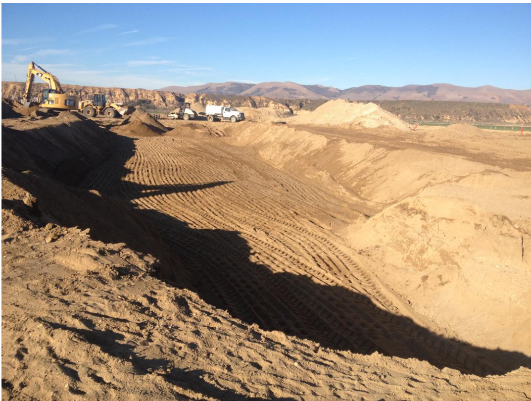
Backfilling over the final segment of pipe installation and restoration of agricultural topsoil.
