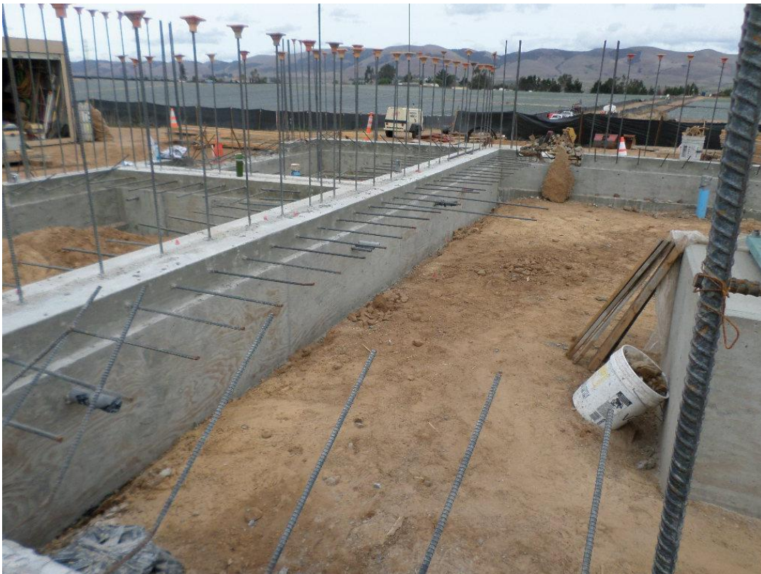
Forms being stripped from the stem wall pour at the pump station.
