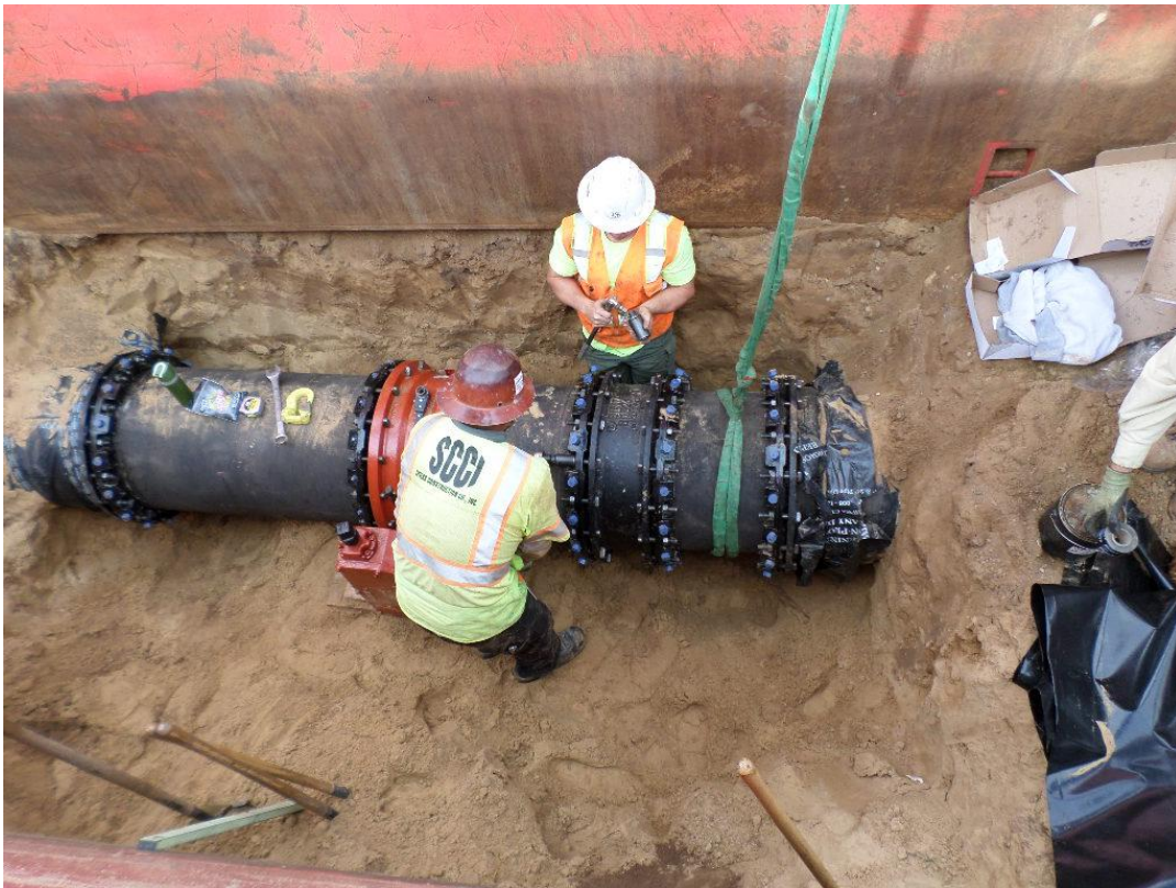
Spieß installing 24-inch valve at the bypass in Santa Maria Vista Way.
