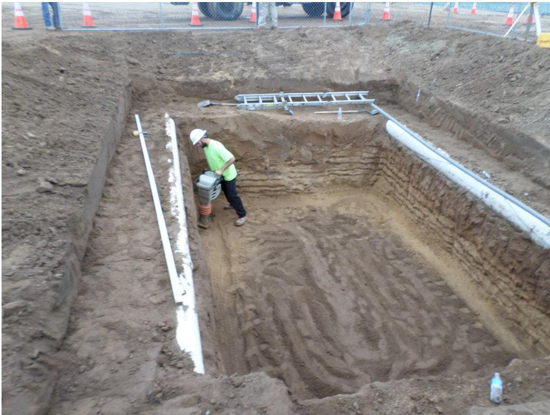
Spiess compacting subgrade for the PRV vault in Santa Maria Vista Way.
