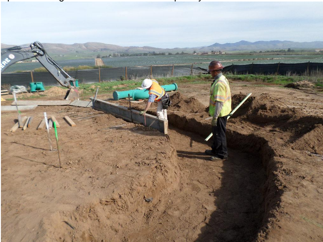
Excavation completed for the concrete spillway and Spieß starting on form construction.
