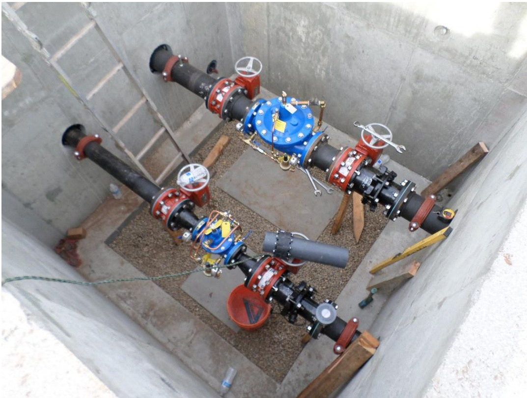
Piping installed inside PRV vault.
