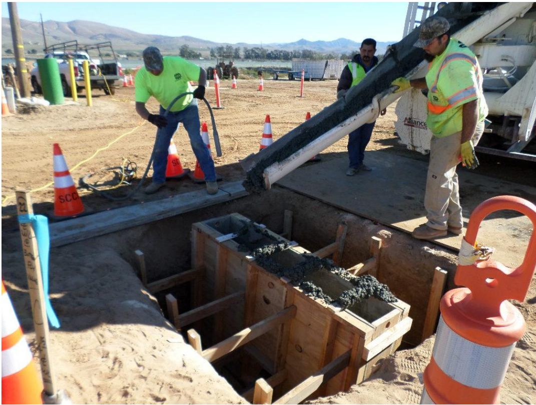
Spieß pouring one of the thrust collars on the 12-inch water line in Santa Maria Vista Way.
