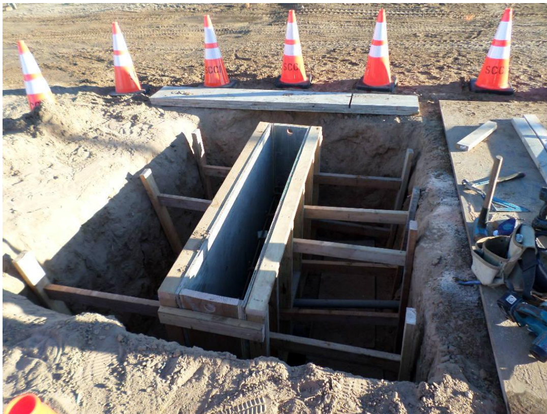
Thrust collar formed for 12-inch PVC water line in Santa Maria Vista Way.
