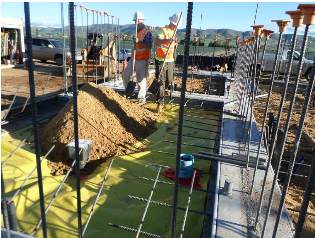
Spiess spreading sand over vapor barrier for slab at ammonium sulfate room.
