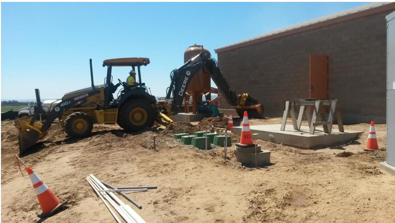
Spies removing native material to prepare site for aggregate base installation for driveway.
