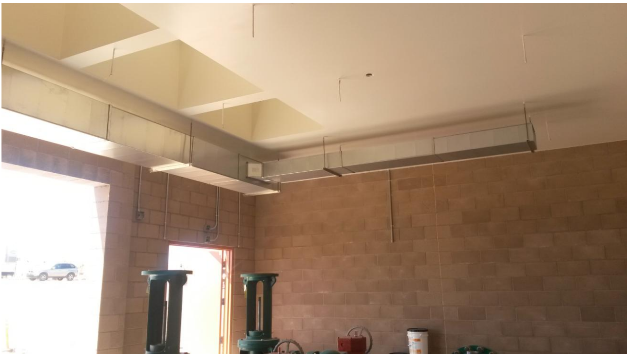
HVAC ducts installed in pump room.
