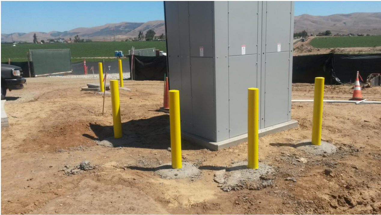
Bollards coated at PG&E electrical control panel.
