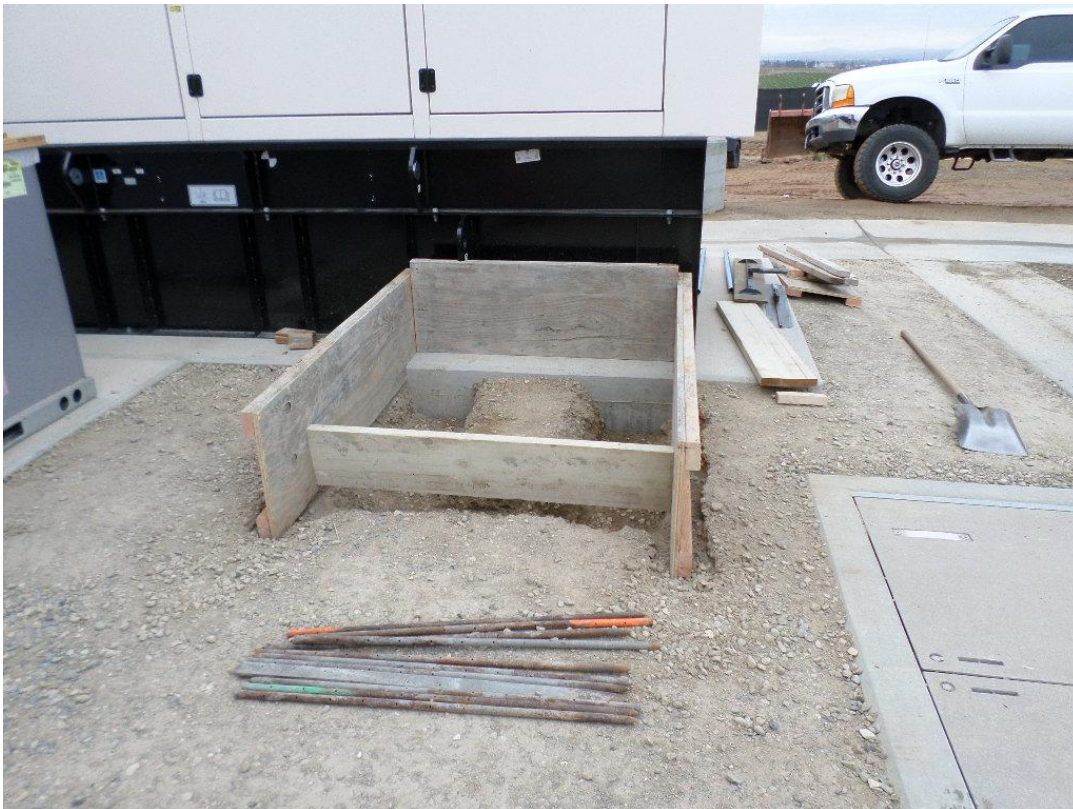
Spies forming steps to access emergency generator.
