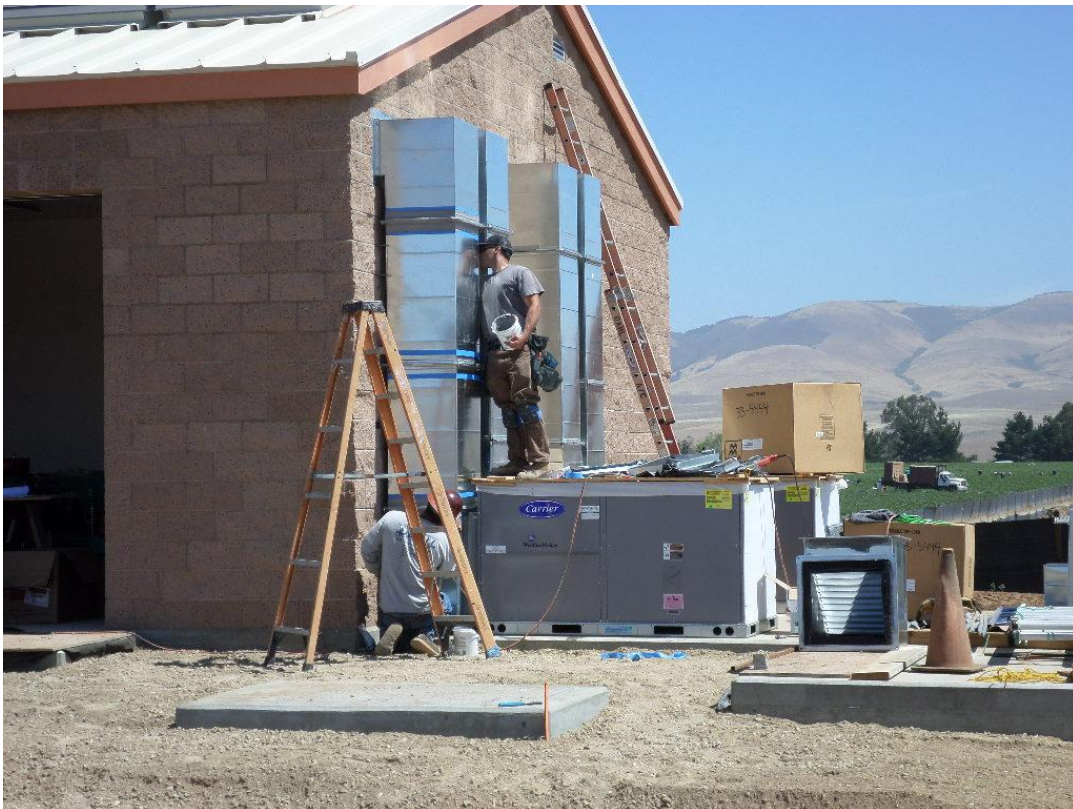
Exterior HVAC ducts installed.
