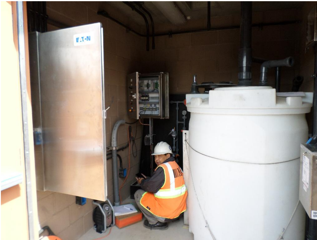
Hopkins testing chemical feed pump.
