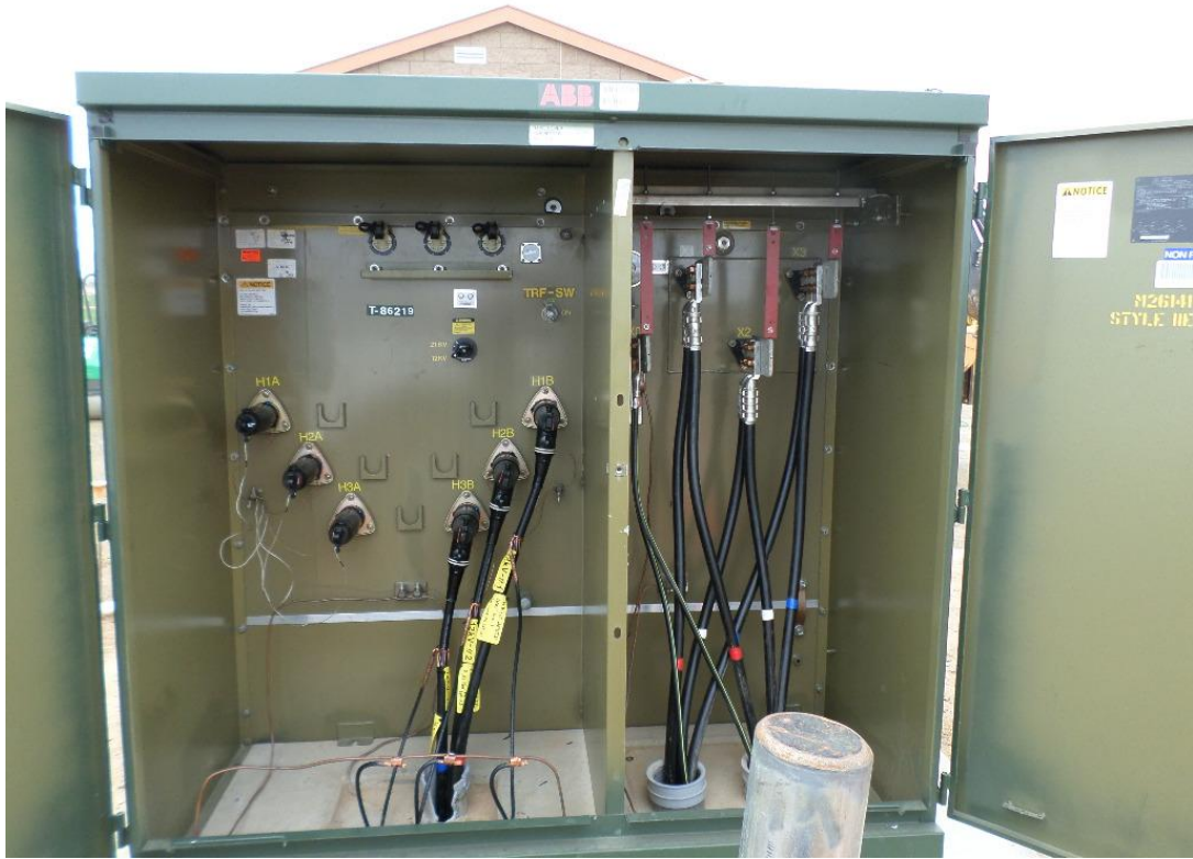
Electrical service terminated by PG&E at transformer.
