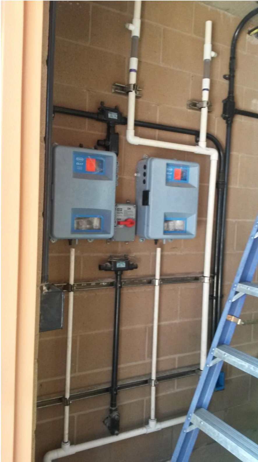
Chlorine analyzers installed.
