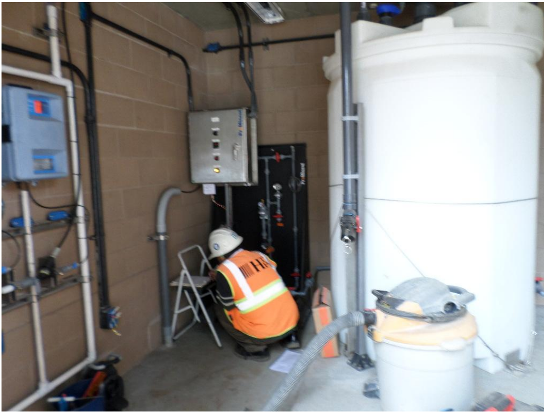
Testing chemical pumps.
