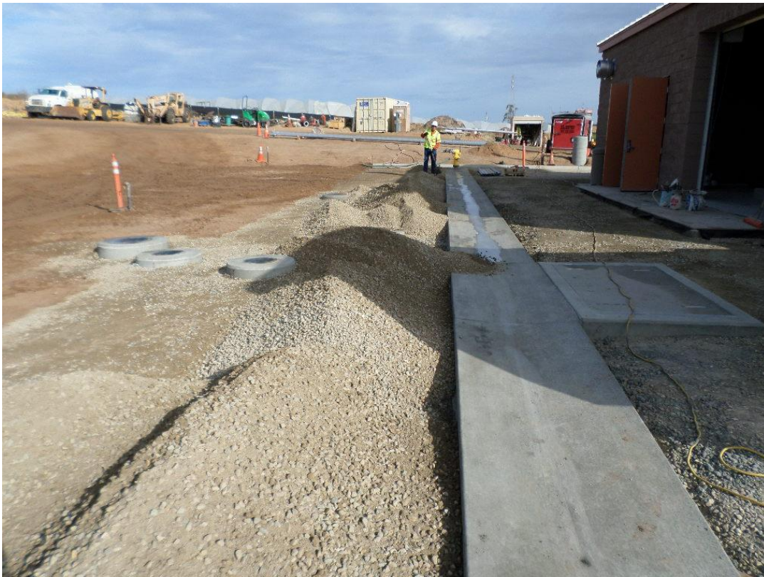
Spieess placing aggregate base around valve cans and V-ditch for finish grade.
