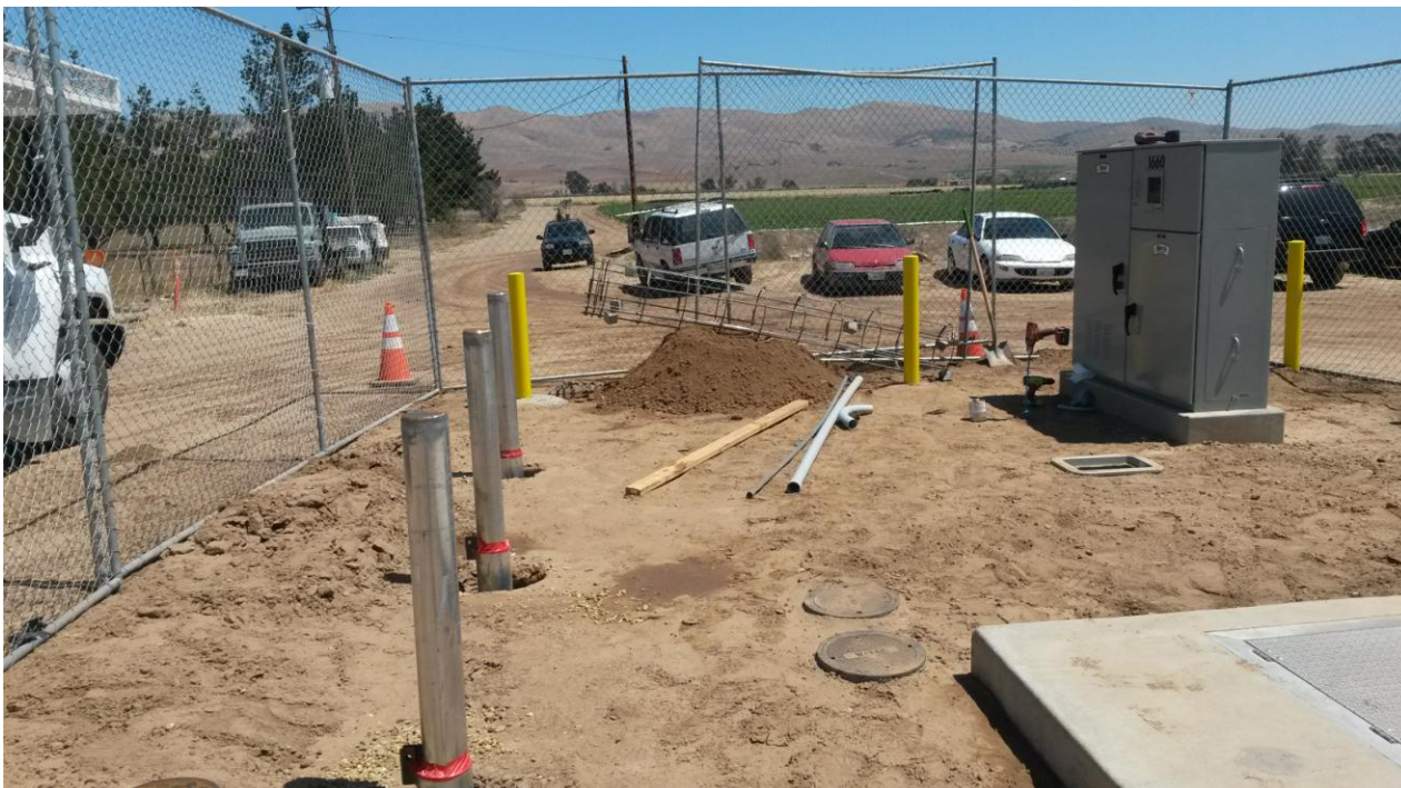
St. Denis Electric drilling for the SCADA antenna base at the PRV vault.
