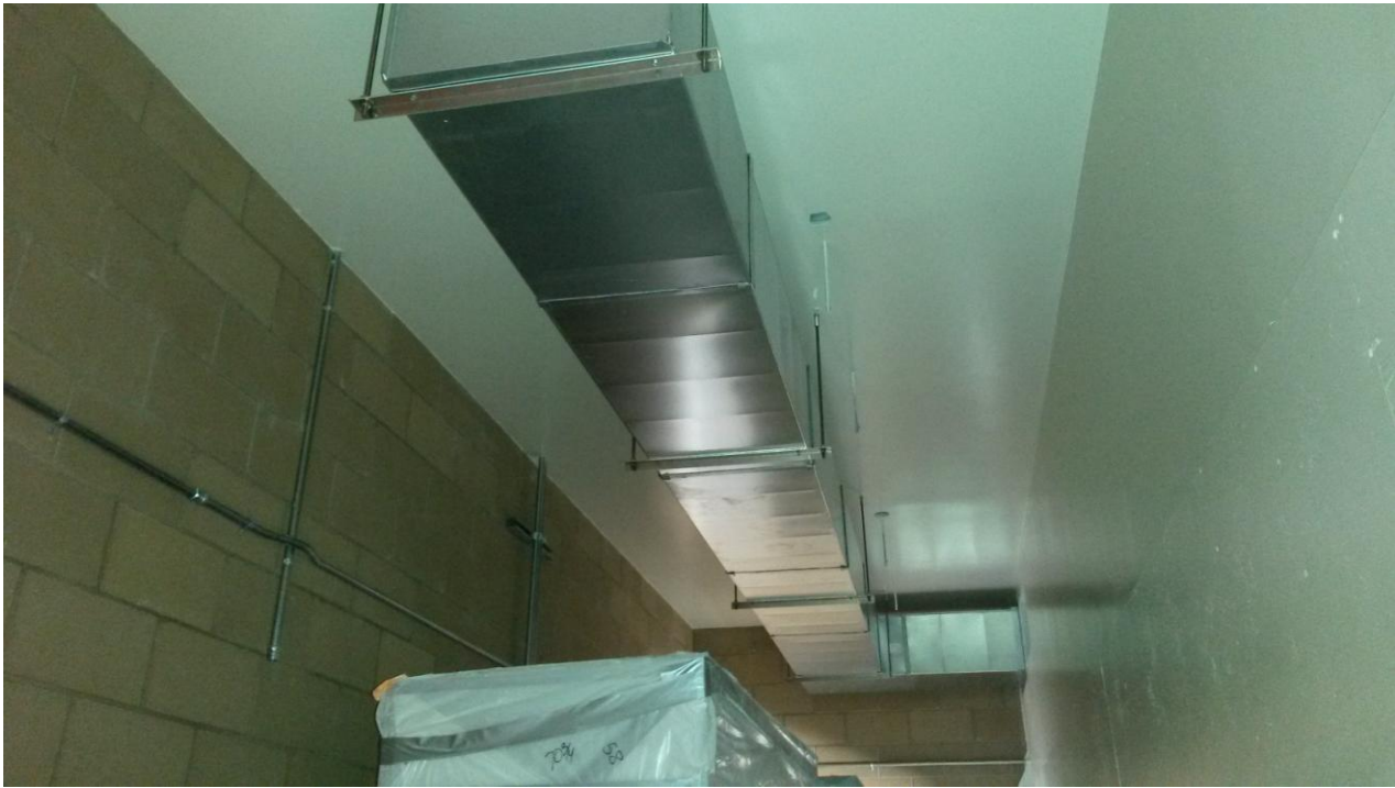
HVAC ducts installed in electrical room.
