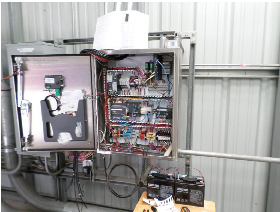
PLC panel and wiring.
