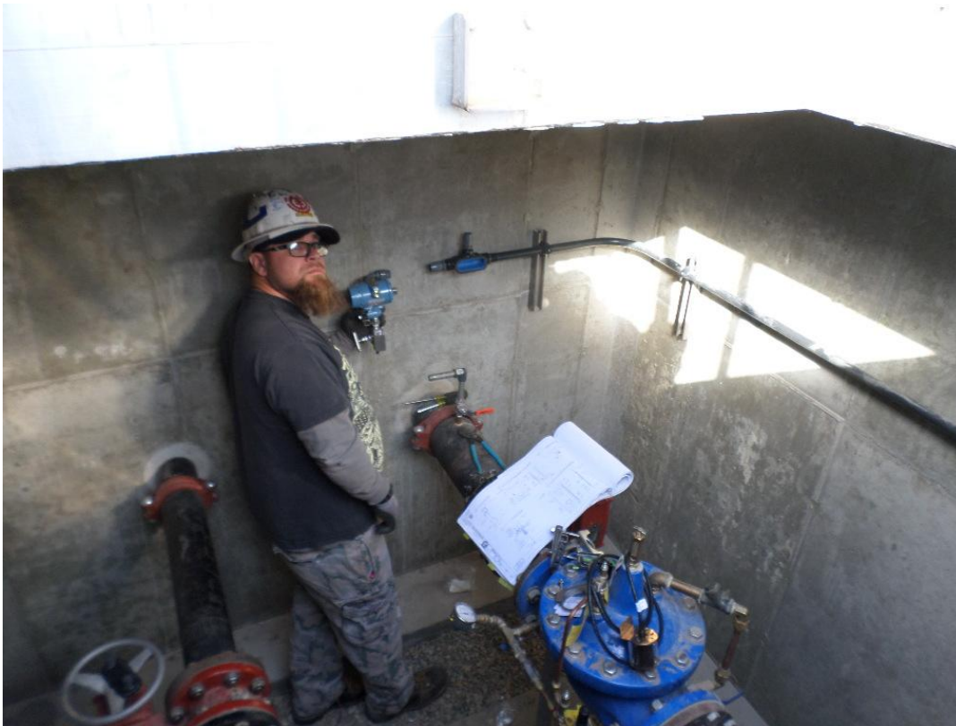
St. Denis Electric installing the pressure transmitter and conduit in the PRV vault.
