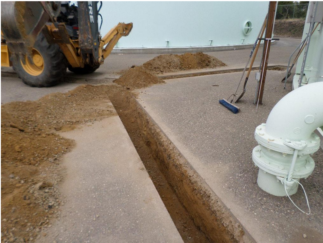
Spiess excavating trench to prepare for installation of drain line and conduits at the Quad Tanks.
