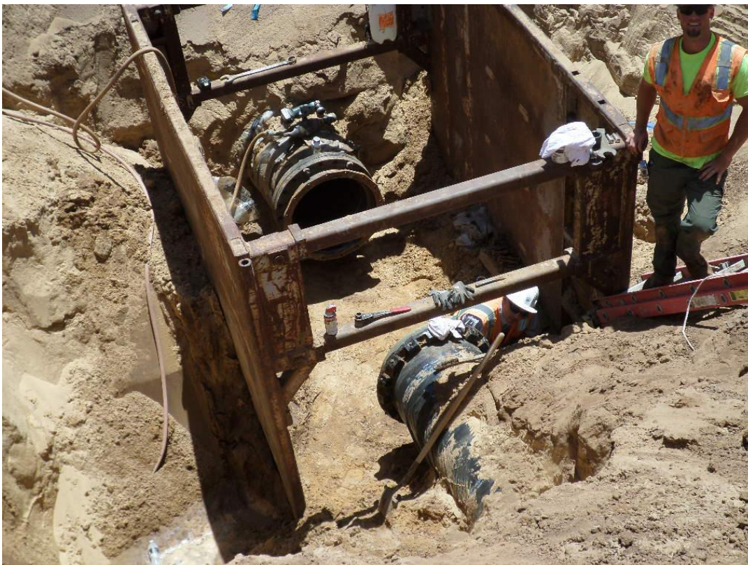
Spies preparing to connect the 24-inch DIP pipe from the pump station to the HDPE pipe from Bid Package #1.
