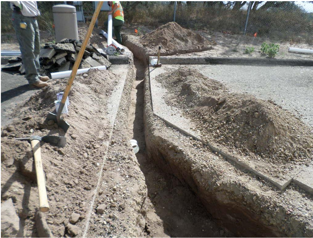
Spies excavating trench for the 4-inch drain line and conduit at the Standpipe Tank.
