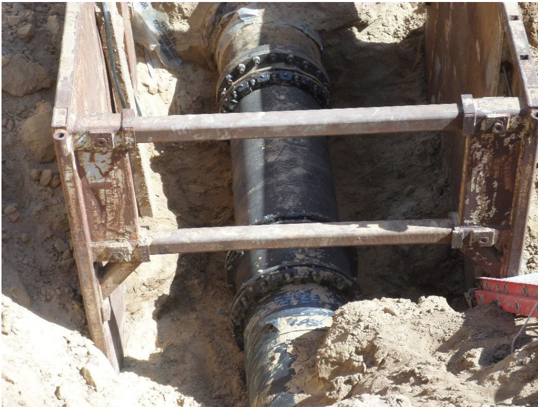
Connection of the 24-inch DIP to the HDPE pipe from Bid Package #1 completed.
