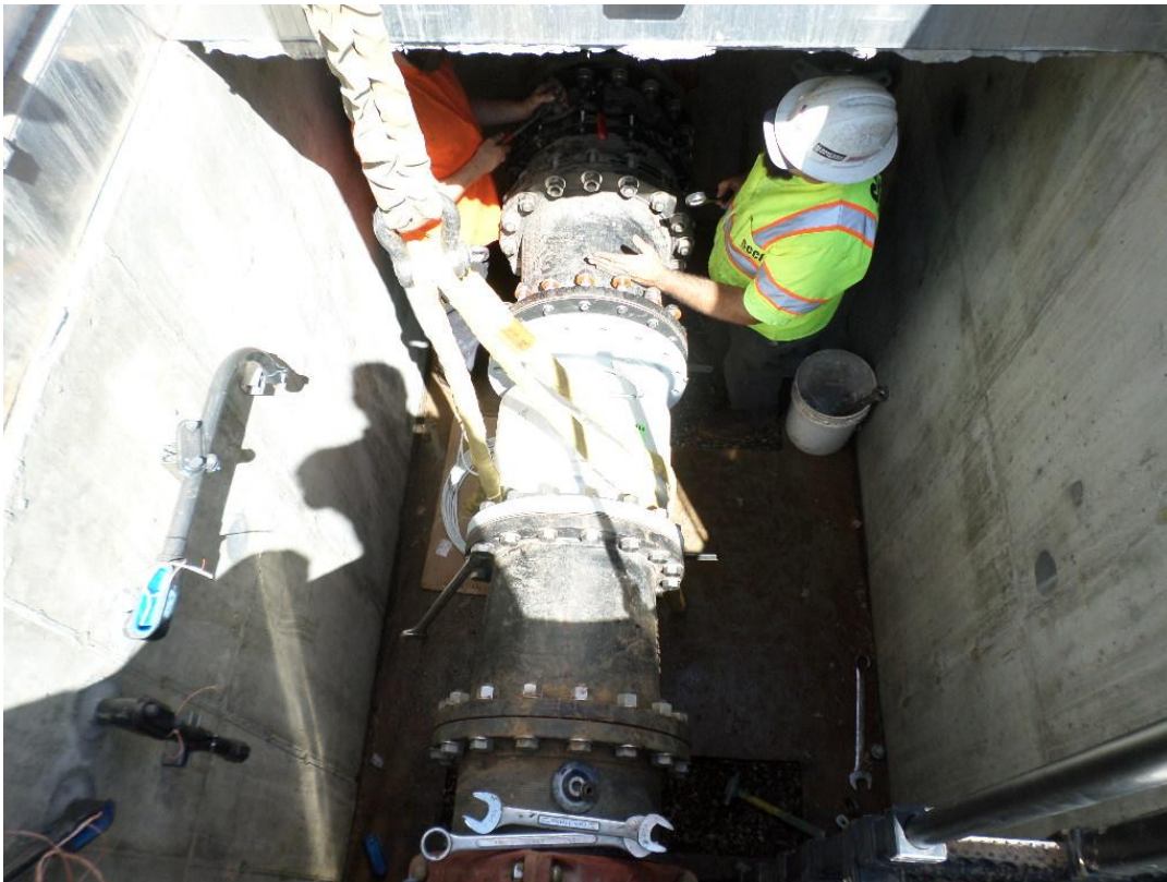
Flow meter installed in flow metering vault.
