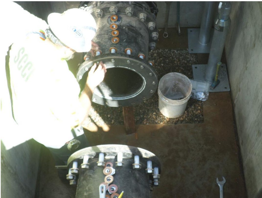
Spieß installing the flow meter in the flow meter vault at the pump station.
