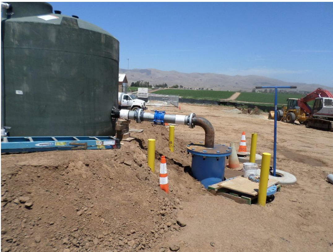
Temporary tank and piping for testing the pump station prior to taking water from the City of Santa Maria.
