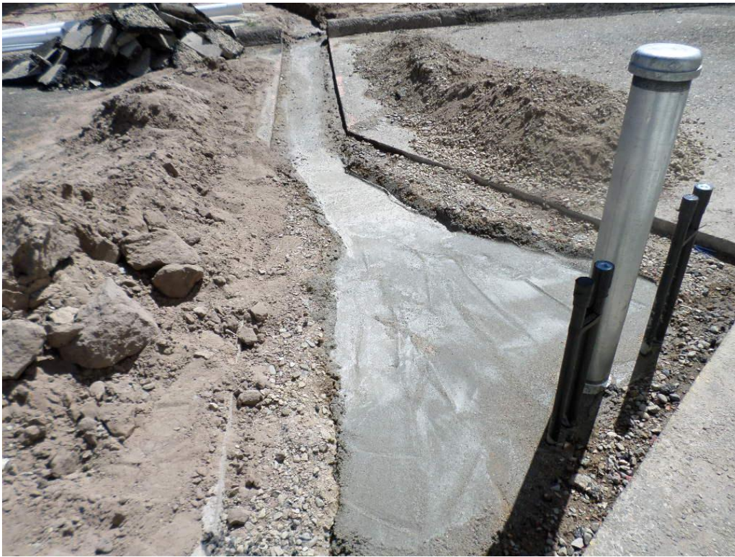
Slurry poured over the 4-inch drain line and conduits at the Standpipe Tank.
