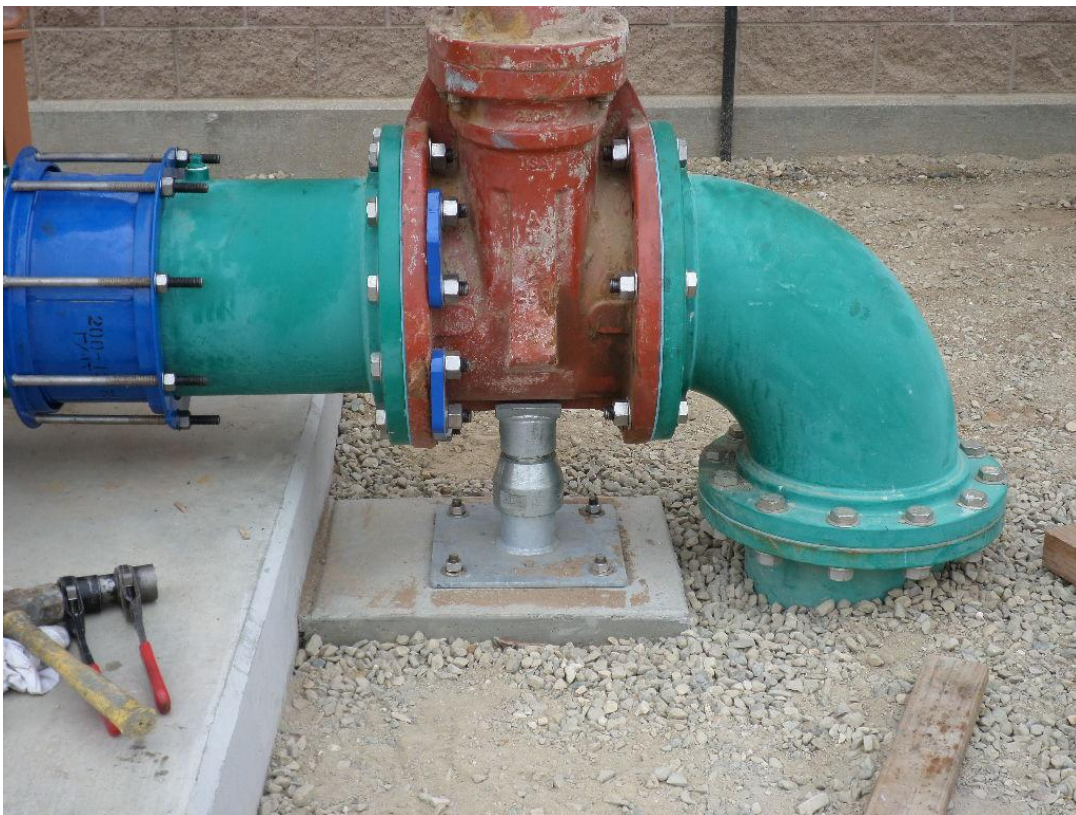
Pipe support installed under the valve at the surge tank.
