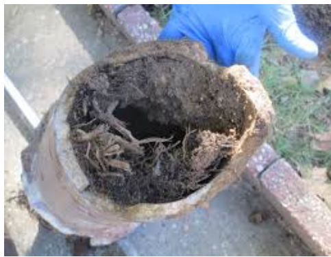
Sewer main destroyed by roots
