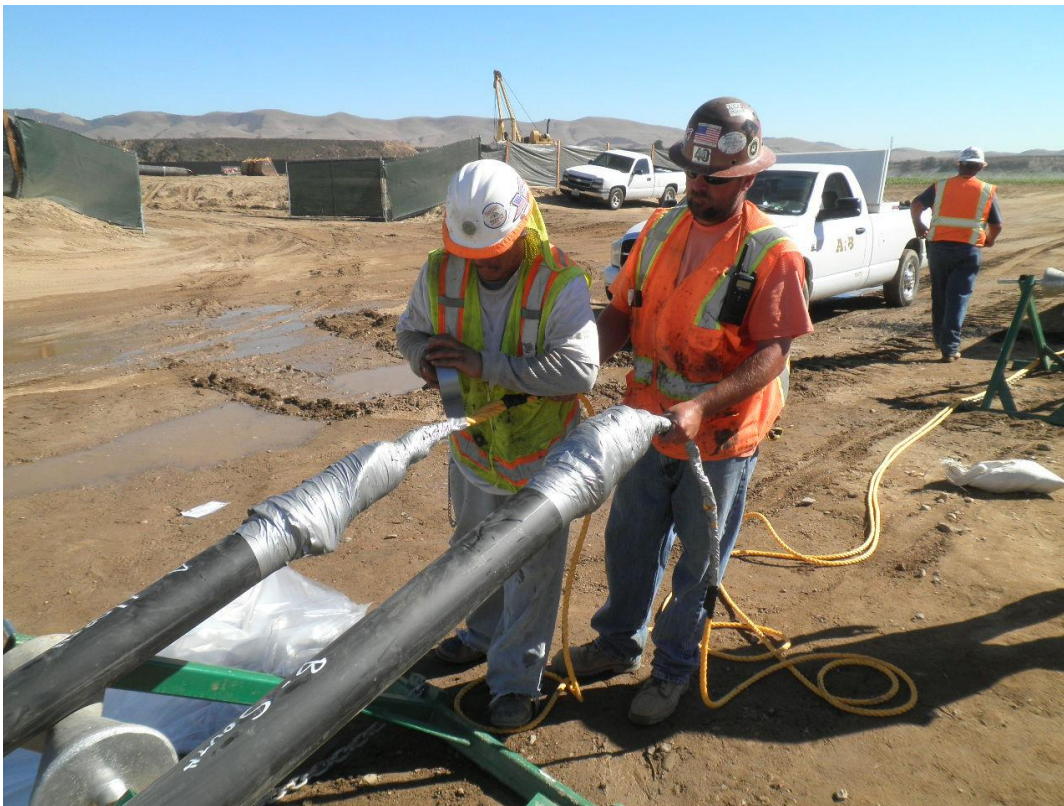
ARB attaching rope to the two 4-inch ballast and vent pipes in preparation for inserting them into the HDPE pipe.
