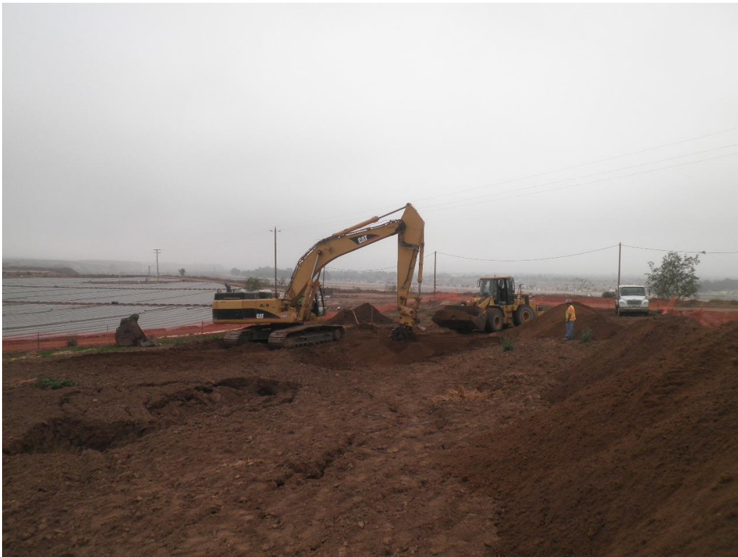
ARB backfilling sink holes with imported material in preparation for GeoGrout mobilization.
