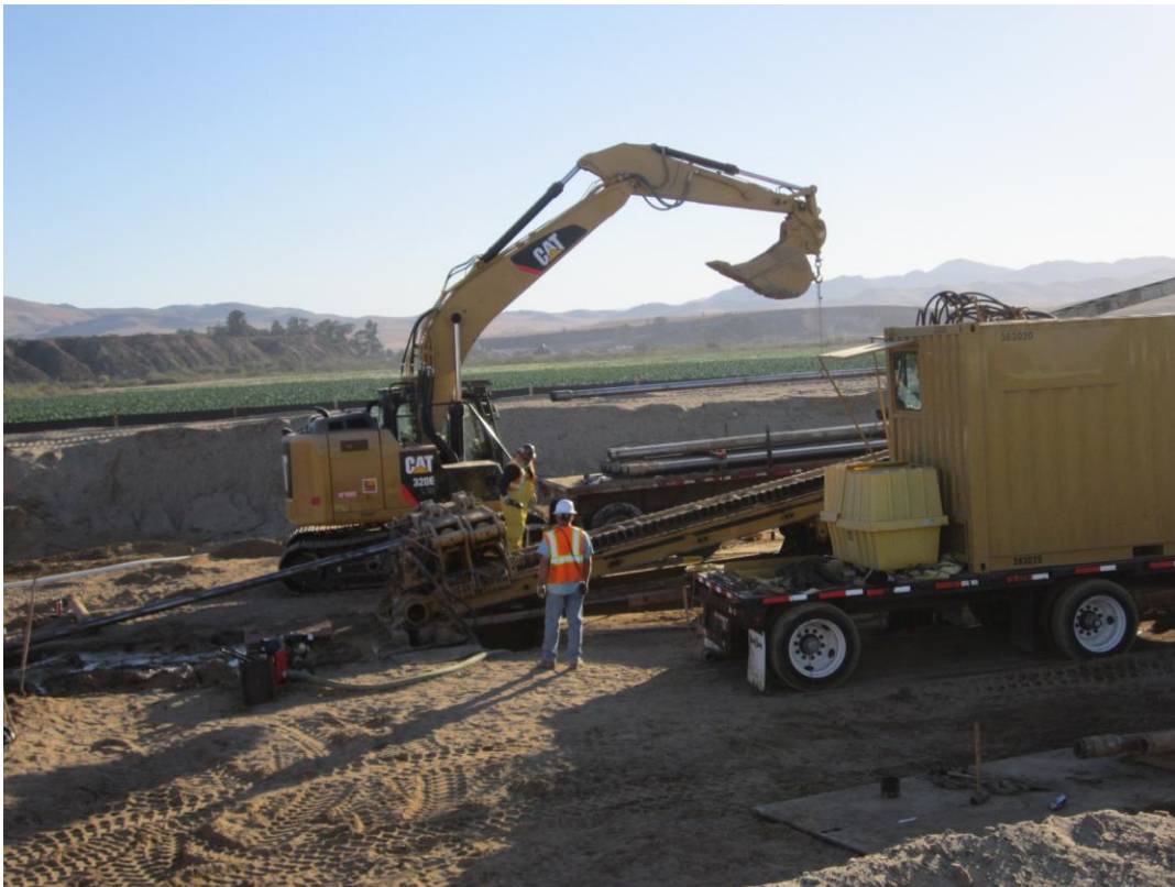
ARB removing pipe string after the second failure of the adapters on the 42-inch drill.
