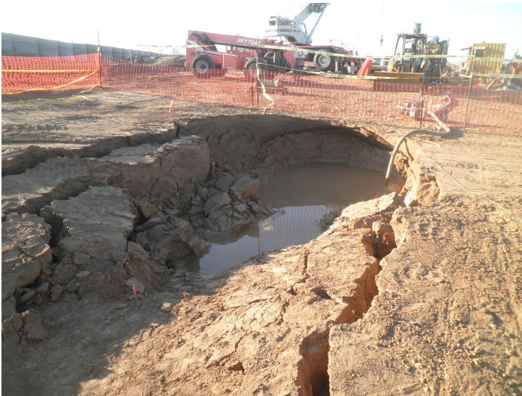
Mud rising in sink hole within the temporary construction easement area as ARB proceeds with the 42-inch ream on October 21.
