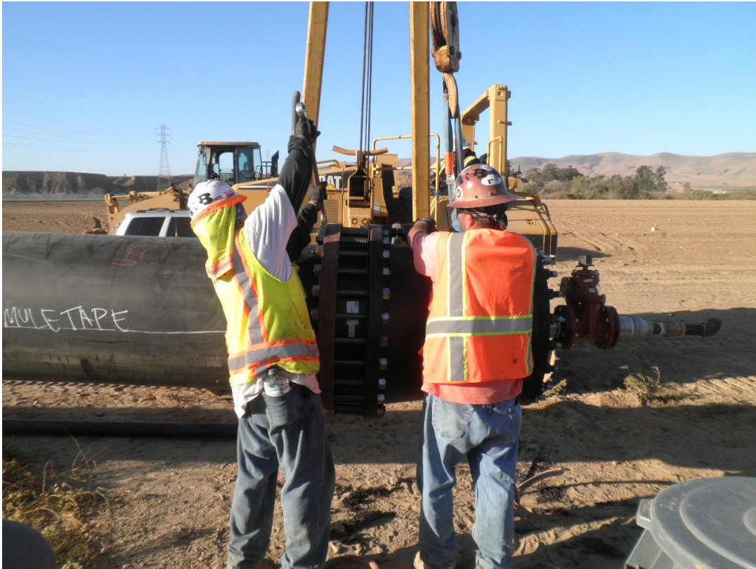
ARB bolting test fitting to the east end of the HDPE pipe.
