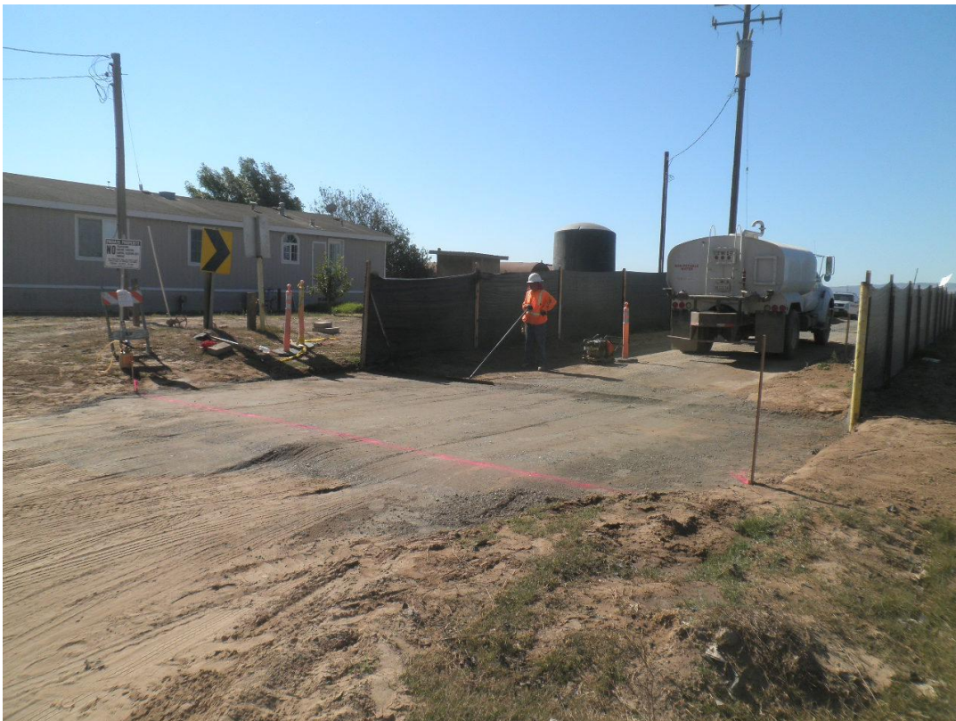
R. Burke Construction placing base for installation of a gate at the site entrance to prevent CRLF from entering the site.
