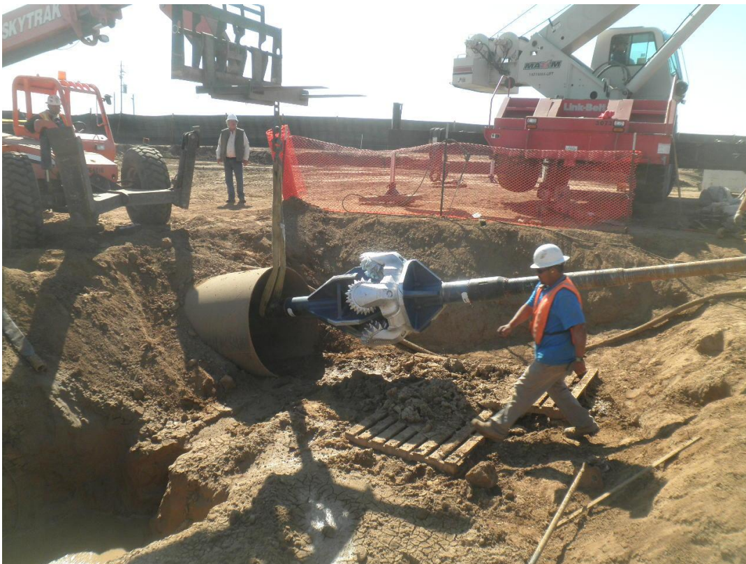
ARB inserting 42-inch drill for final attempt at completing the reaming from the north side on October 21.
