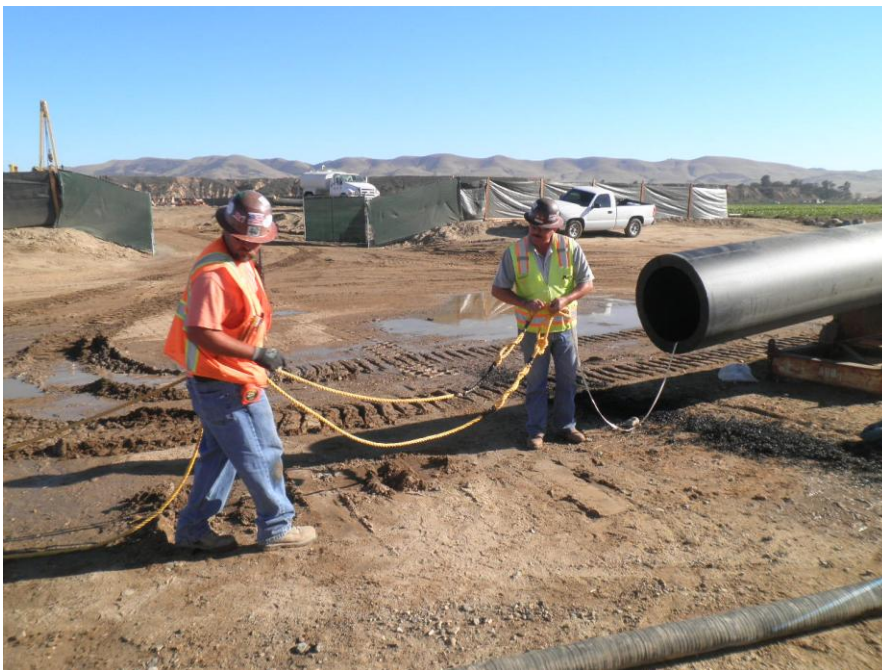
ARB using mule tape and rope to prepare for pulling of two 4-inch pipes (ballast and vent) into HDPE pipe.
