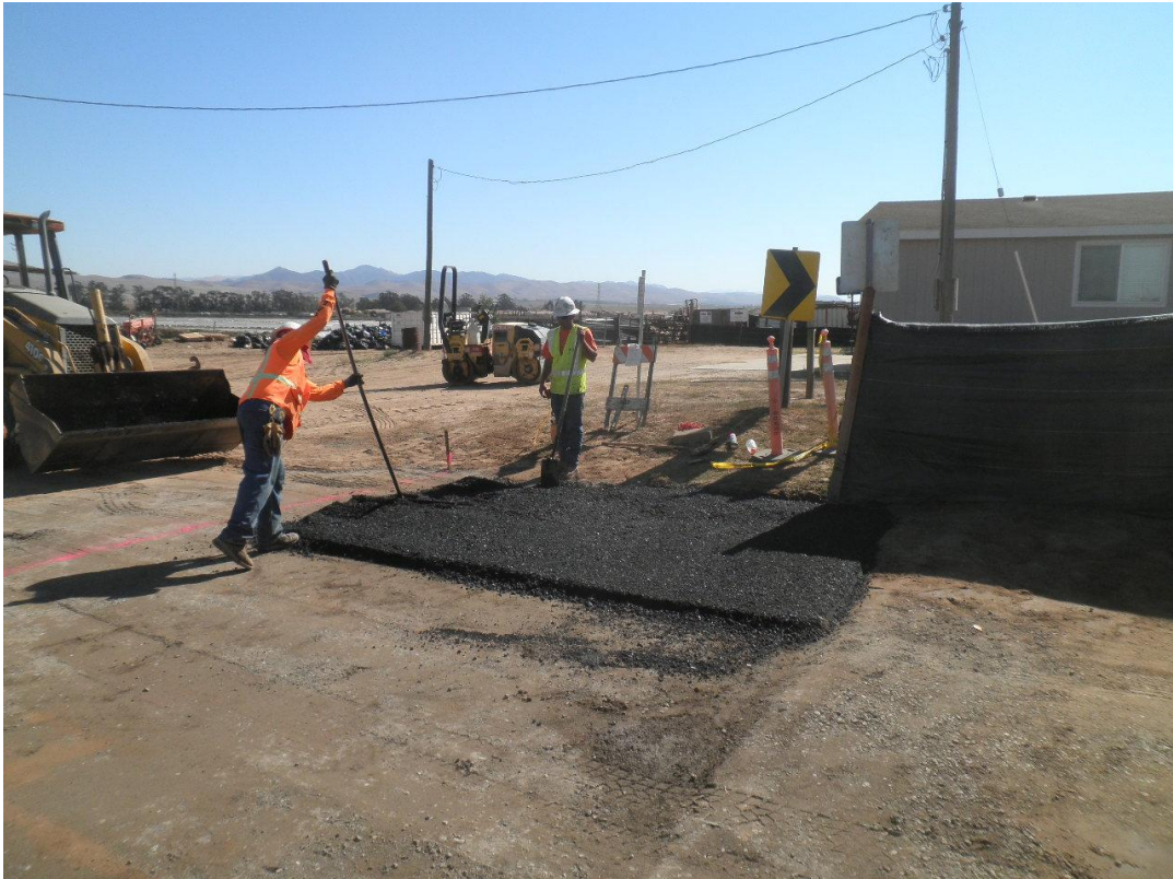
R. Burke Construction placing an AC apron under the gate to prevent CRLFs from entering the site.
