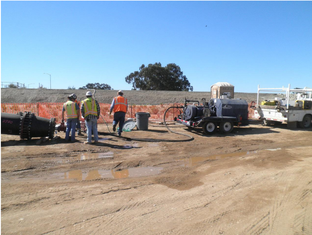
New pump brought in by ARB to reach hydrostatic test pressure of 152.5 psi.
