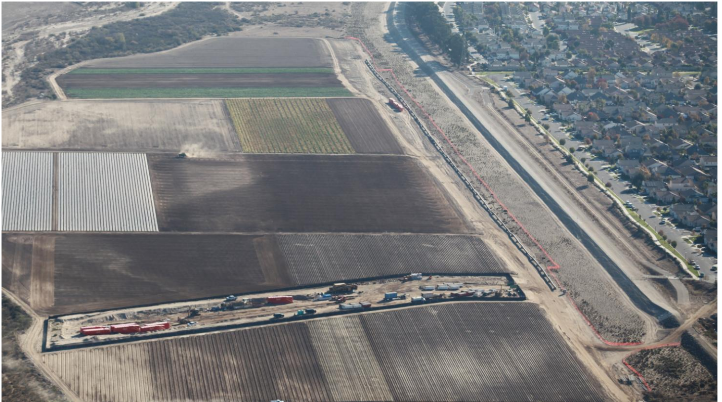
Aerial photo of the south side with ARB's equipment and the HDPE pipe fused and laid out to the east.
