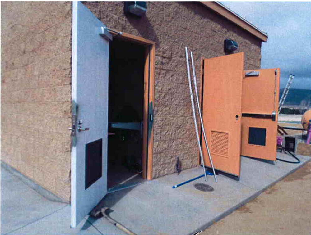
J & J Door installing door hardware at the Sodium Hypochlorite Storage Building.
