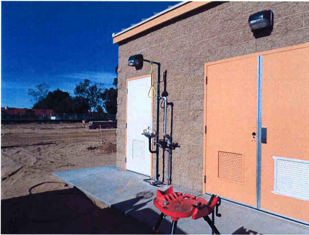
Eyewash station installed at the Sodium Hypochlorite Storage Building.
