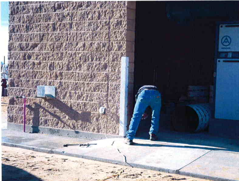
Cushman installing corner guards at the roll-up door in the Electrical/Blower Building.
