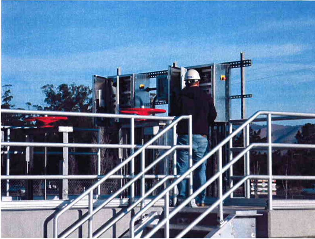
Westech on site trouble shooting at the panel for the headworks.
