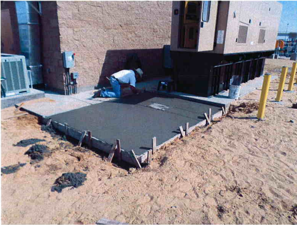
Cushman pouring slab for the aluminum stair landing at the emergency generator.
