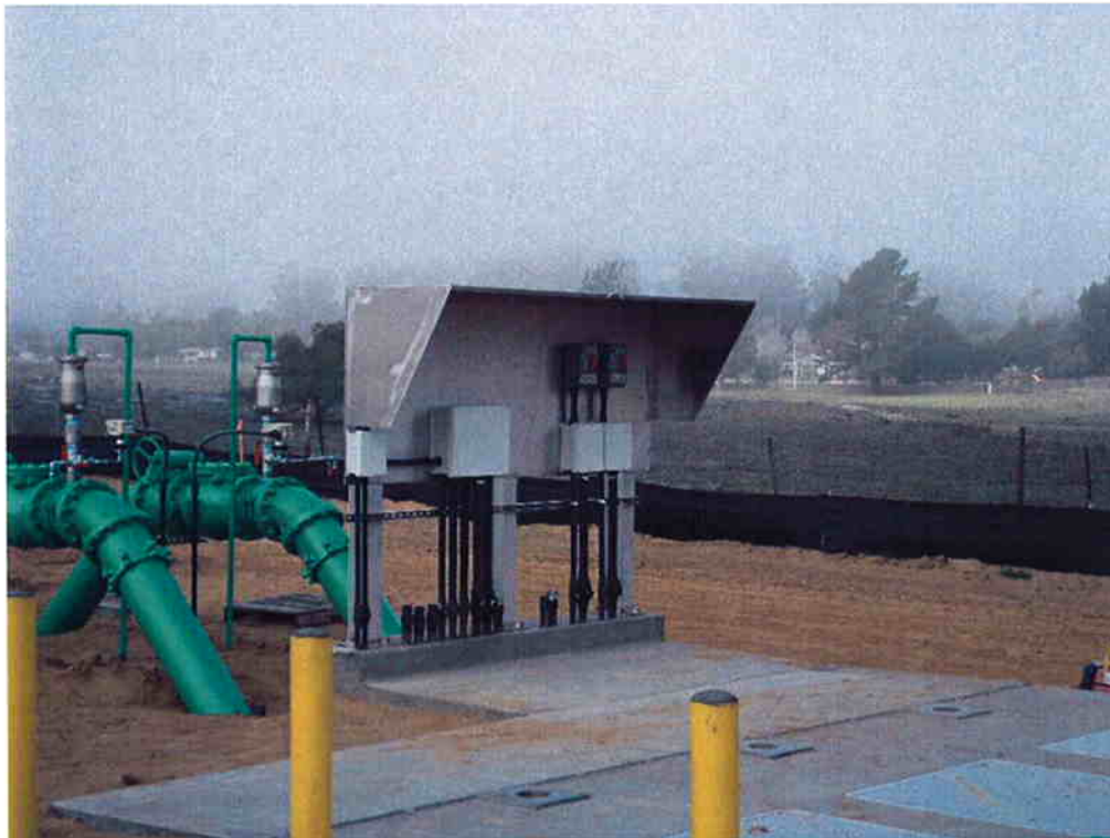
Sunshield installed at Influent Pump Station control panel.
