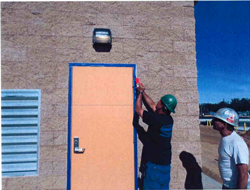
Cushman sealing doors.
