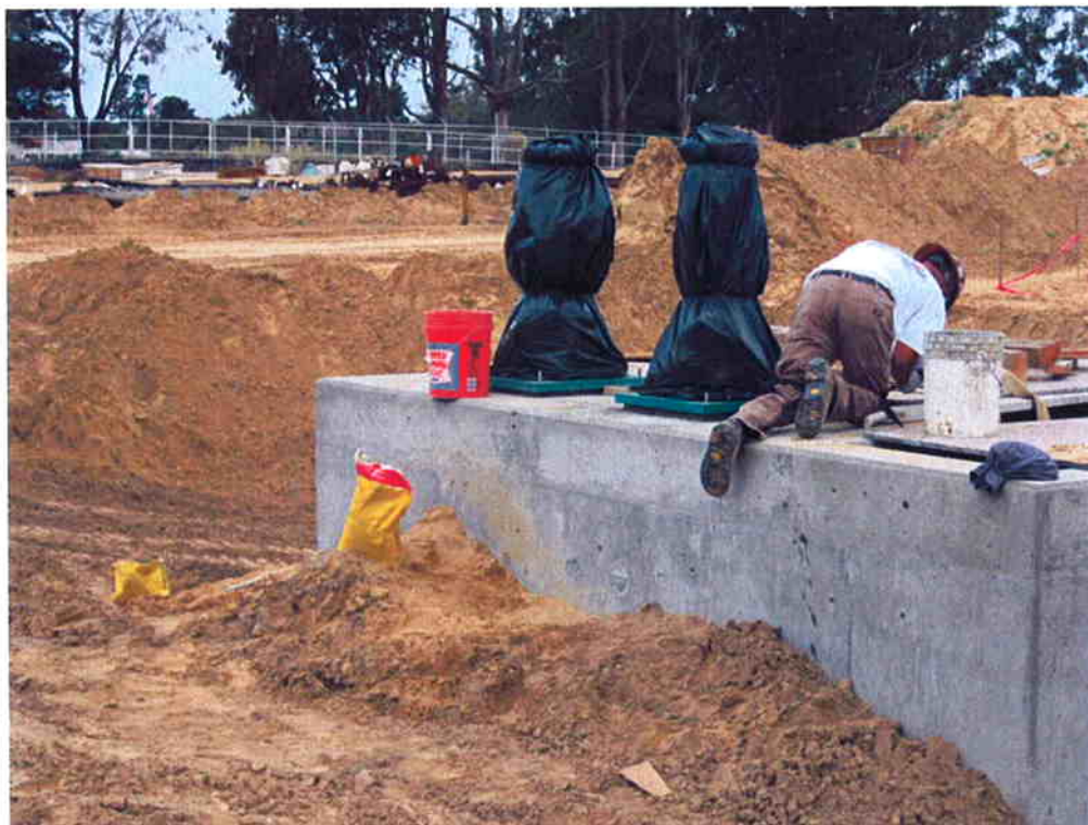
Cushman dry packing the mounting plates for the vertical turbine pumps at the Process Water Pump Station.
