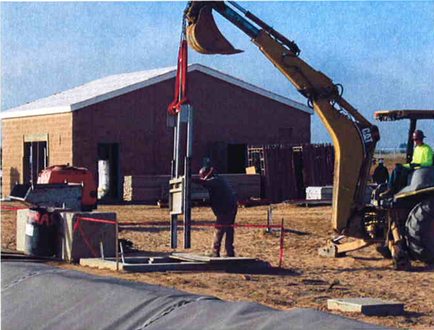
Cushman installing the weir gate at the Weir Box for Aeration Basin #1.
