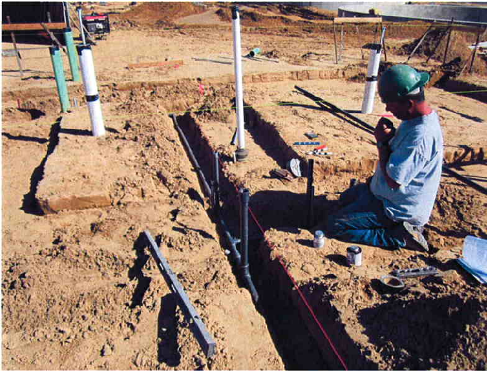
Cushman installing the under slab plumbing for the Sodium Hypochlorite Storage building.
