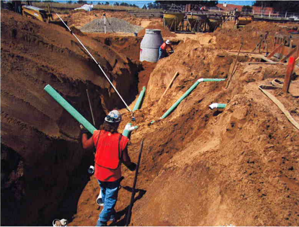
Cushman installing the 6" DR piping from Manhole #7 and connecting to the Sodium Hypochlorite Storage building drains.
