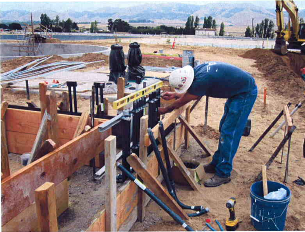
Bergelectric installing conduit through the footings of the Sodium Hypochlorite Storage building.
