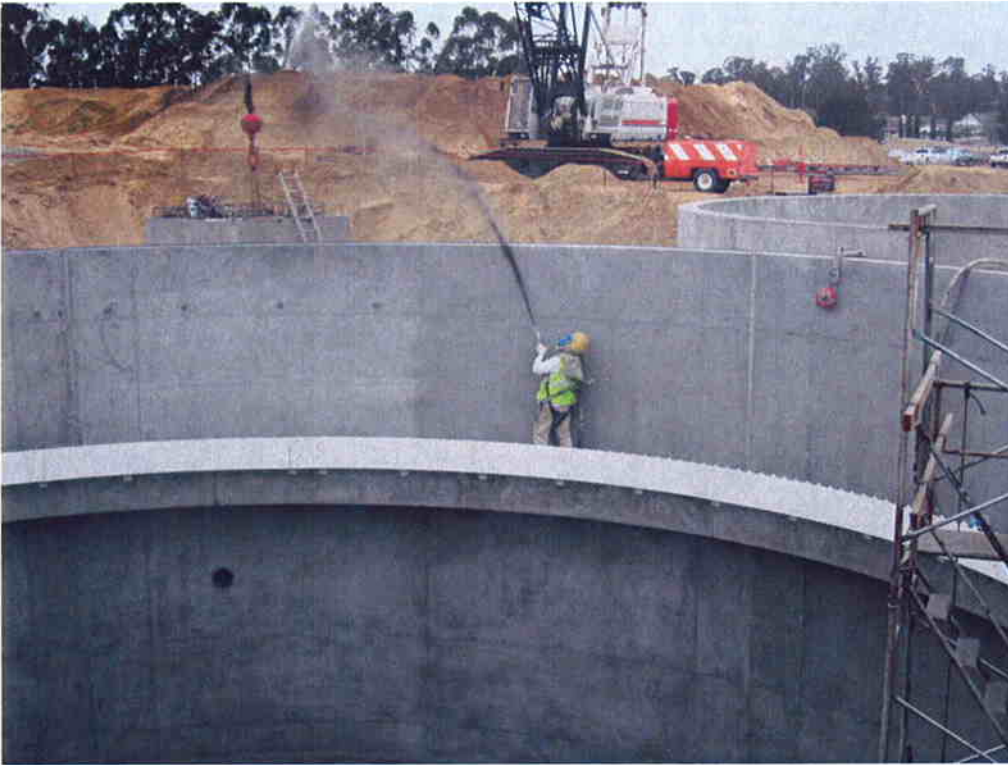
KNK Coating sandblasting the inside of Clarifier #1 in preparation for applying the Xypex coating.
