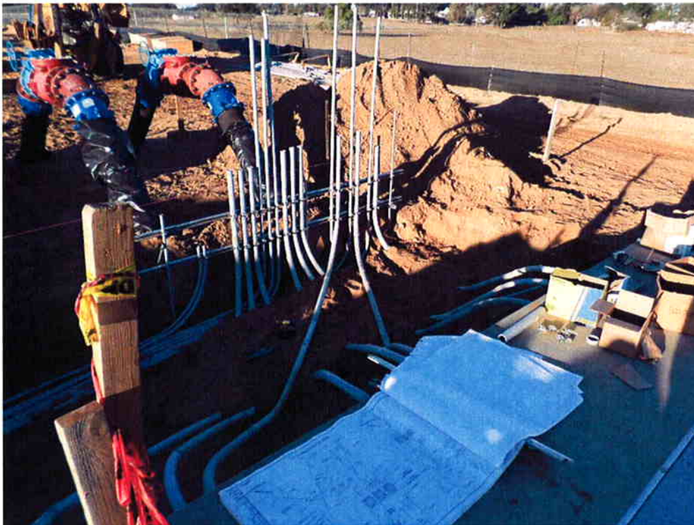
Bergelectric installing under slab conduits to the control panel for the Influent Pump Station.
