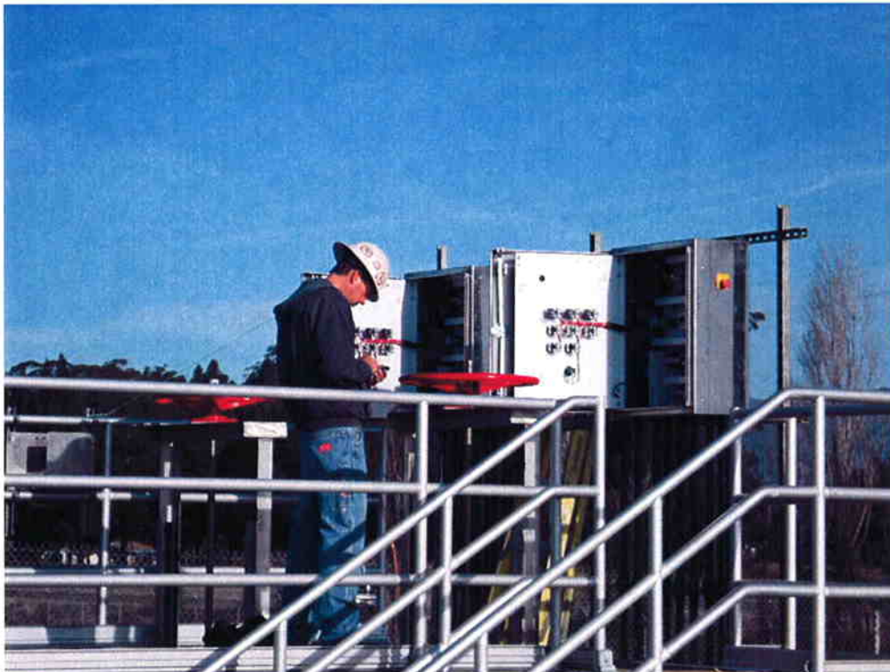
Bergelectric terminating wires at the Headworks control panel.
