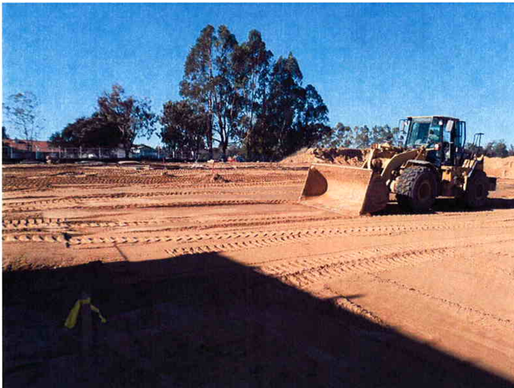
Cushman grading the future road to the west of the Electrical/Blower Building.
