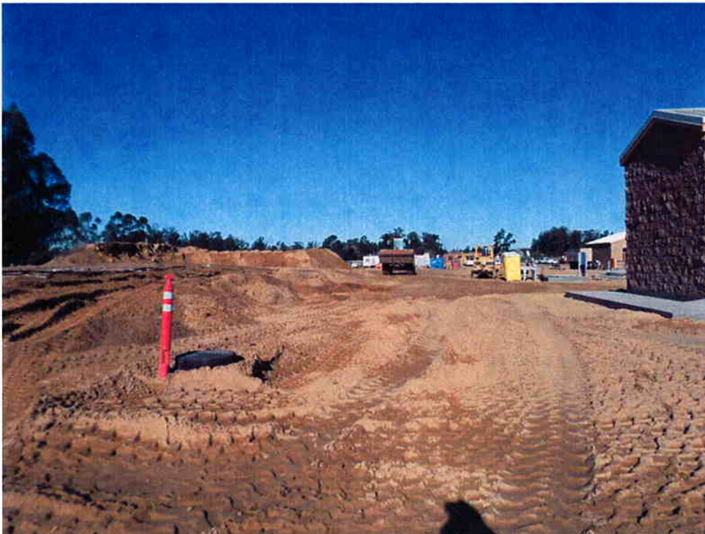
Cushman performing site grading work to the west of the Electrical/Blower Building and Sodium Hypochlorite Storage Building.
