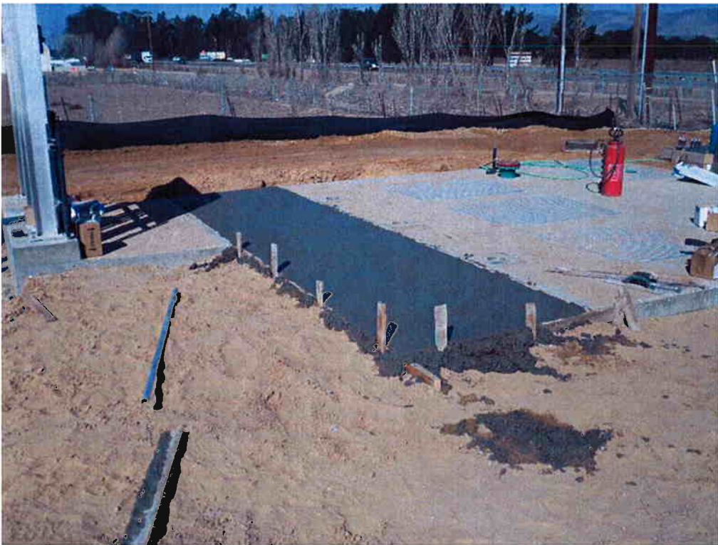
Cushman pouring sidewalk section between Influent Pump Station and the control panel pad.
