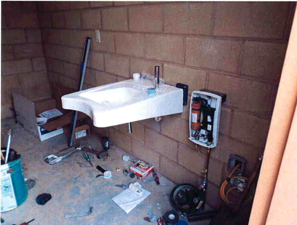
Cushman installing the sink and water heater in the bathroom at the Sodium Hypochlorite Storage Building.
