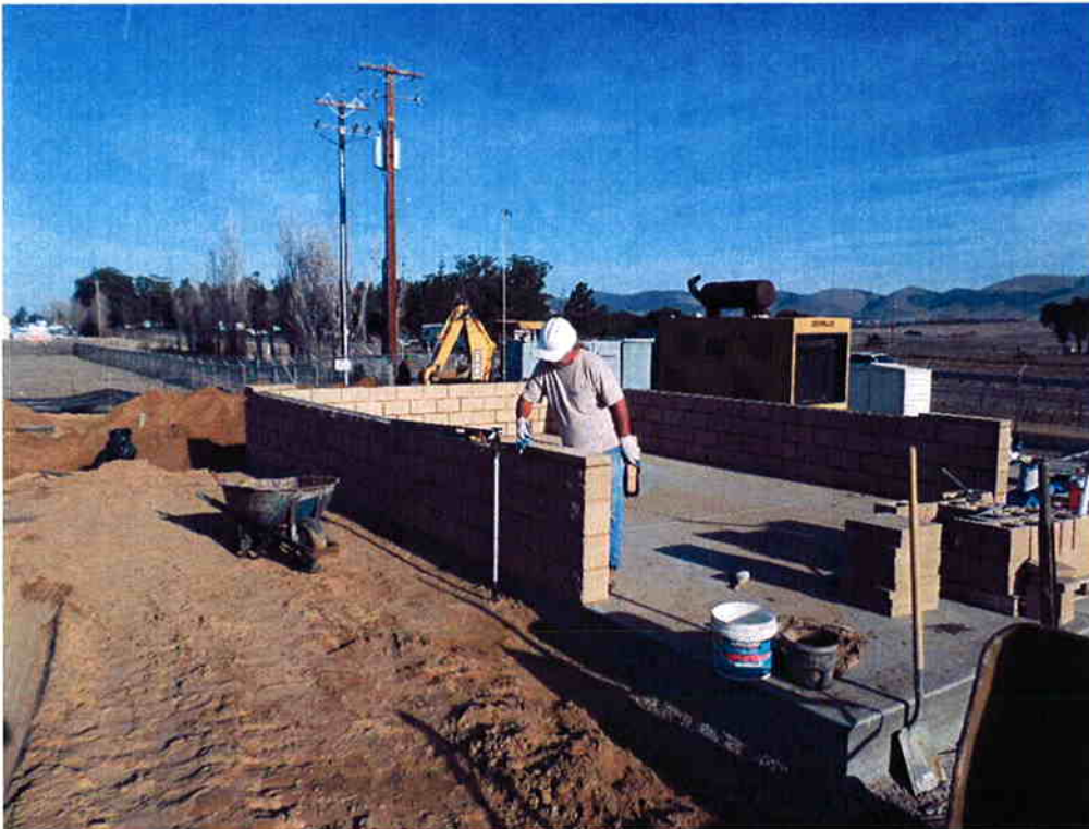
Bienscroth Masonry grouting and installing wall caps at truck wash down station.
