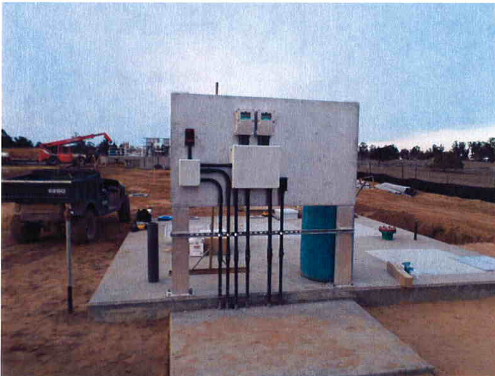
Pull boxes, level transmitters and disconnect switches installed at the control panel rack at the Influent Pump Station.
