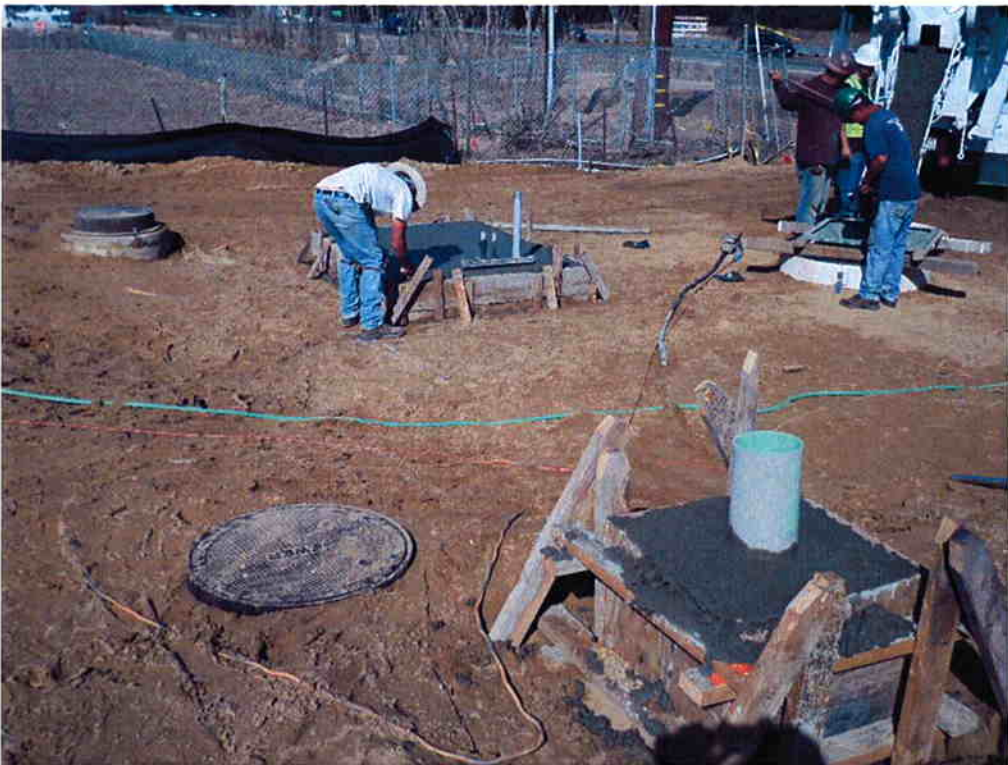
Cushman pouring valve operator pad and sampler pad.
