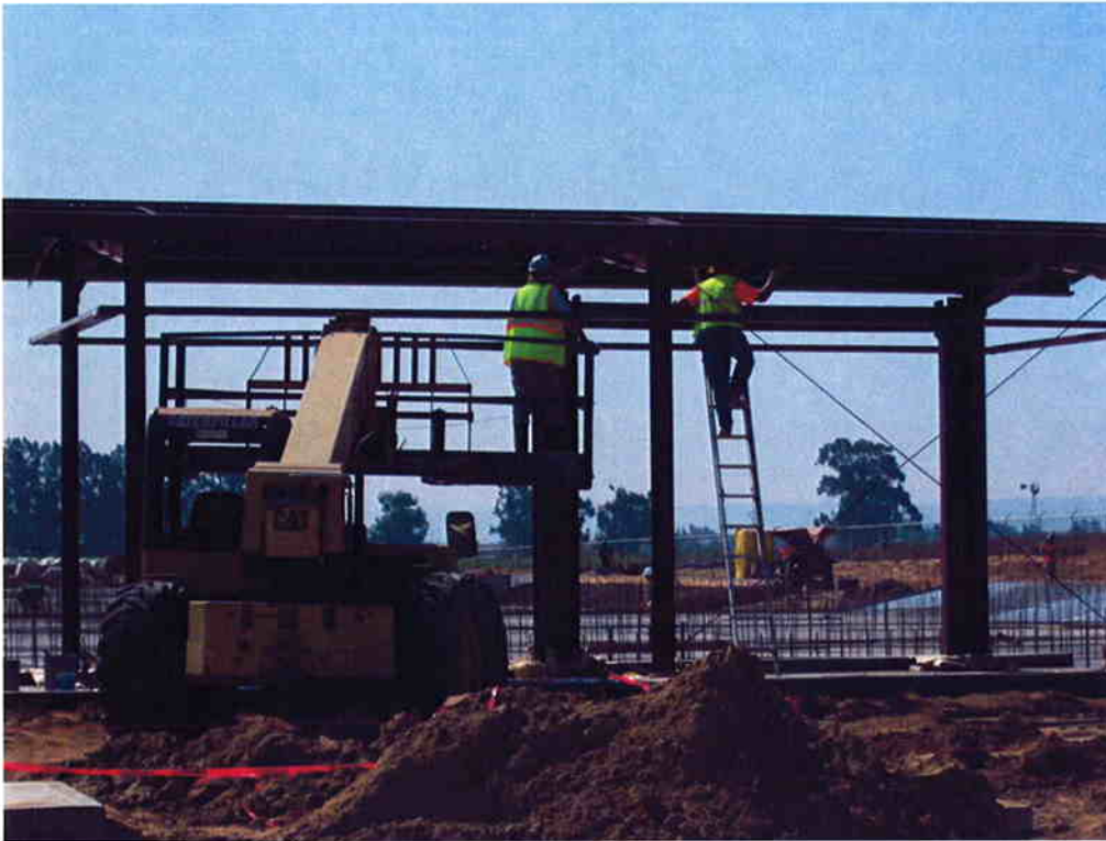
KNK Coating sanding the Sludge Thickening Building in preparation for applying the prime coat.
