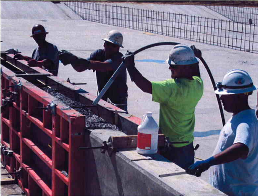
Cushman vibrating concrete during pour of divider walls at the Sludge Drying Beds.
