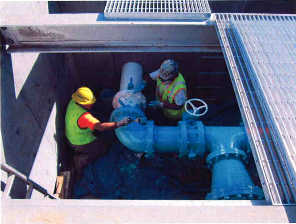
KNK Coating painting AR piping inside the Air Meter and Flow Control Valve Vault.
