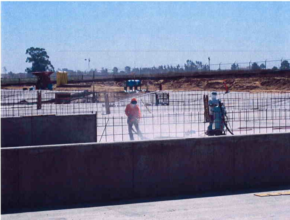
Cushman sandblasting rebar and concrete before next divider wall pour at Sludge Drying Beds.
