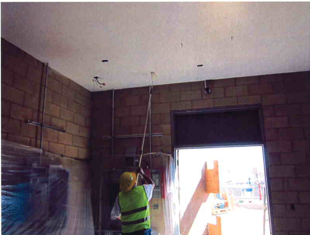
KNK Coating prime coating the ceiling inside the MCC Room of the Electrical/Blower Building.
