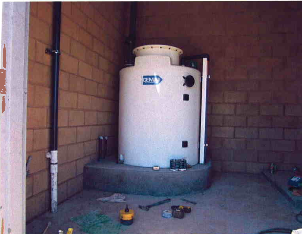
The 300 gallon sodium hypochlorite storage tank installed.
