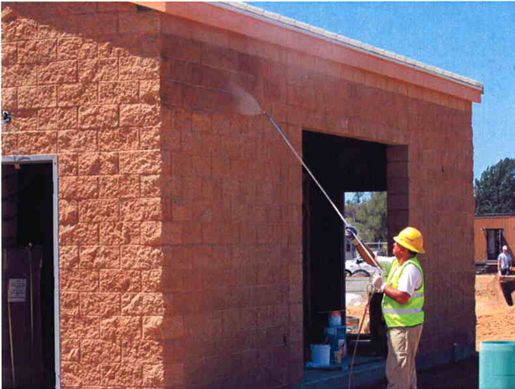
KNK Coating applying Bloc Seal to the outside of the Electrical/Blower Building for waterproofing.
