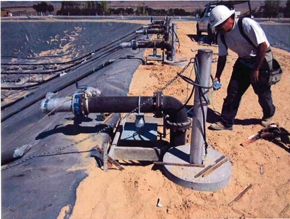
Cushman forming pads for pipe supports and disconnect switches at the AR piping for the Aeration Basin.
