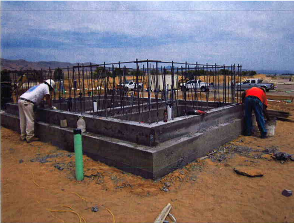
Cushman stripping forms from the concrete starter wall of the Sodium Hypochlorite Building.
