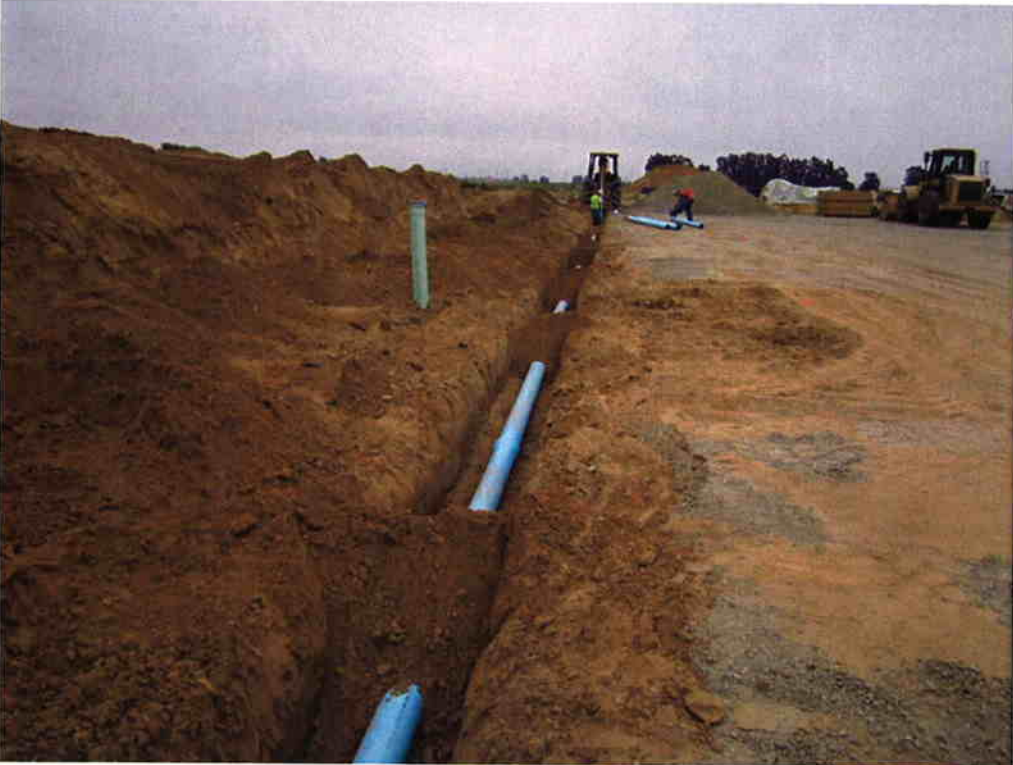
Cushman installing the 6-inch NPW along the east side of the Sludge Drying Beds.
