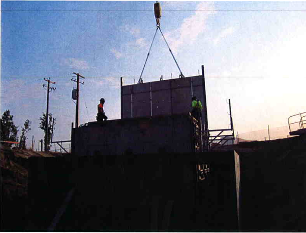
Stripping the forms at the Influent Pump Station after the wall pour.
