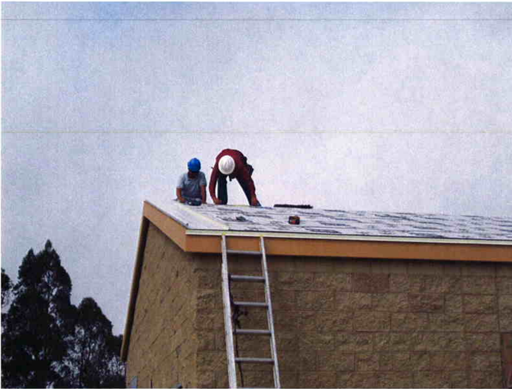
Dueck Roofing installing the standing metal roof on the Sodium Hypochlorite Building.
