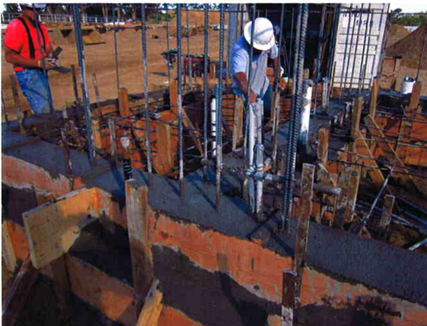
Cushman pouring concrete for the starter wall at the Sodium Hypochlorite Building.
