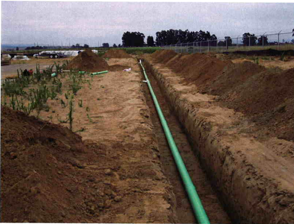
Cushman installing the 6-inch DR piping to the west of the Sludge Drying Beds.
