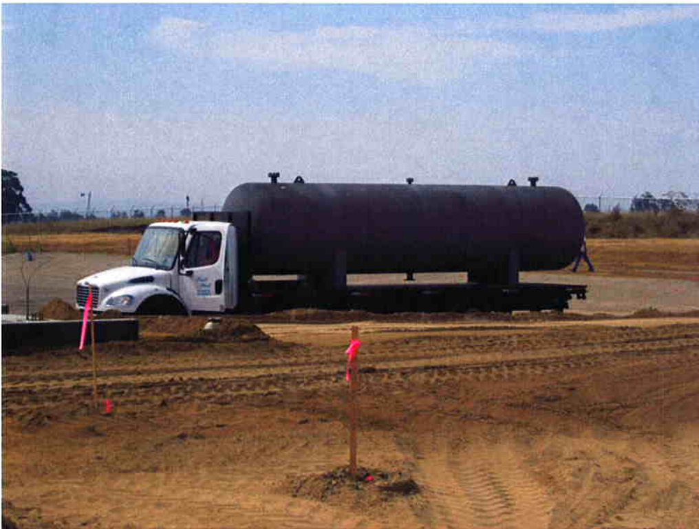
Receiving the hydropneumatic tank.
