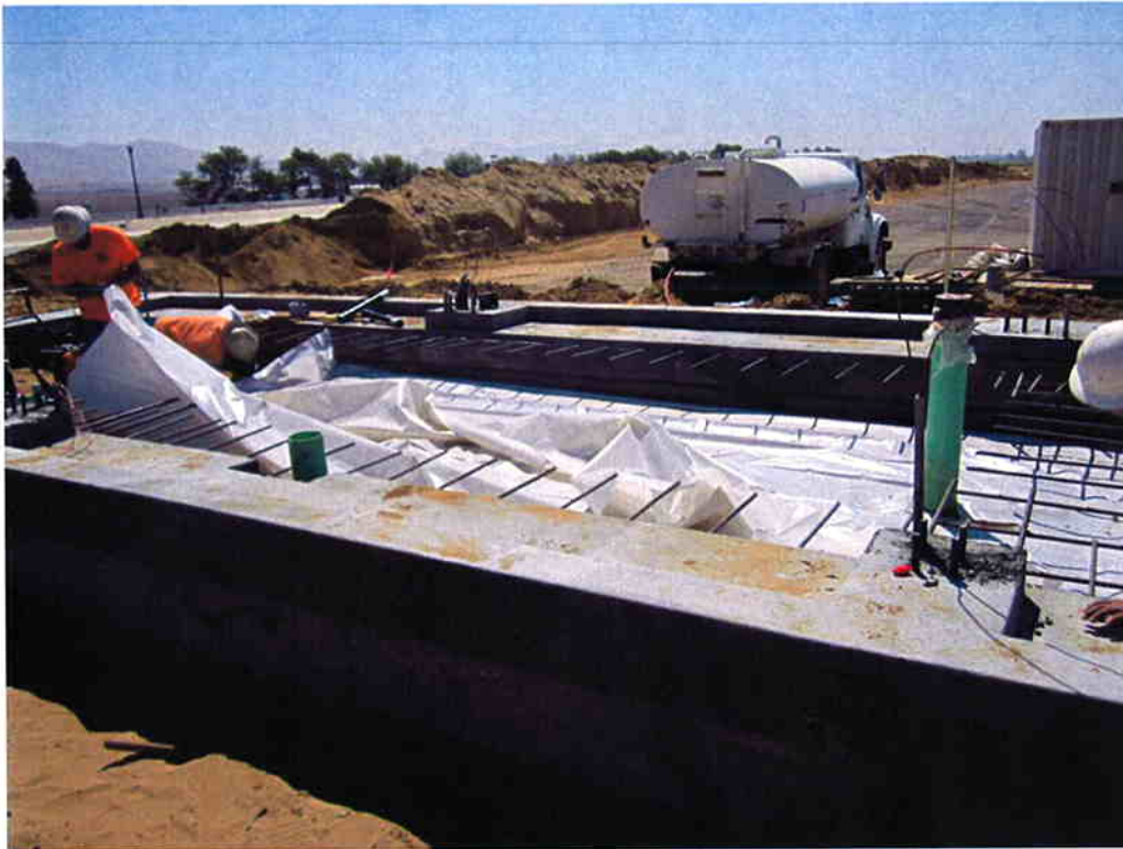
Installing the vapor barrier under the slab for the Sludge Thickening System.
