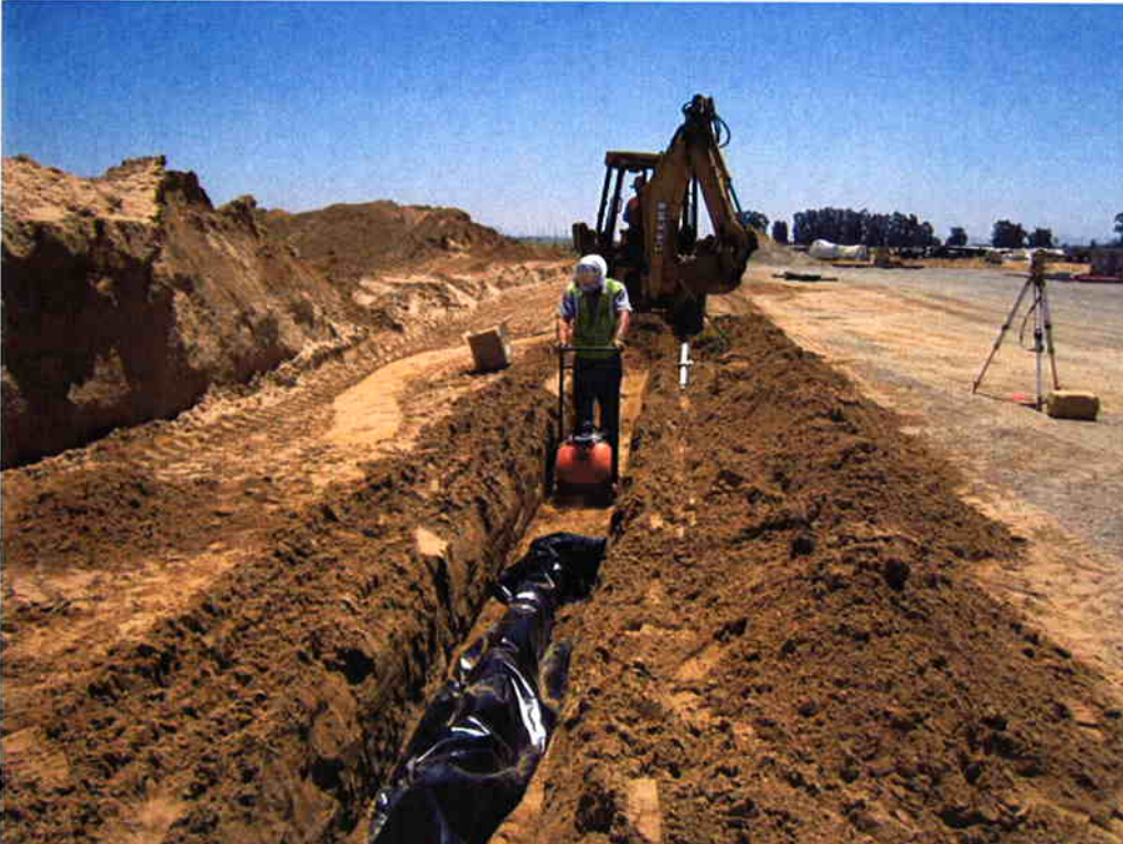
Cushman installing the 6-inch TWAS to the east of the Sludge Drying Beds.
