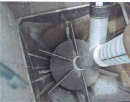
DynaSand Filter modules in concrete basin
