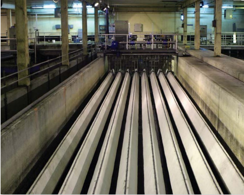
Overview of AquaDiamond® filter retrofitted into a 16' wide sand filter cell.
