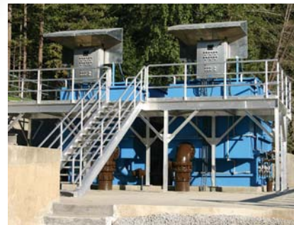
Two AquaDisk® Filters with walkway access.
