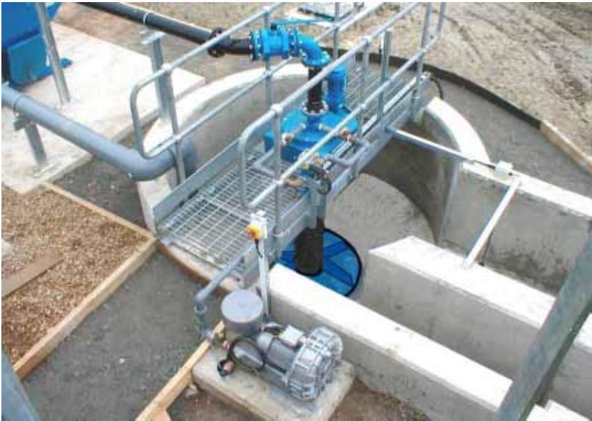
The completed Jetair installation.
