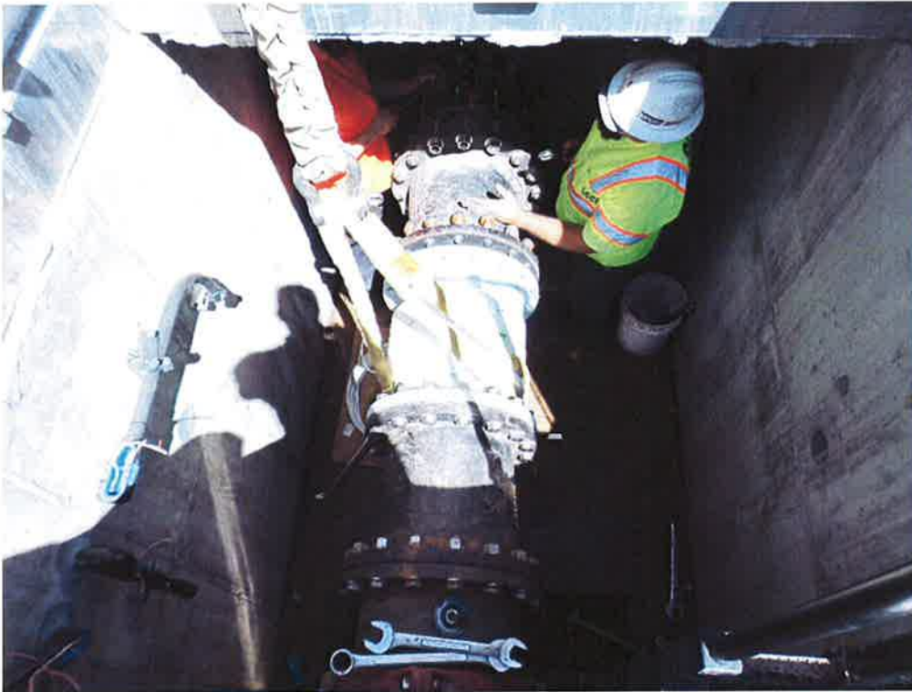
Flow meter installed in flow metering vault.
