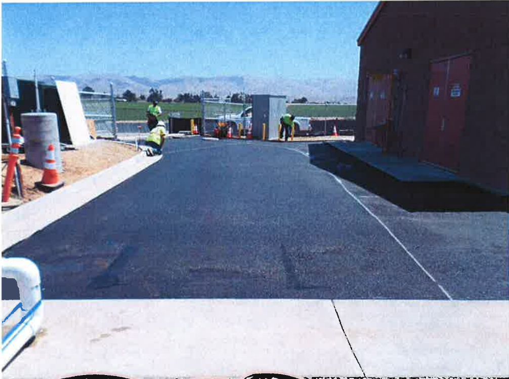
Toste Grading and Paving laying out drainage swale for pump station driveway.
