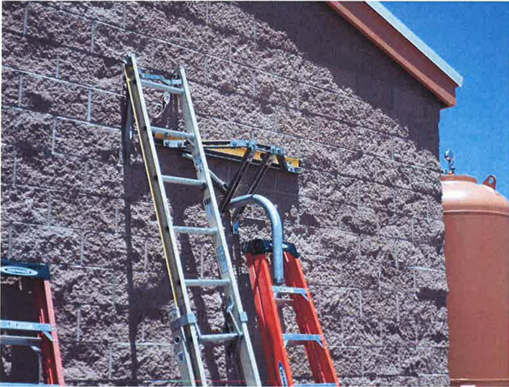
St. Denis Electric setting up support brackets to mount SCADA antenna to the building.
