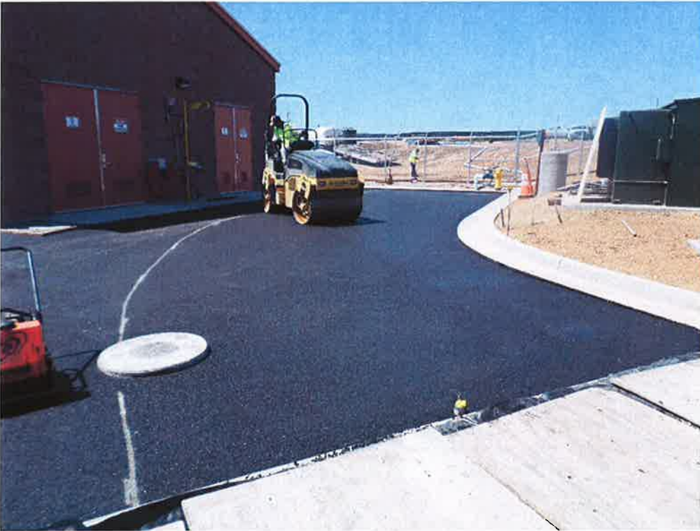
Toste Grading and Paving rolling first lift of asphalt for pump station driveway.
