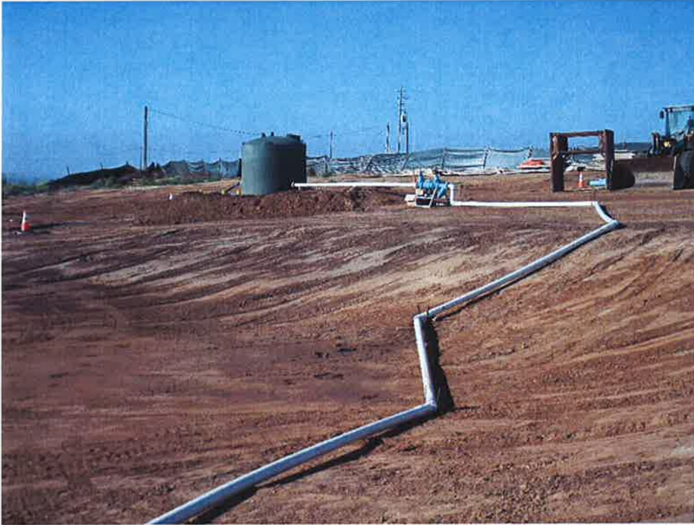
Temporary tank and piping installed in preparation for testing the pump station prior to taking water from the City of Santa Maria.
