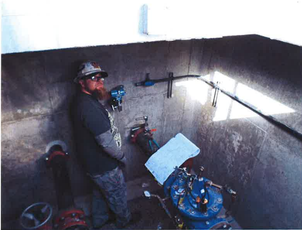
St. Denis Electric installing the pressure transmitter and conduit in the PRV vault.
