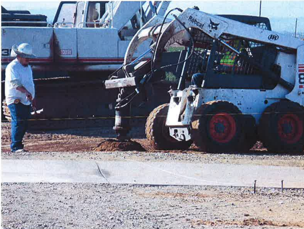
Central Coast Fencing augering fence post holes at the pump station site.
