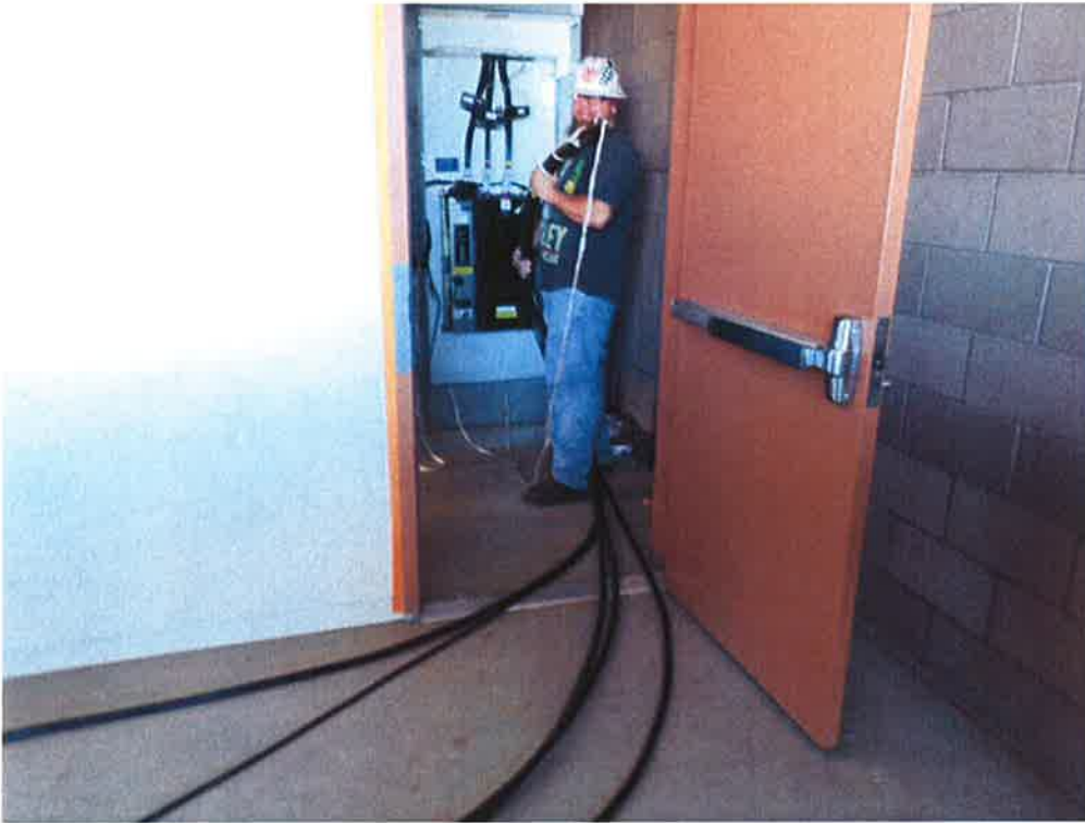
St. Denis Electric pulling wire at the ATS in the electrical room.
