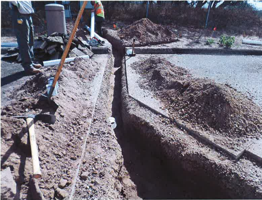
Spiess excavating trench for the 4-inch drain line and conduit at the Standpipe Tank.
