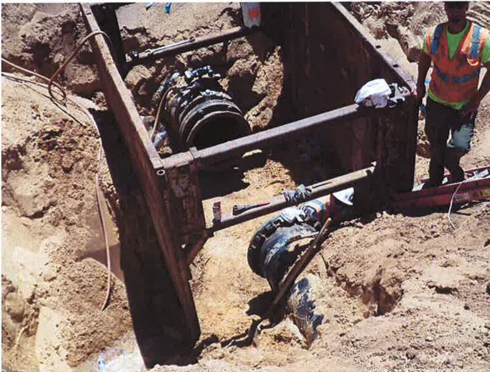
Spies preparing to connect the 24-inch DIP pipe from the pump station to the HDPE pipe from Bid Package #1.
