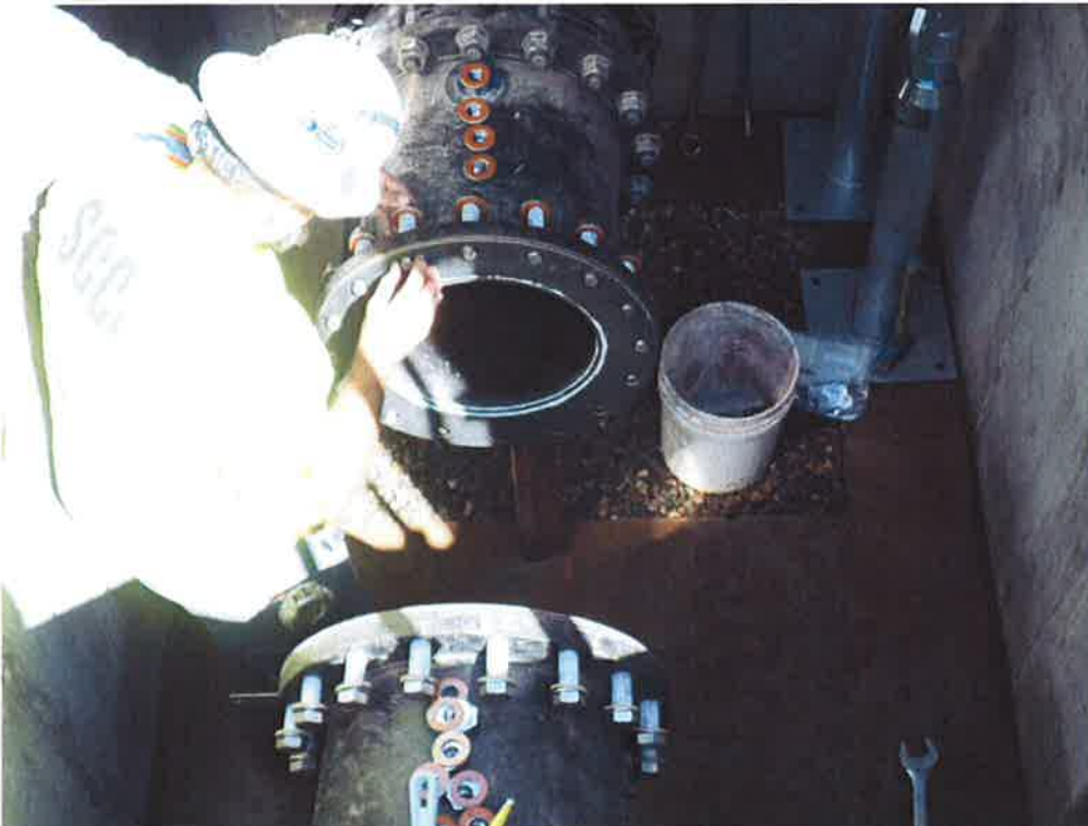
Spiess installing the flow meter in the flow meter vault at the pump station.
