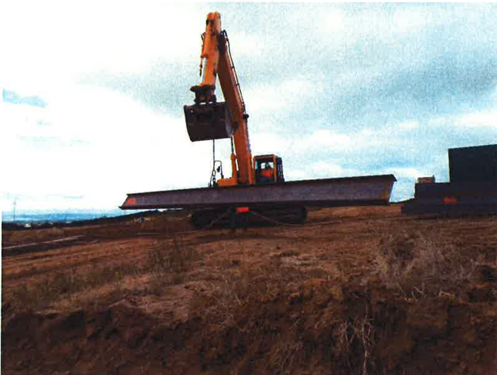
Moving I-beam for placing into drilled hole and backfilling with concrete and slurry.
