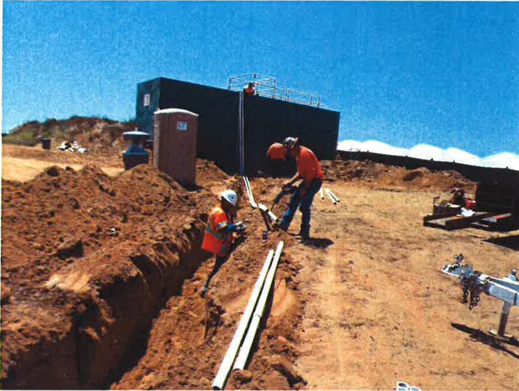
Curtis Drilling mobilizing Baker tank and installing trenching for drilling mud application to prevent failure of the pile holes during drilling.
