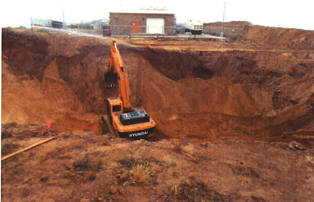
PHC compacting bank in reservoir excavation to help prevent material failure during drilling of pile holes.
