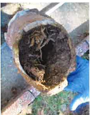
Sewer main destroyed by roots
