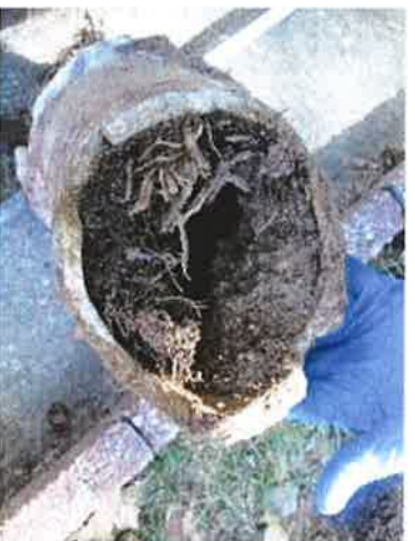
Sewer main destroyed by roots
