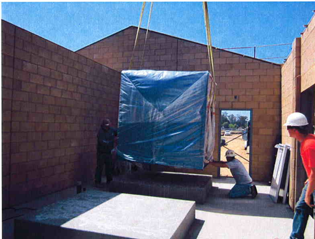
Cushman and Bergelectric setting blowers on equipment pads before installing the roof.
