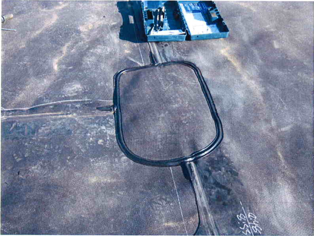
Patch made with extrusion weld at destructive double fusion weld test location.
