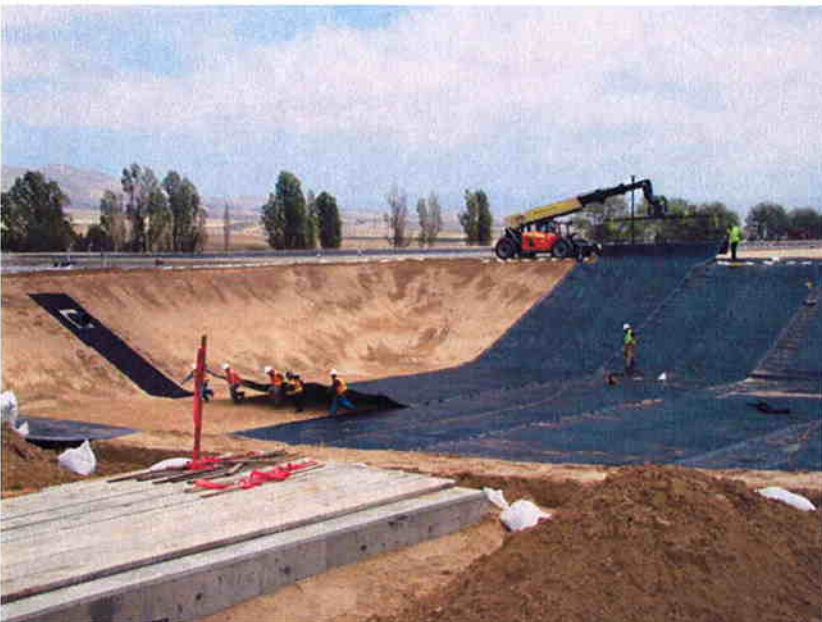
Subcontractor Barber-Webb pulling the liner sheets into place across the Emergency Holding Basin.
