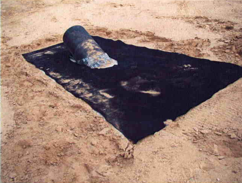
Felt pad installed over concrete at inlet pipe to protect liner from rubbing and wear.
