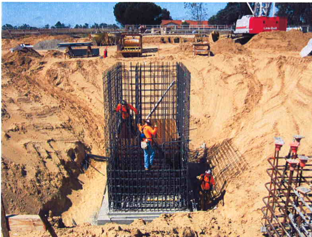
Subcontractor, CMC Rebar installing rebar for walls of Processed Water Pump Station.
