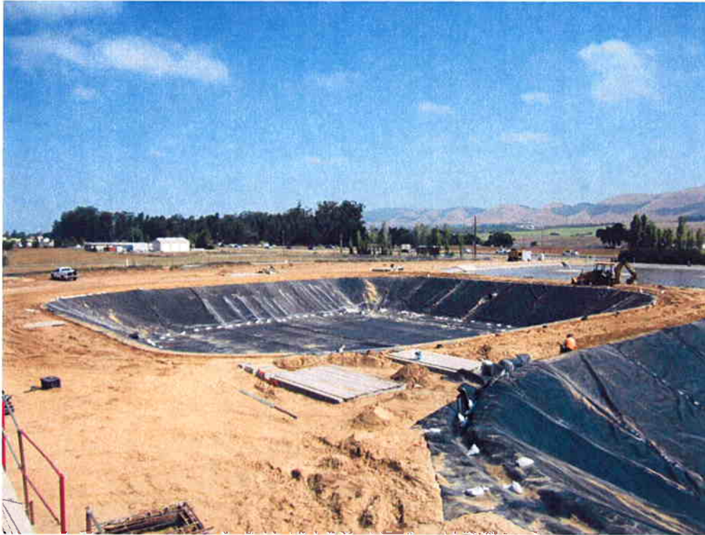
Lining installation completed in Aeration Basin #1 and Cushman compacting lining anchor with backhoe.
