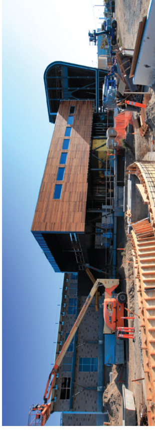
Advanced Water Purification Facility (AWPF)
